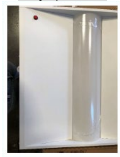
Emergency Test Button
