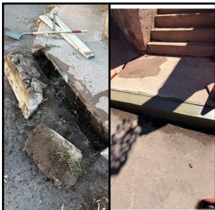
A resident reported a dangerous sidewalk; repairs were quickly made.
