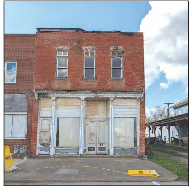
The building at 137 North Bridge Street is cordoned off due to safety hazards. The property has been approved for demolition with assistance from the Ashland County Land Bank. Photo by Amanda Chambers
