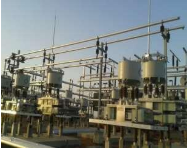
SVC view of filter area Installation
