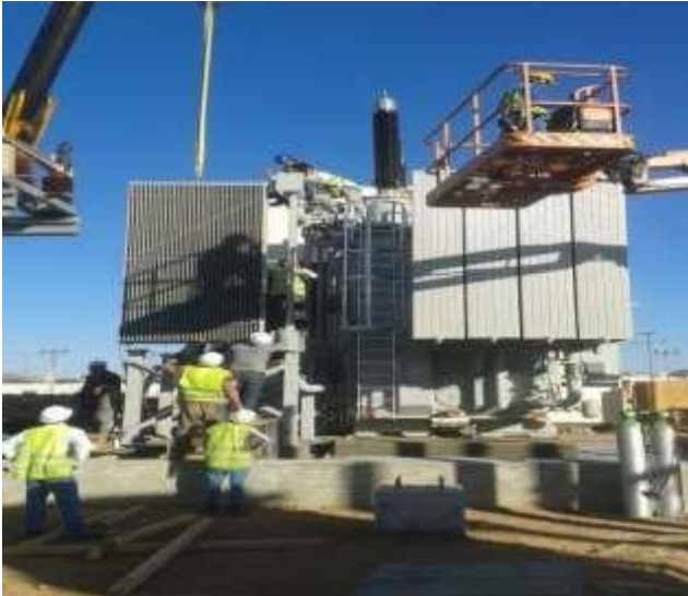
Power Transformers Assembly
