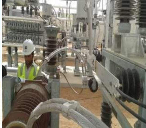
Internal Aluminum cable connections at
