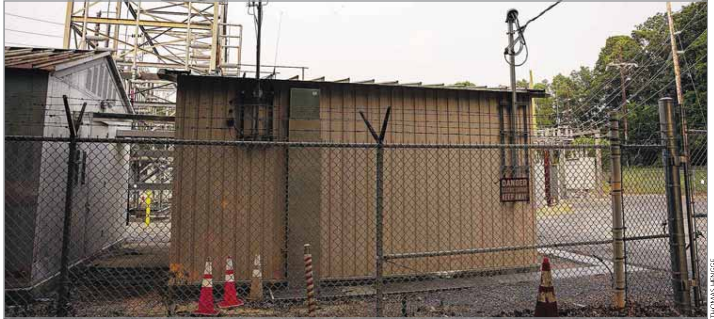
A lithium-ion battery storage facility in East Hampton. Tests of some nearby wells show high levels of forever chemicals from a toxic plume.
