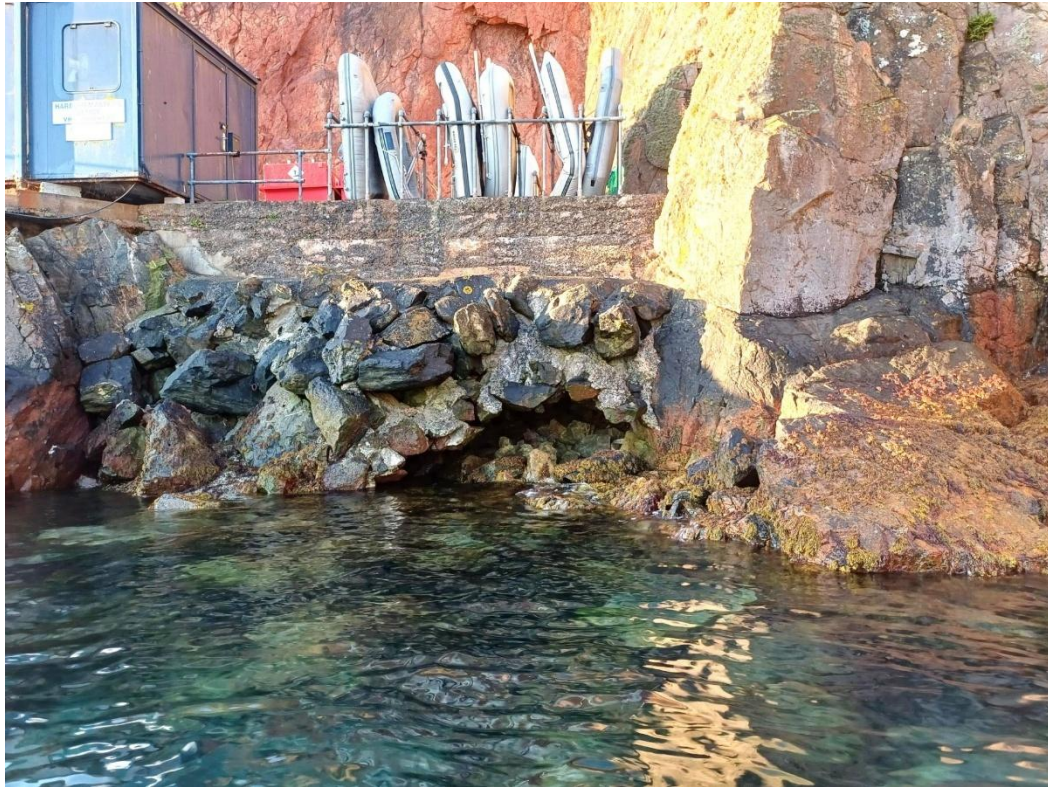
Undermining of the Maseline Harbour Quayside
