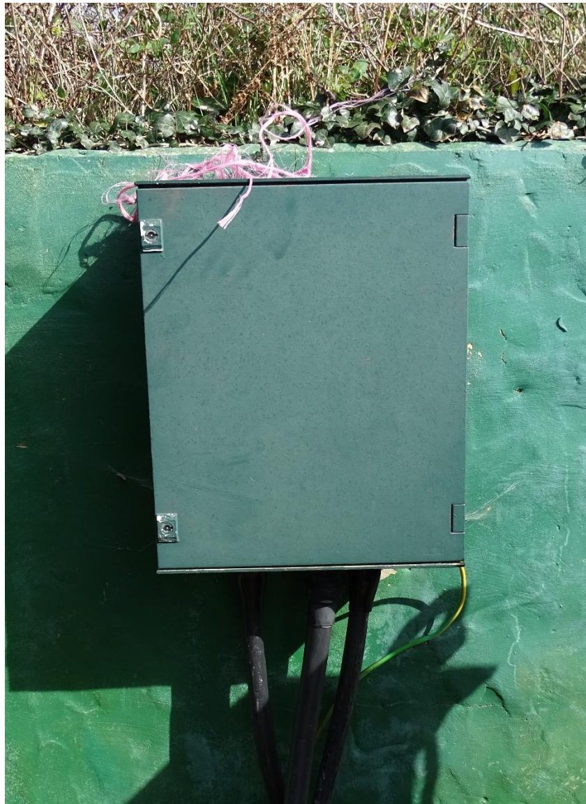
Figure 7: Typical substation LV cabinet
