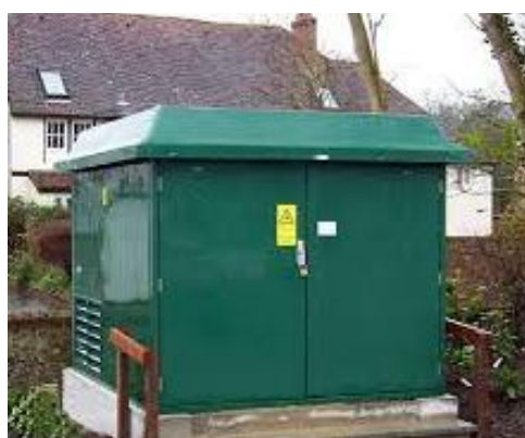
Figure 11: GRP substation enclosure
