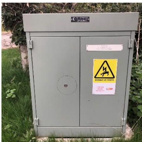
Figure 10: Free standing pad mount substation
