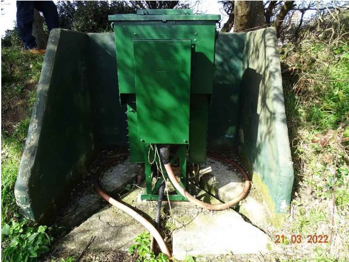
Figure 6: Typical high voltage ring main unit operating space & trip hazards
