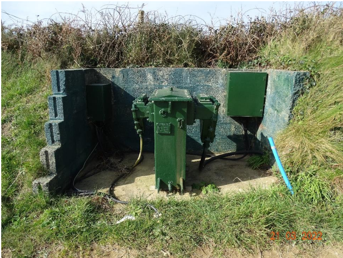
Figure 5: Typical transformer and low voltage cabinet installation
