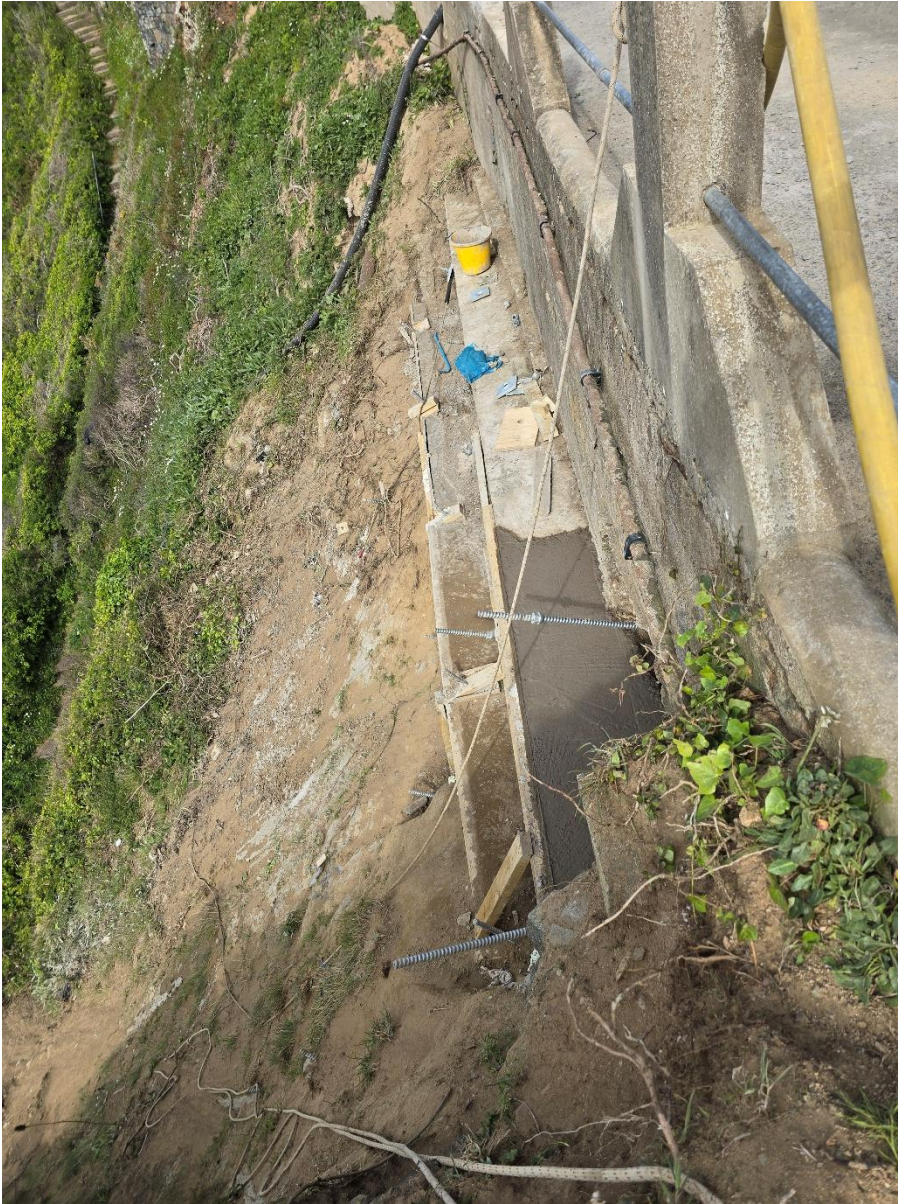
Detail of former with concrete setting inside shuttering former at area W2
