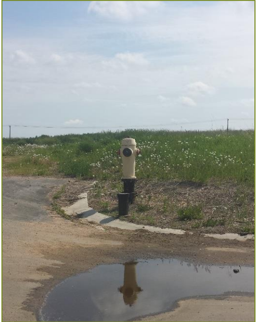
Figure 16. Fire hydrant within Boyle
