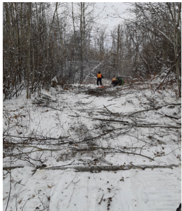
Vegetation cleanup during development south of Maintenance Access near KM 17 on Canfor Road
