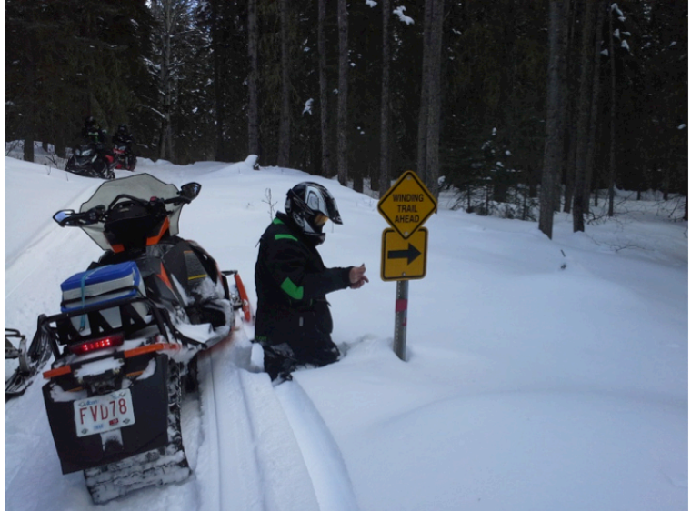
Installing reflector tape on a sign post near the west end, March 2018
