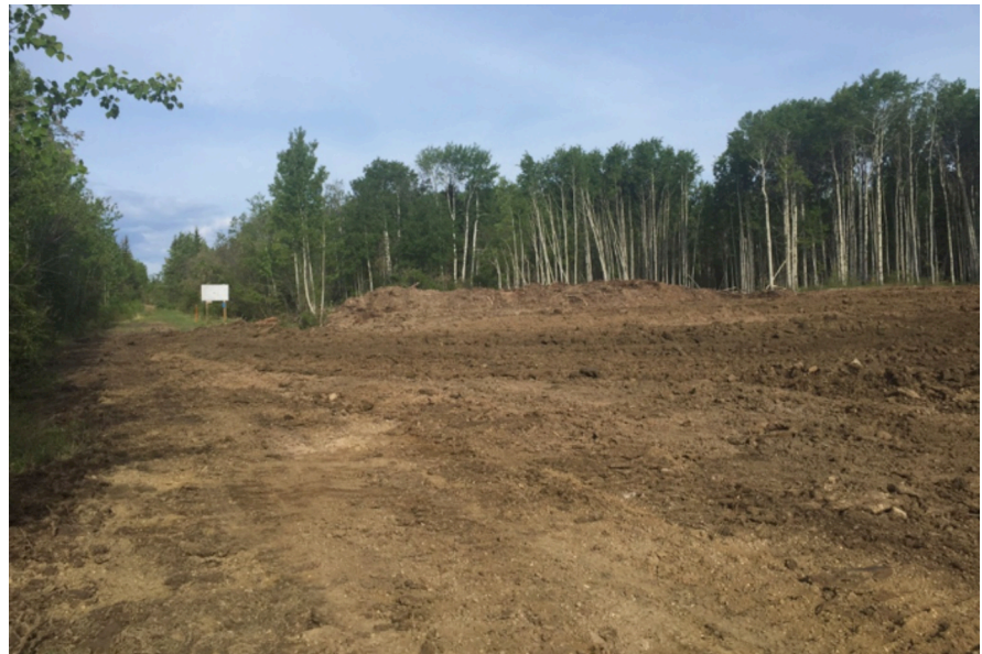
East End Staging Area under construction just prior to the May 2016 snow on long weekend
