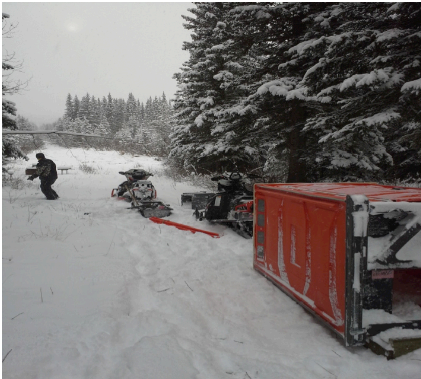
The Club's first outhouse arrives at the rest area for installation, November 5, 2017
