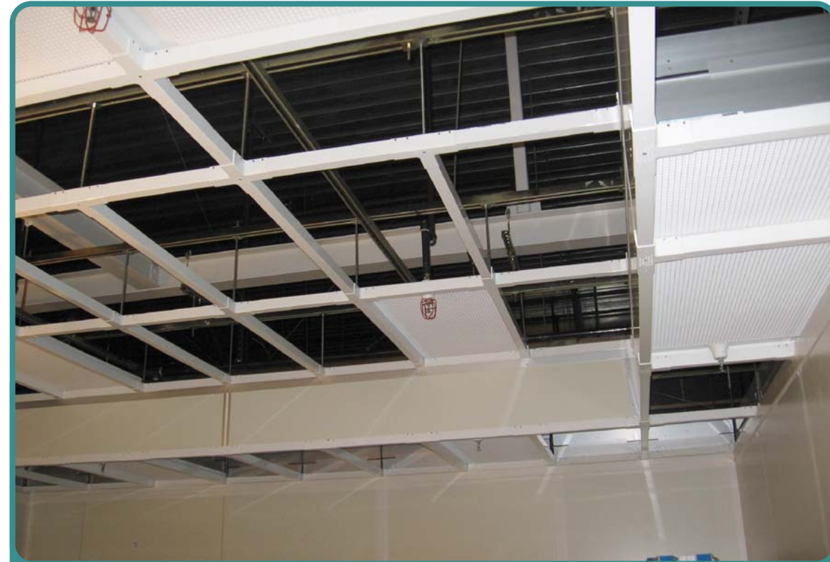
Figure 1. Raised Section of the HEPA Support Structure Inside the Solid Construction Barrier
