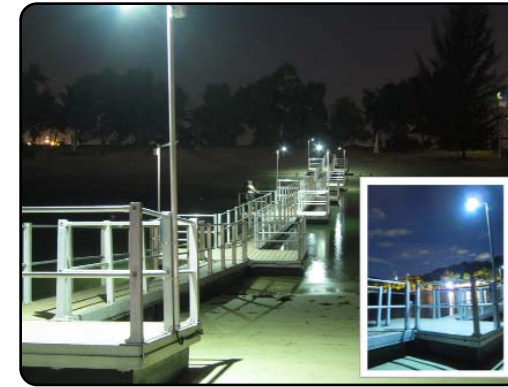
Figure 3 – Luna Eyes Illuminating a Floating Bridge With no AC Supply
