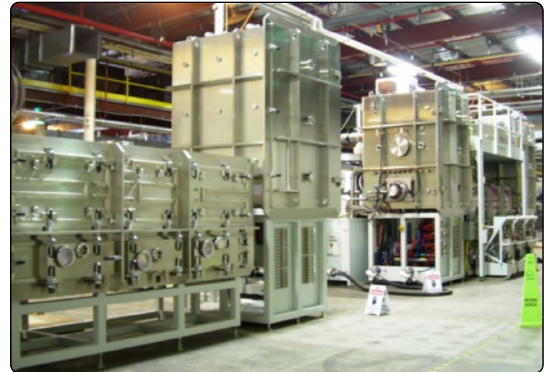
Figure 4 – Large-scale CIGS Deposition Tool Capable of Processing 1 m Wide Web to be Installed at USPVMC Manufacturing Development Facility
