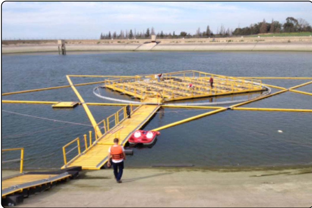
Figure 3 – View of the Installed Floating CPV System
