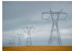
New Transmission Lines
