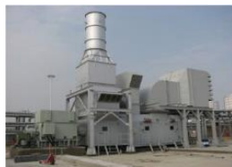
Gas Peaking Plant
