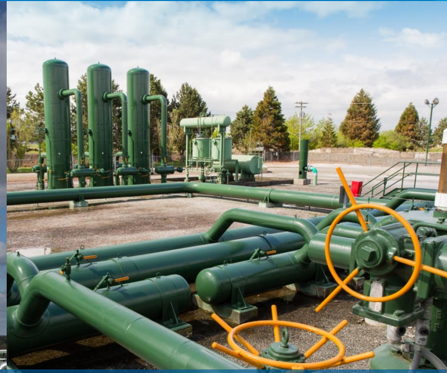
SUMAS COMPRESSOR STATION
