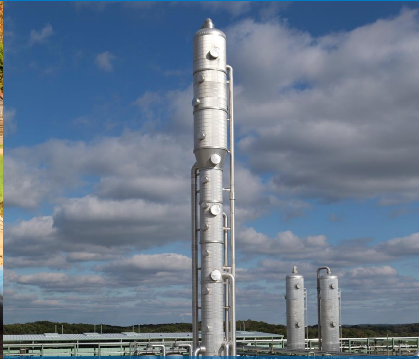
KENSINGTON GAS PROCESSING PLANT
