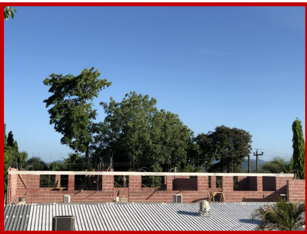
Construction has been halted temporarily. We hope to finish by graduation day (December 2, 2019).
