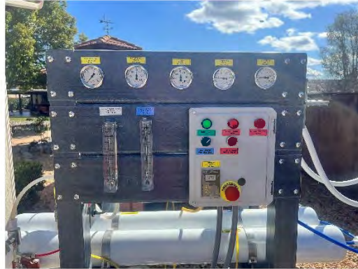
4.6.1.2 High Pressure Pump Concentrate Pressure Reading
