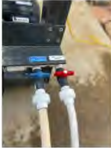
5.5.1.1 Fresh water and Sea water Inlet Valves Off
