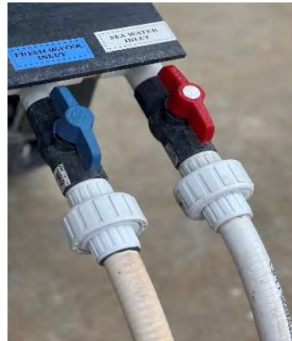
5.1.1.1 Fresh Water and Seawater Valves On
