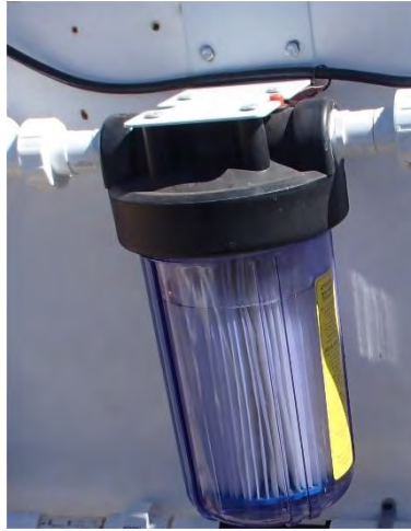
10.6.1.1 UV – Aeration 20 Micron Filter
