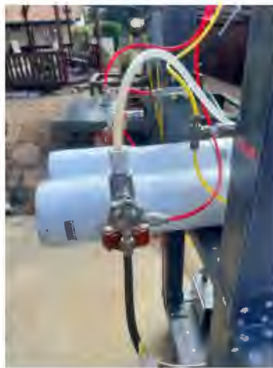
4.6.1.1 Inlet Vessel Pressure Control Valve
