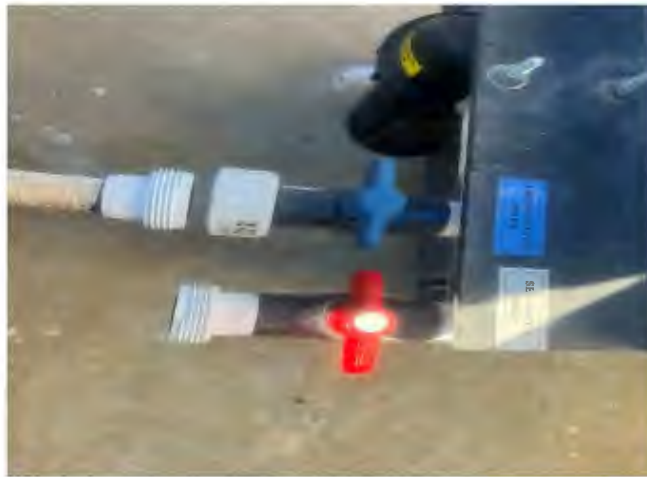
2.1.1.1 Fresh Water Connection Photo
