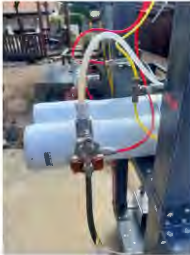
5.6.1.1 Inlet Vessel Pressure Control Valve
