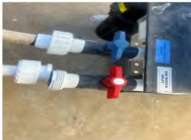
2.2.1.1 Brackish Water Connection Photo
