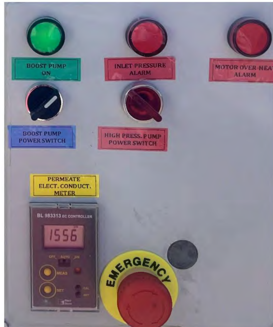
8.1.1.1 GVA-4000 Electric Panel External View
