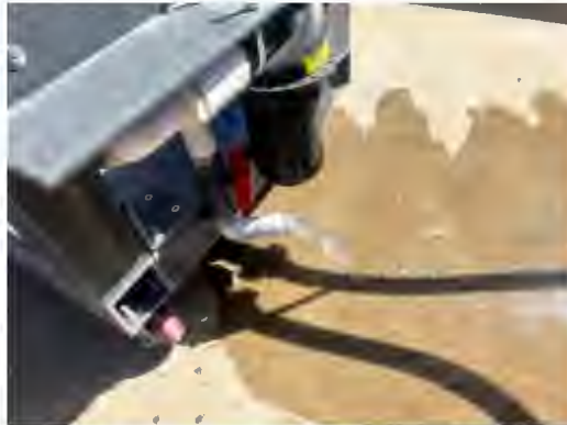
4.5.1.1 Inlet Water Purge Valve
