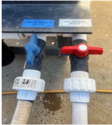
4.3.1.1 Fresh Water Inlet Valve On Photo
