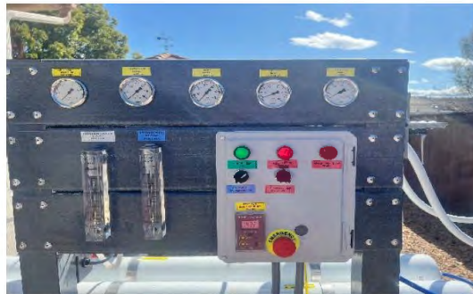
4.4.1.1 Pre-Filter Inlet Pressure Gauge Low Reading
