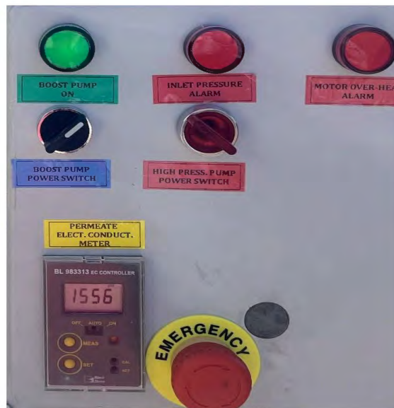
6.4.1.1 GVA-4000 Emergency Shutdown Switch
