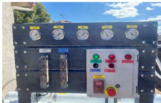
4.4.1.2 Pre-Filter Inlet Pressure Gauge Operational Reading
