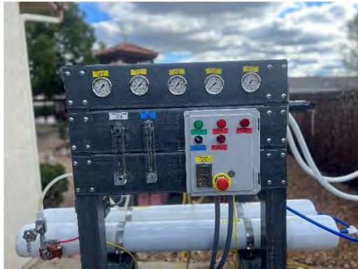
5.4.1.1 Booster Pump Power Switch Off
