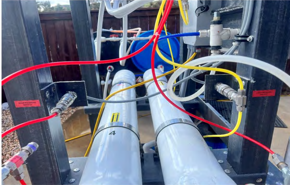
6.1.1.1 GVA -4000 High and Low Pressure Device Location
