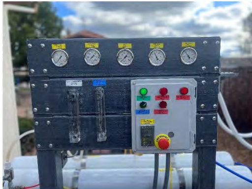
5.3.1.1 High Pressure Pump Power Switch Off
