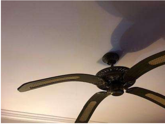
Light Fixture/Fan Existing Damage from Move-in. 📅 2023-08-07 10:59:38 🖼️ Image
