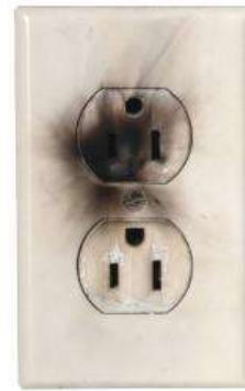
Switch/Outlet Item was damaged when I moved in. 📅 2023-08-07 10:55:41 🖼️ Image
