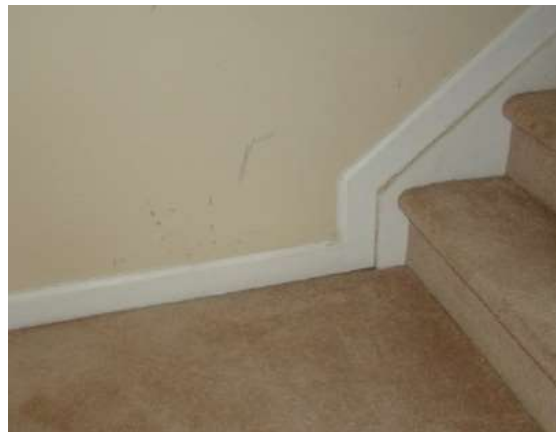
Wall/Ceiling Marking on walls noted as existing damage 📅 2023-08-07 10:58:31 🖼️ Image
