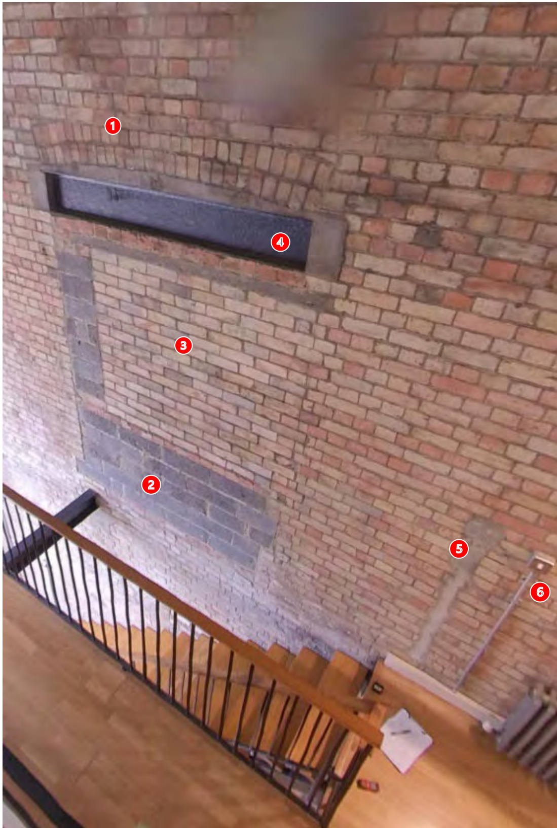
Figure 31: The side wall from the inside (1) the original bricked lintel, (2) the first infill with blocks, made probably before 1975, (3) the second infill made at the time of the conversion in 2001, (4) the steel lintel, made probably in 2001 as well, (5) cement infill to grooves into the wall next to wall mounted switches (6).
