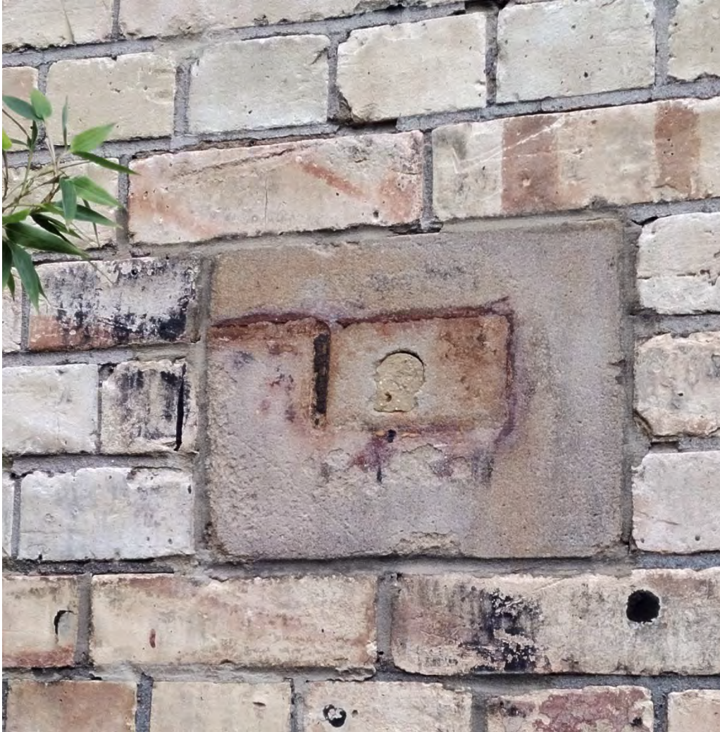
Figure 30 One of the spots where the metal structure of the coal lift was fixed to the wall.
