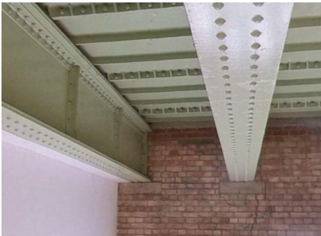
Figure 25: The giant "I" beams supporting the roof and the water tank above it.
