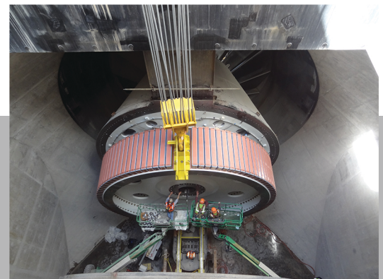
Meldahl Hydroelectric Plant Foster, KY
