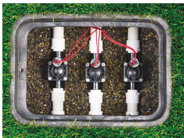
PGV-100G Valve Installed
