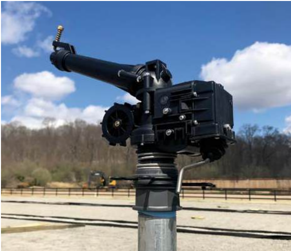
ST-1200-BR Rotor Installed
