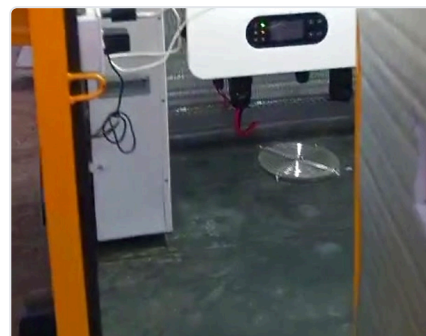
ELECTRICAL ROOM — 6.5 KVA INVERTER
