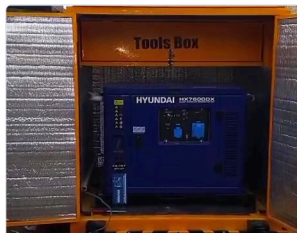
GENERATOR ROOM — 5 KVA GENSET
