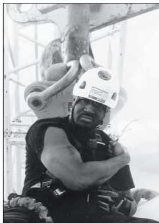
Norman having a little fun after climbing a 320 foot Siemens wind turbine, preparing to hook up the rigging behind him in order to replace a main bearing.
