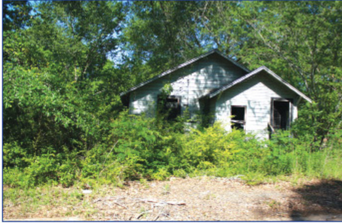
Many families enjoyed this rent house on MLK before it deteriorated
