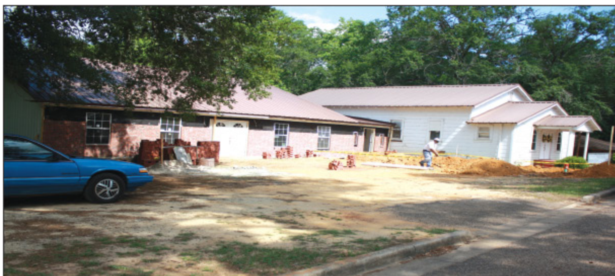
H. R. Waggoner, member, installs safety tape around opening for plumbing installation.
