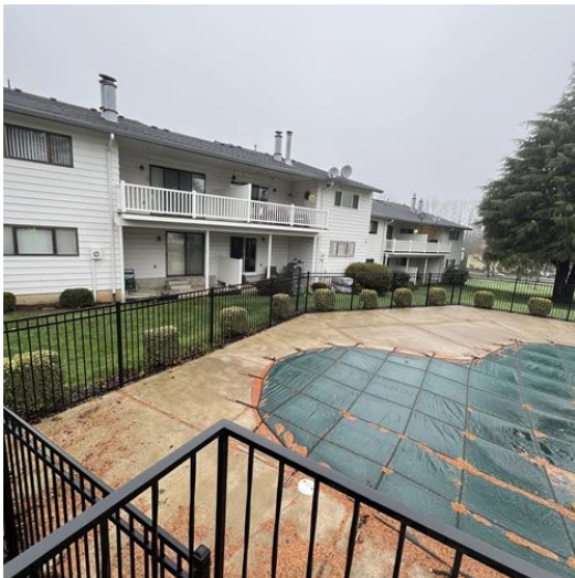
Description: Allowance for repairs to the concrete deck around the pool.
