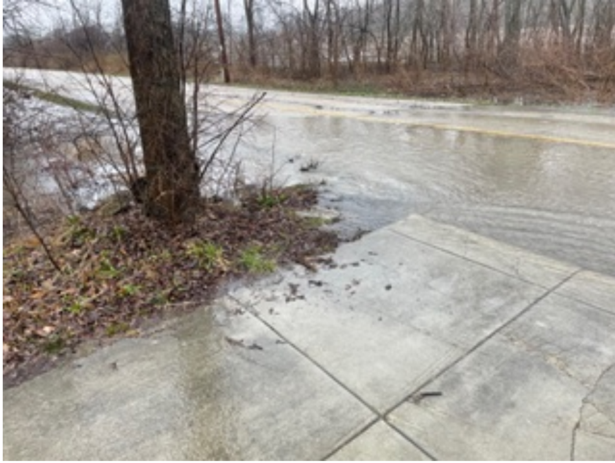
Photo 2: Town Line Road flooding — water flowing across roadway surface and into adjacent ditch, demonstrating insufficient drainage capacity in existing infrastructure.
