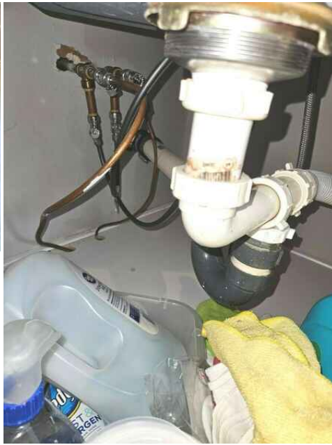
kitchen under sink plumbing
