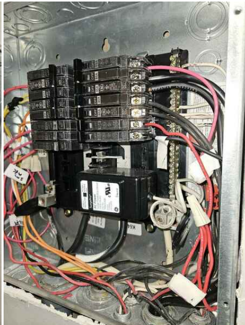
right side breakers
