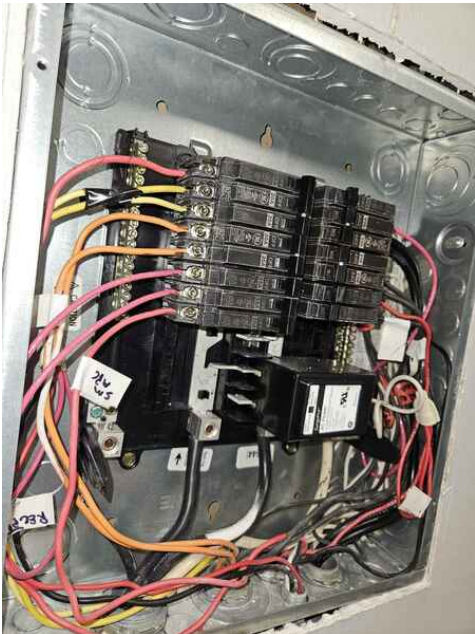
left side breakers
