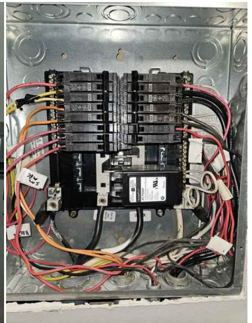
breaker box with cover removed
