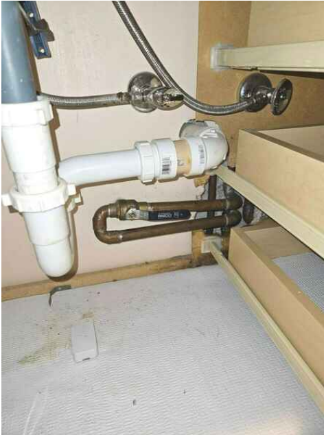
master under sink plumbing
