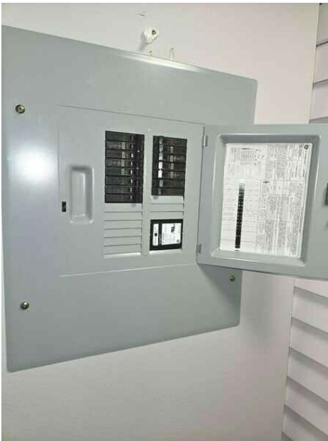
breaker box with cover on
