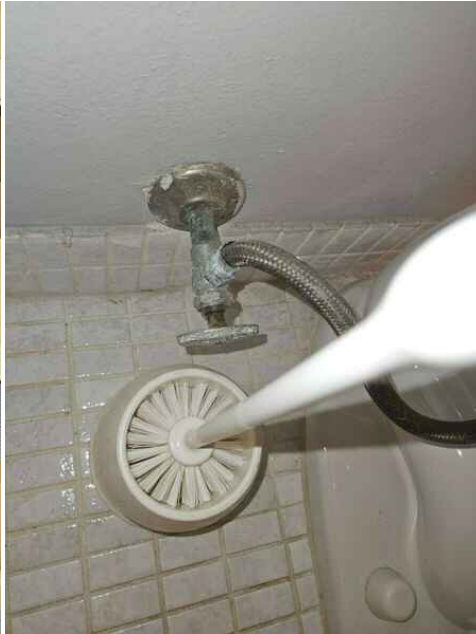
master toilet valve
