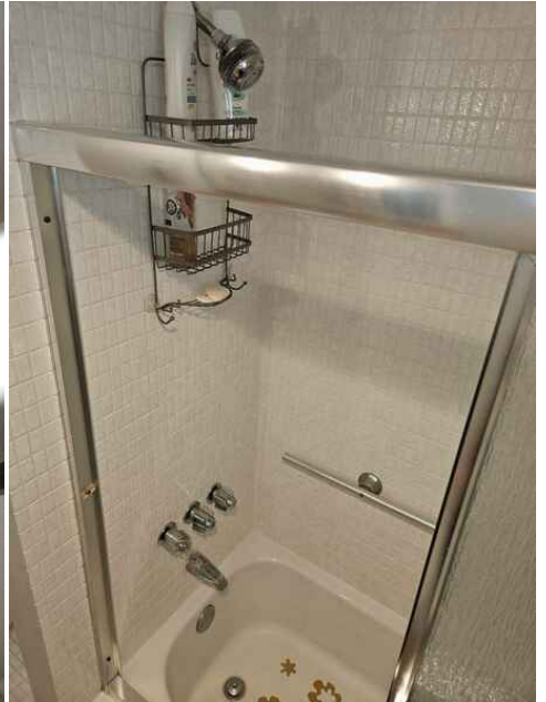
master shower valves and drain
