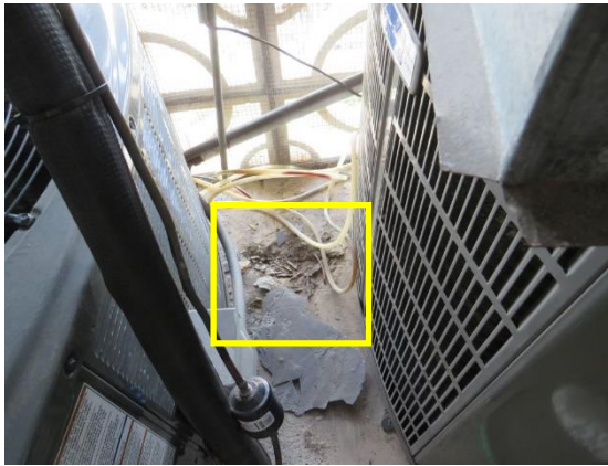
Delaminated Slab Concrete
