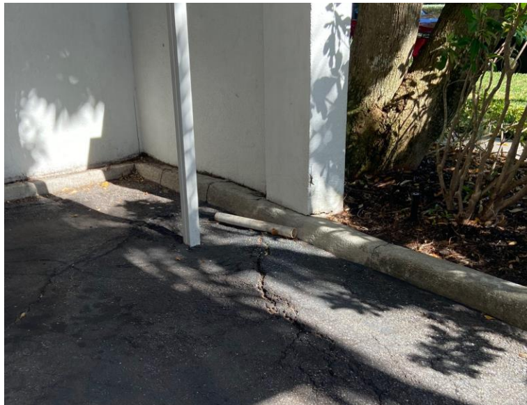
Figure 6: Asphalt cracks potentially caused by tree roots.
