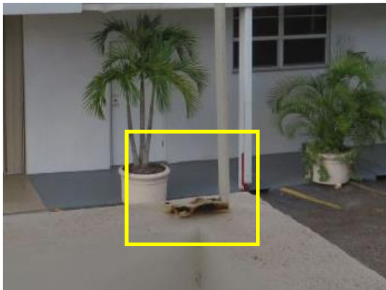
Damaged Steel Canopy Support
