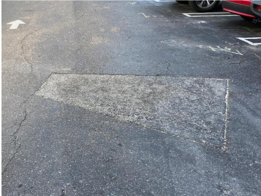
Figure 5: Lot alligator cracking.
