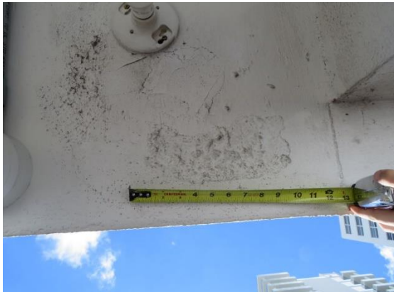
Concrete Spalling at Underside of the Slab
