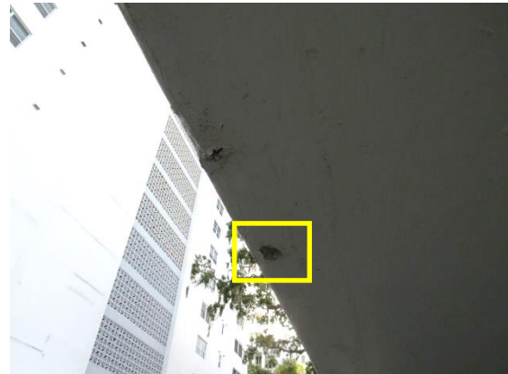
Concrete Spalling at Underside of Slab
