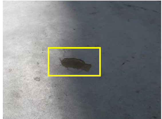
Missing Waterproofing at Parking Slab
