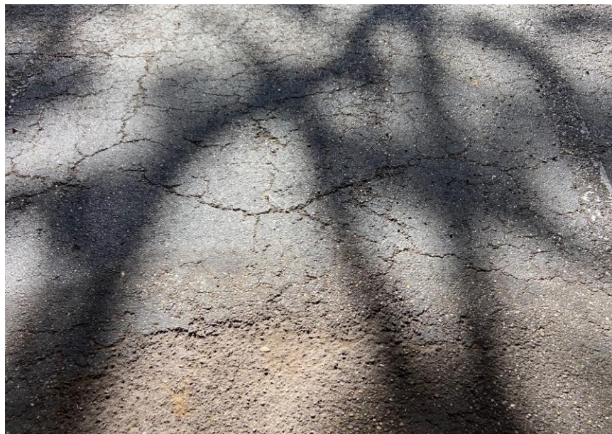
Figure 3: Lot shrinkage cracks.
