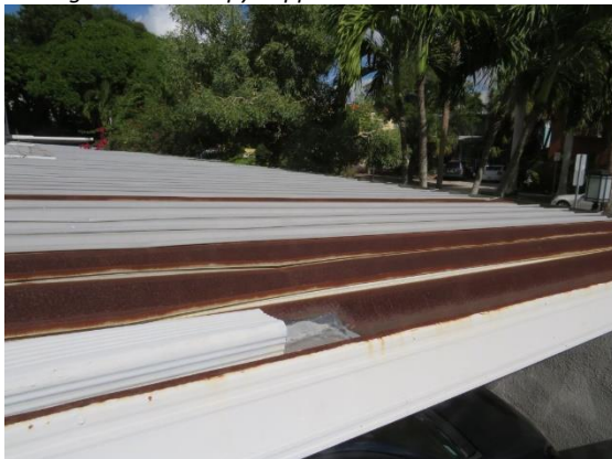
Corroded Metal Deck
