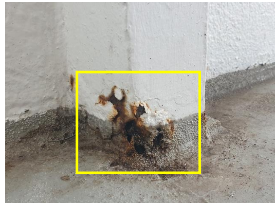
Corrosion at Canopy Support, Voids in Waterproofing
