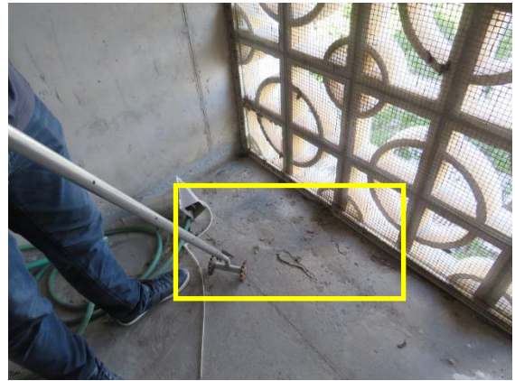
Delaminated Concrete at the Slab Edge
