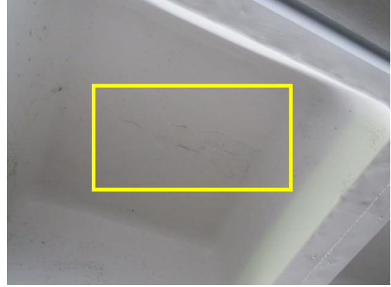
Peeling Paint was Observed in the Slab Voids
