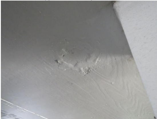
Previous Repairs to the Underside of the Slab
