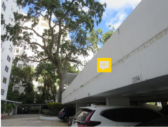
Concrete Spalling at the Western Wall Where an Aluminum Canopy was Previously Installed
