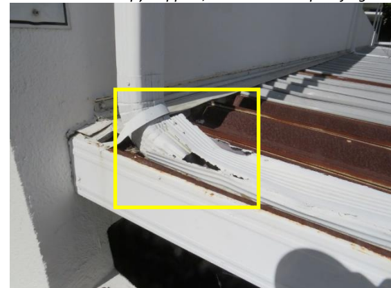
Severe Corrosion / mis-installed Down Spout
