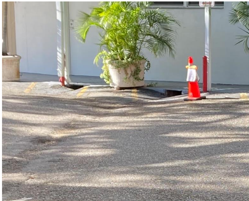
Figure 7B: Asphalt erosion, looking West towards the building.
