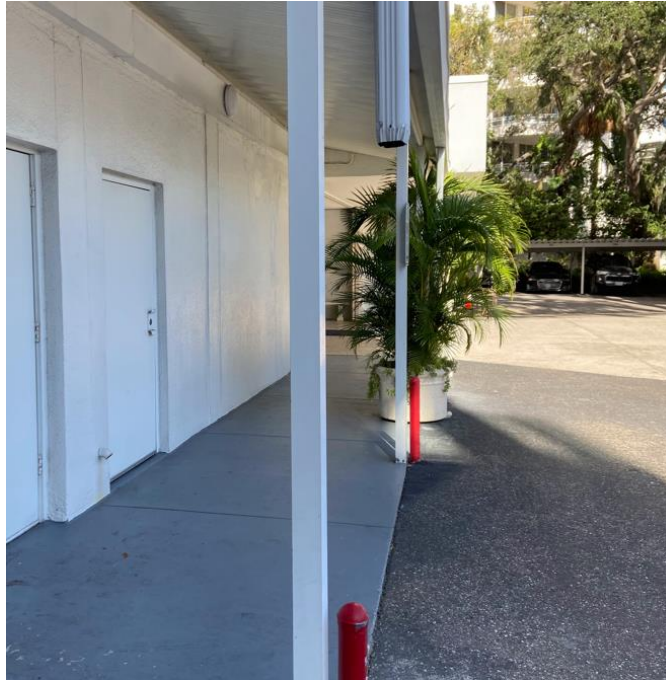
Figure 13: Broken downspout for small roof covering the pedestrian path
