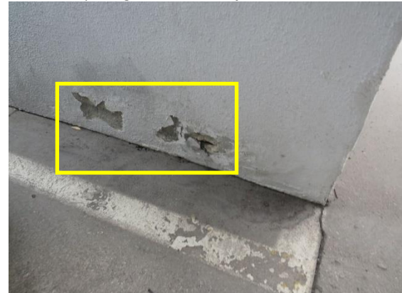
Concrete Spalling at the Walls Adjacent to the Reported
