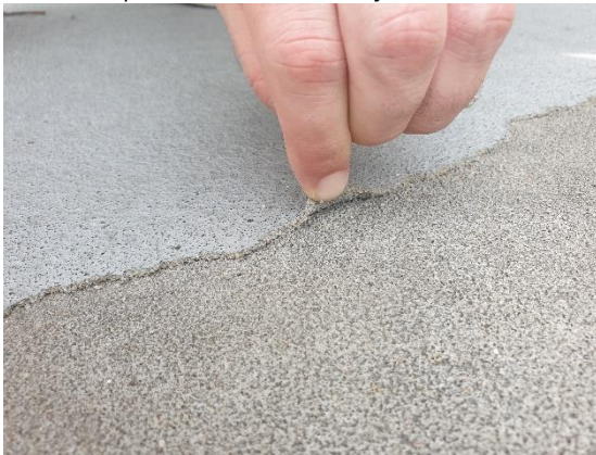
Bond Failure Between Base and Topcoat
