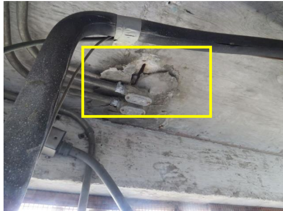
Spalled Concrete to the Underside of the Slab Adjacent to the Conduit
