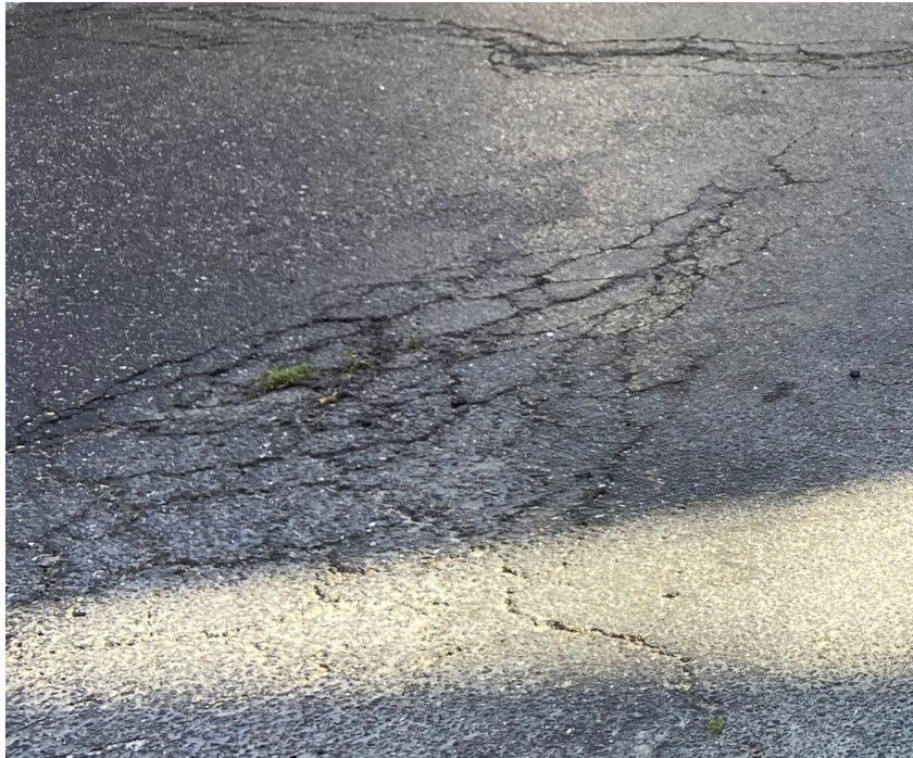
Figure 4: Lot alligator cracking.
