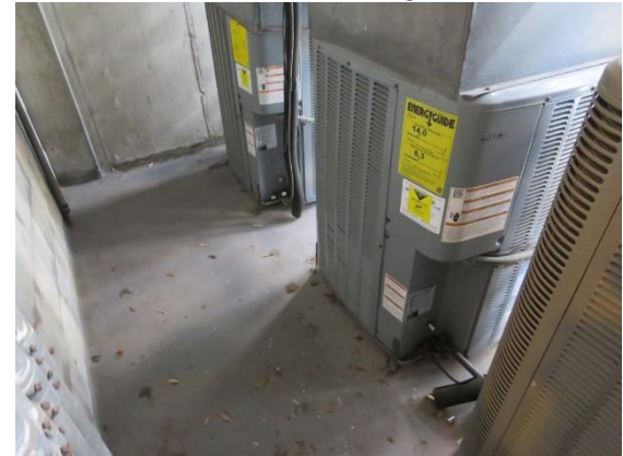
No Waterproofing on the Concrete Slab
