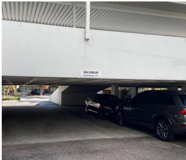
Figure 14: Broken downspout from second level parking
