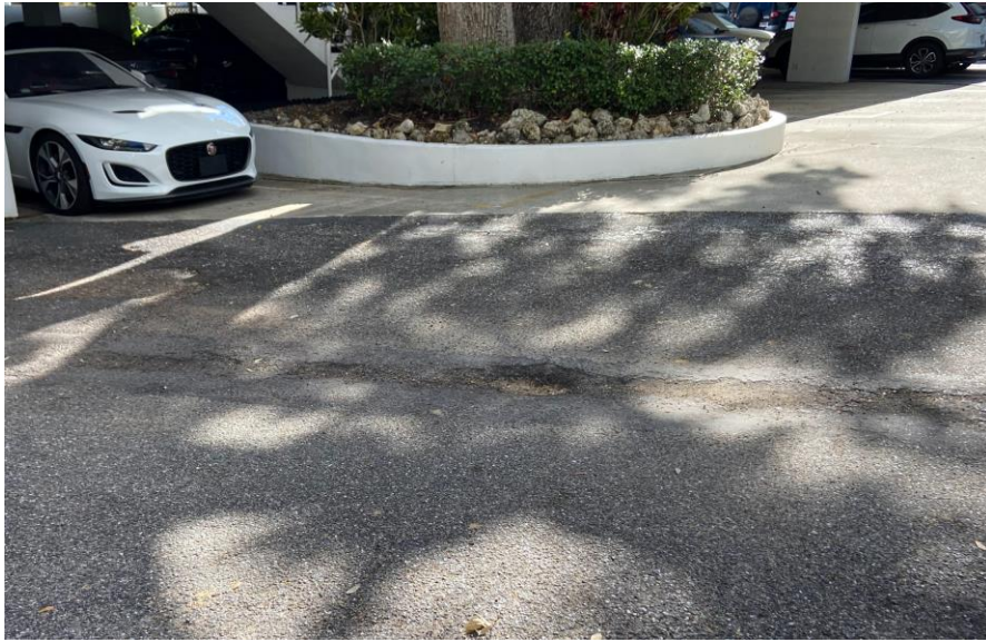
Figure 7A: Asphalt erosion, looking South.
