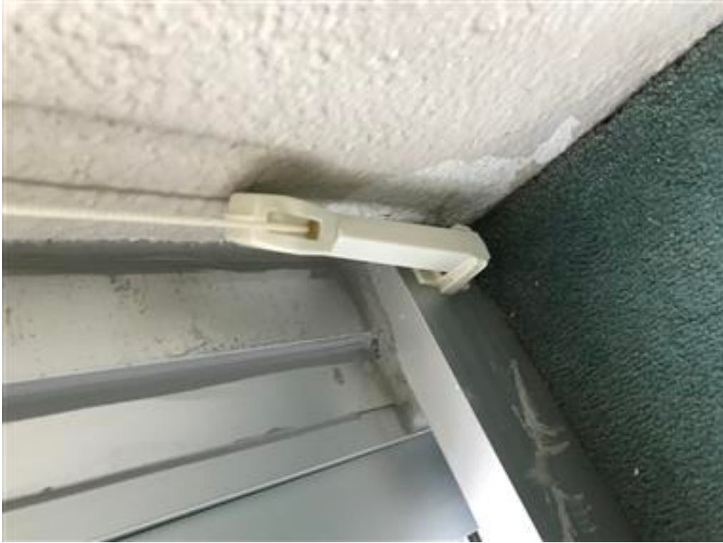
Photo 73-1003, peeling paint at SGD threshold due to water infiltration
