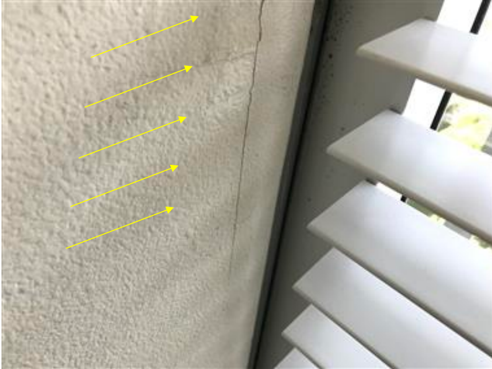
Photo 69-Unit 1002, crack in drywall at SGD, typical
