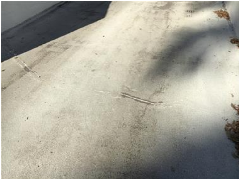
Photo 6-EXIT RAMP- TYPICAL CRACKS
