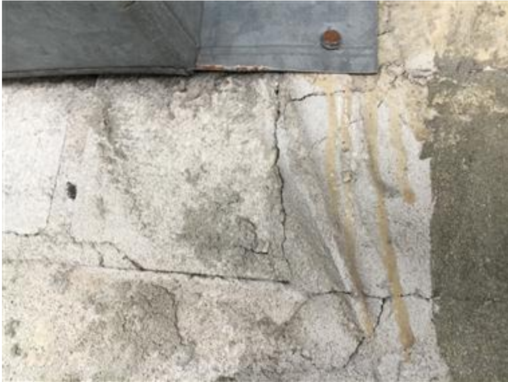
Photo 33-4 th FLOOR- CRACKS
