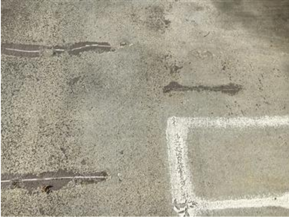
Photo 19- UPPER LEVEL-TYPICAL CRACKS
