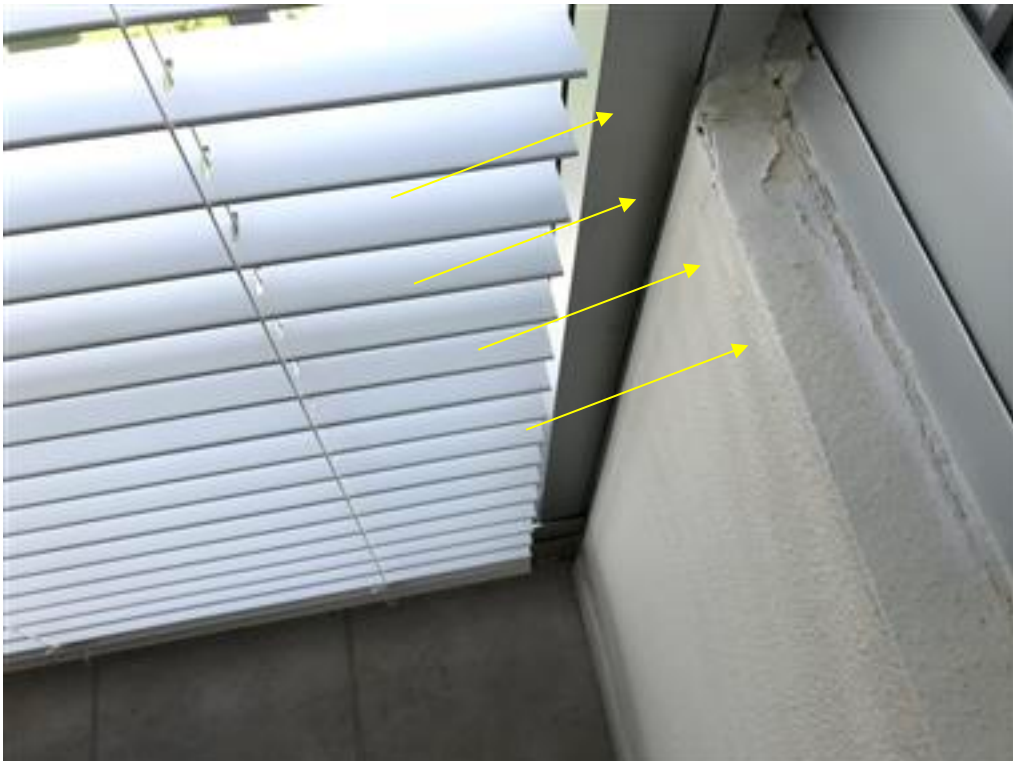
Photo 68-Unit 1004, blistering paint at window sill
