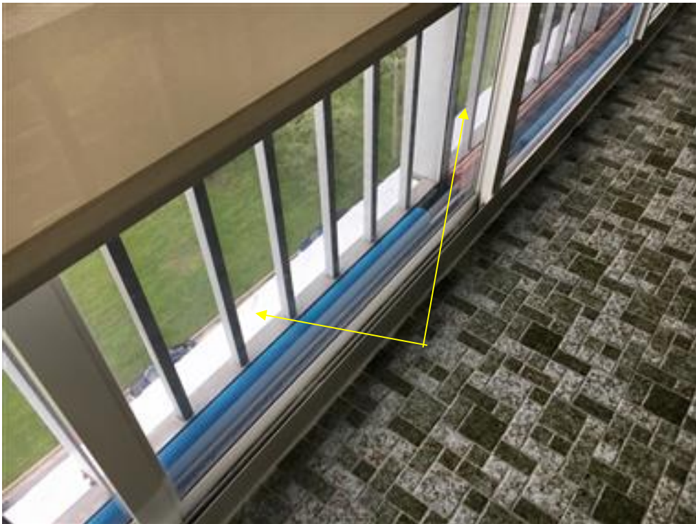
Photo 40-Unit 1203, pool noodles used for possible water absorption at SGD
