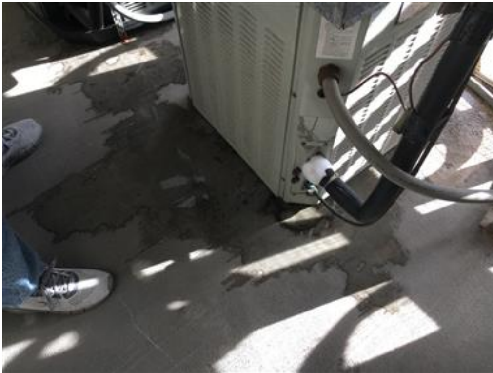
Photo 19-8 th FLOOR- AC LEAK
