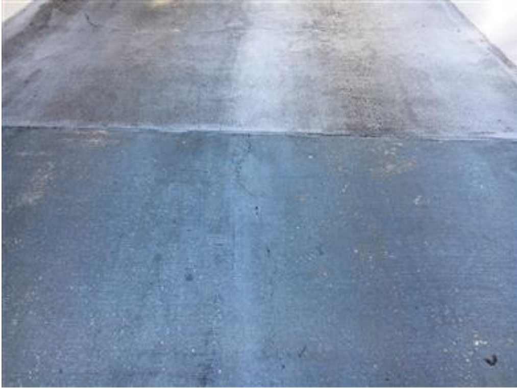
Photo 15-ENTRANCE RAMP- TYPICAL CRACKS
