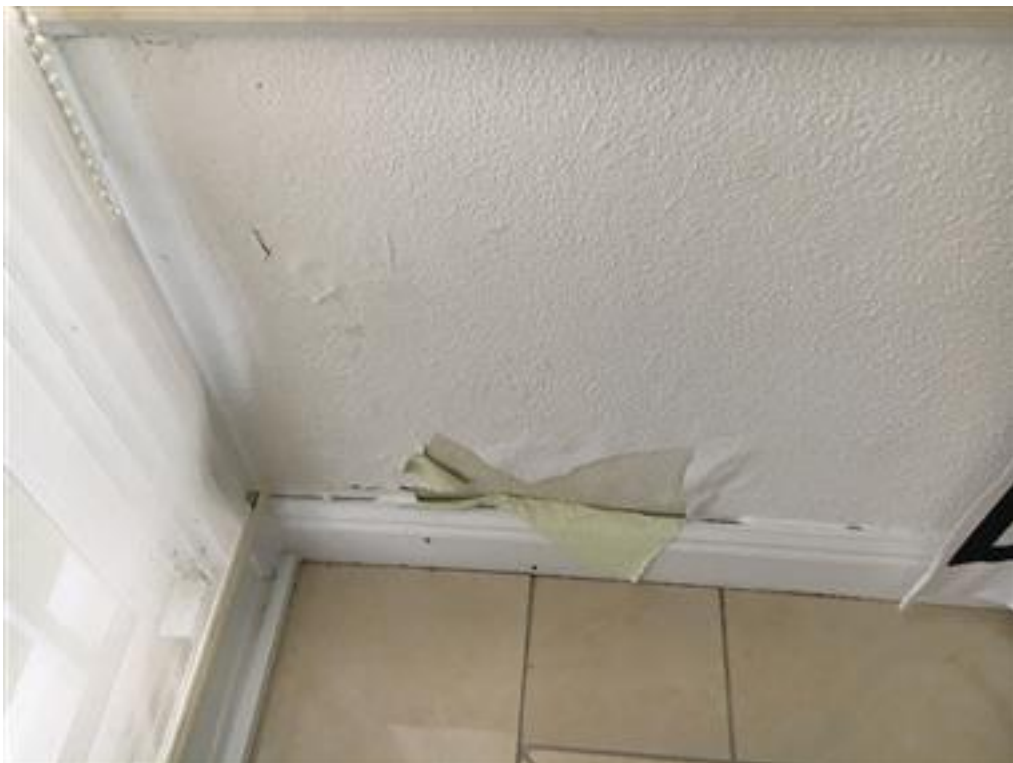
Photo 6-Unit 1601, evidence of water intrusion
