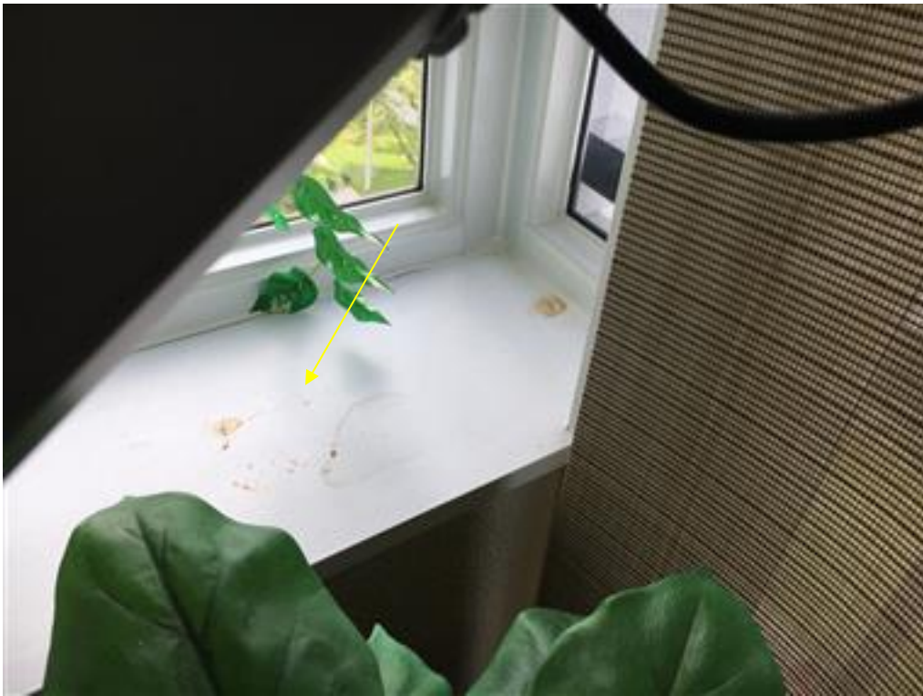
Photo 52-Unit 1103, water stain from evaporated water puddle due to possible water intrusion
