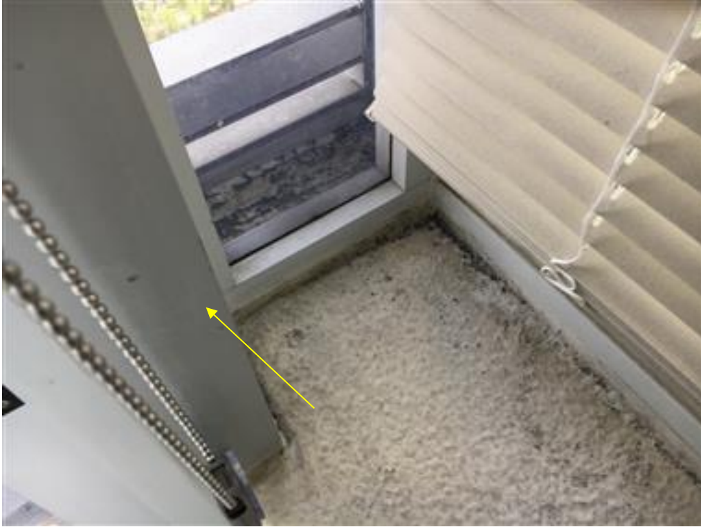
Photo 47-Unit 1202, deteriorated joint sealant
