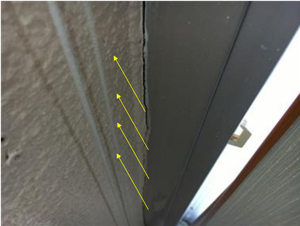
Photo 112-Unit 702, vertical crack at SGD
