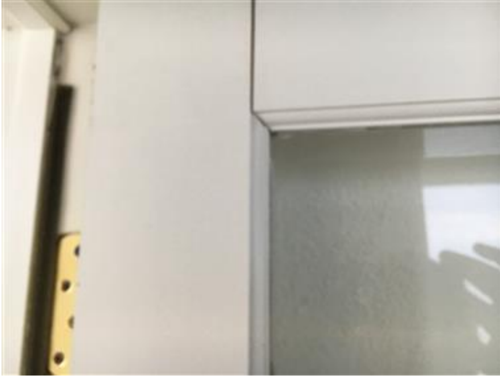
Photo 7-Unit 1601, gap at raised panel door
