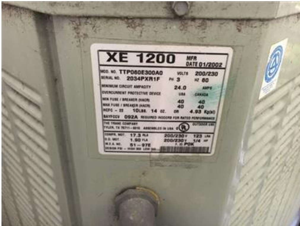
Photo 53-Office Condenser, good condition
