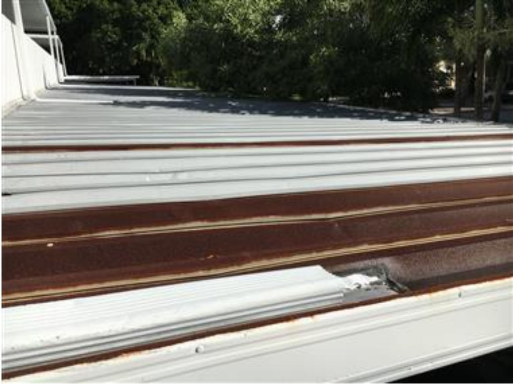
Photo 25- RUSTED CARPORT ROOF NEAR EXIT
