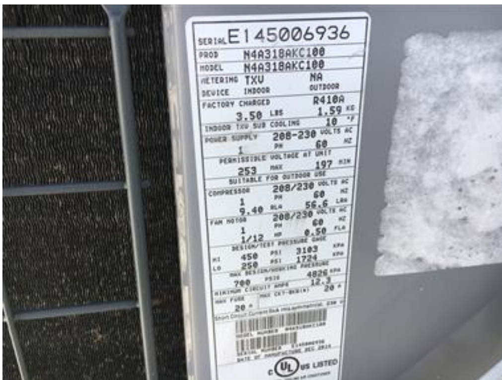
Photo 42-Elevator penthouse condenser, good condition
