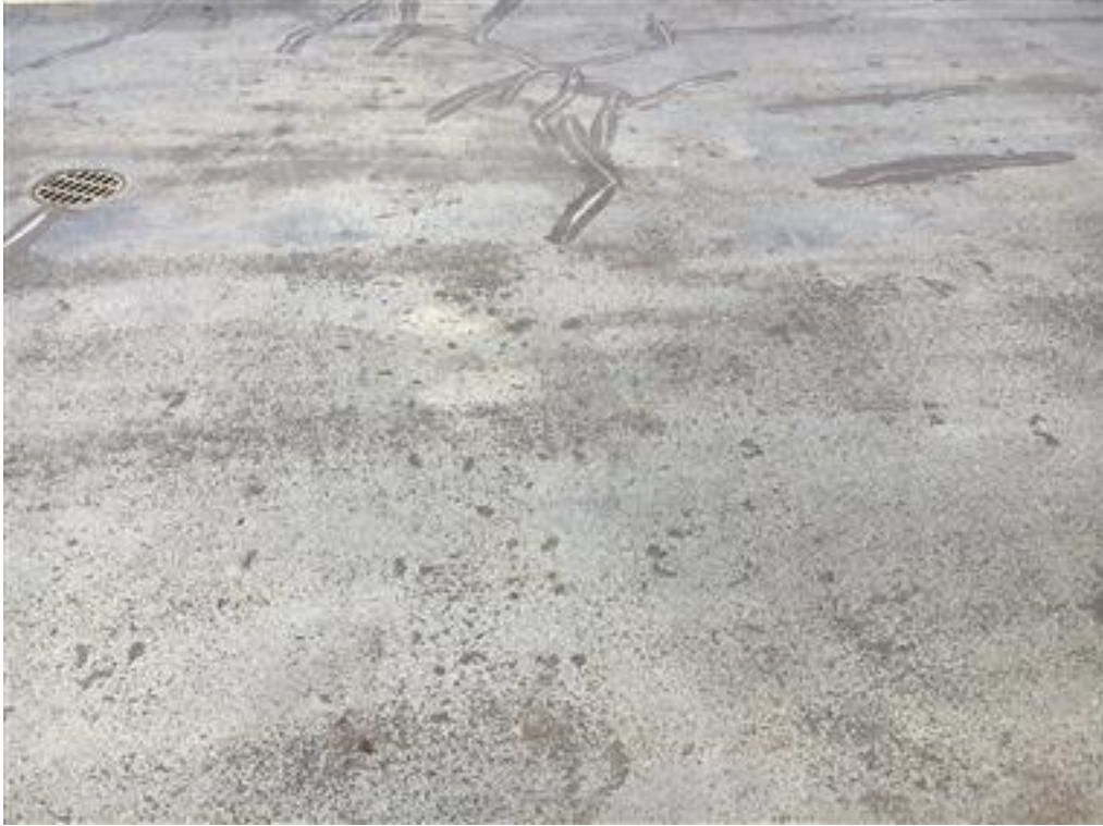
Photo 21- UPPER LEVEL-TYPICAL CRACKS
