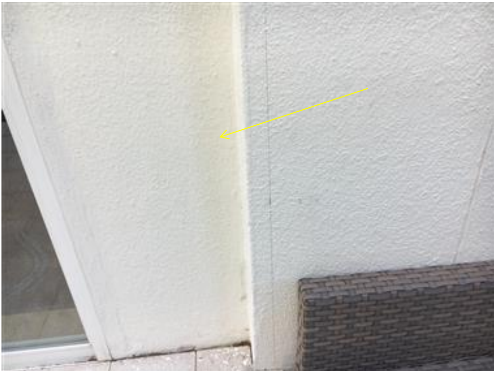
Photo 181-EXTERIOR, vertical stucco crack
