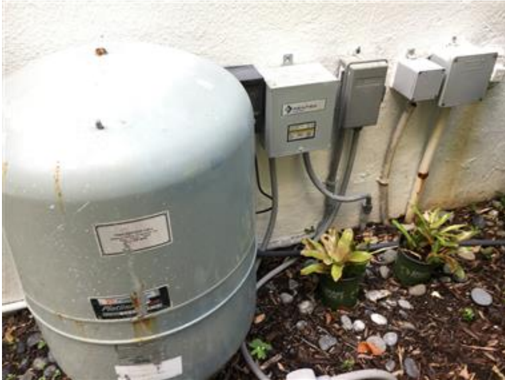
Photo 3- Irrigation controls, good condition
