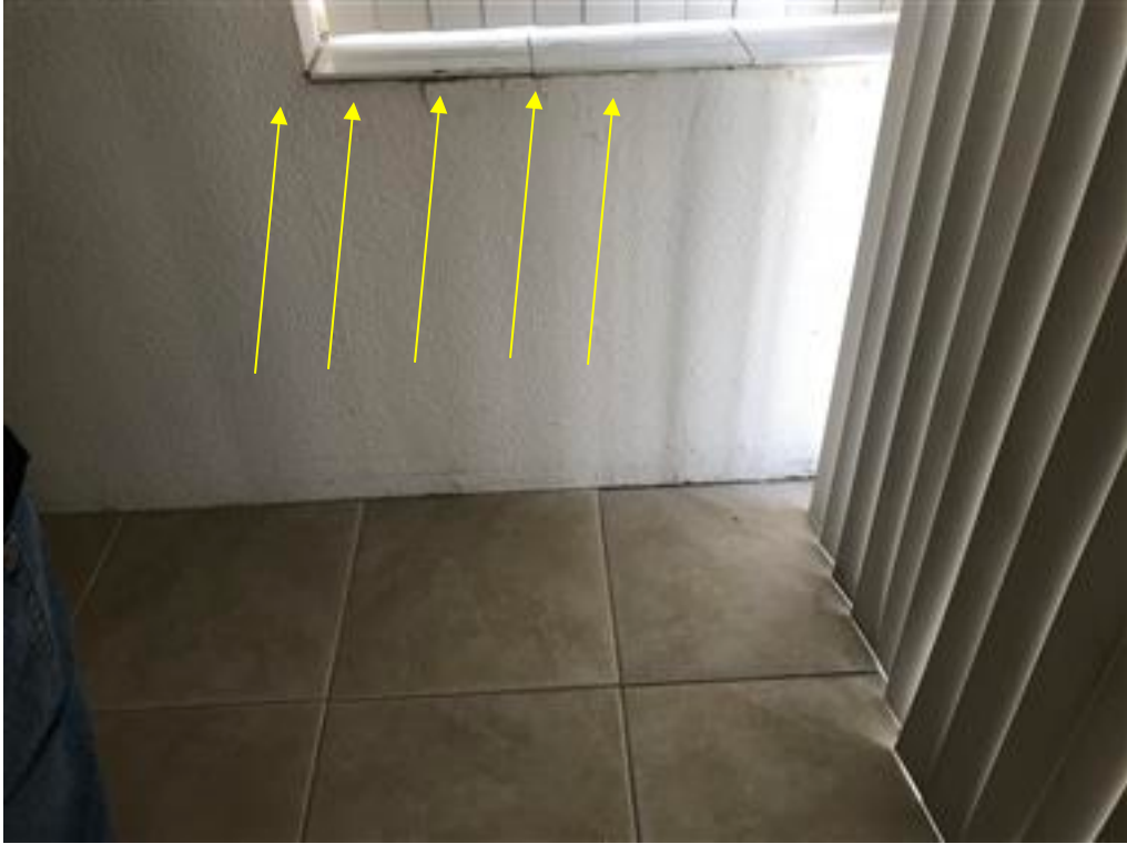
Photo 87-902, paint peeling due to water infiltration
