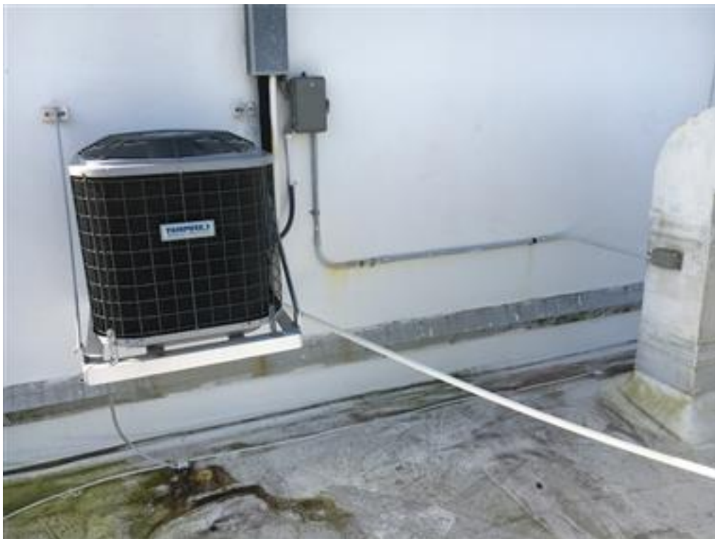
Photo 18-Elevator penthouse AC condenser, good condition, north
