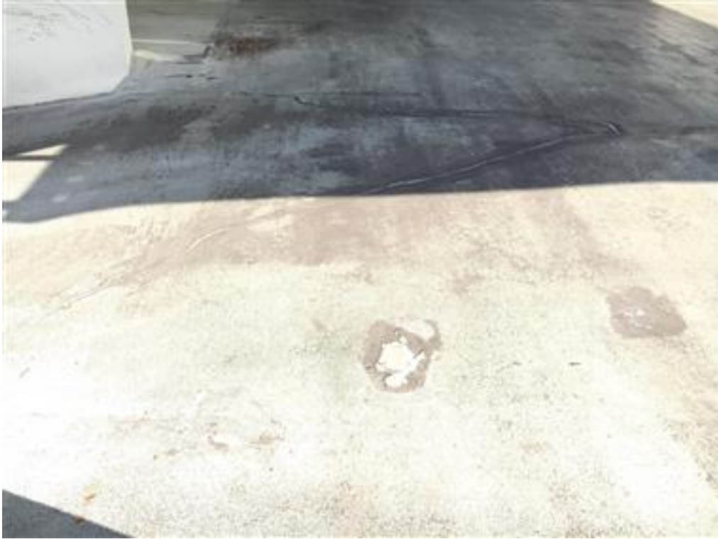
Photo 23- UPPER LEVEL-TYPICAL CRACKS
