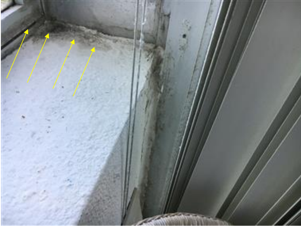
Photo 130-Unit 501, water damage at window sill, typical
