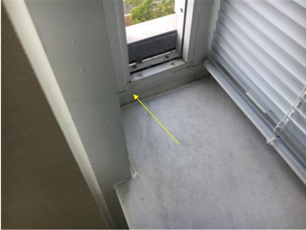
Photo 39-Unit 1203, sealant joint failure
