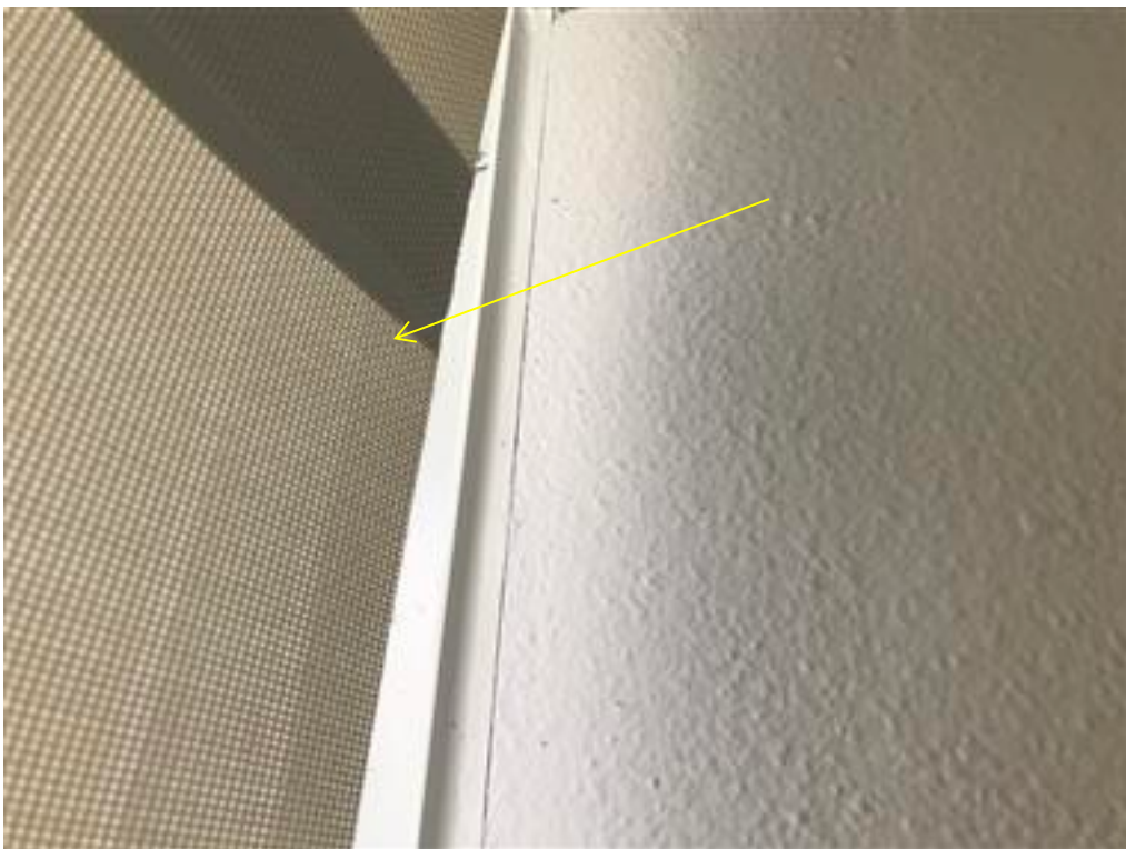
Photo 99-Unit 802, unfamiliar joint at SGD
