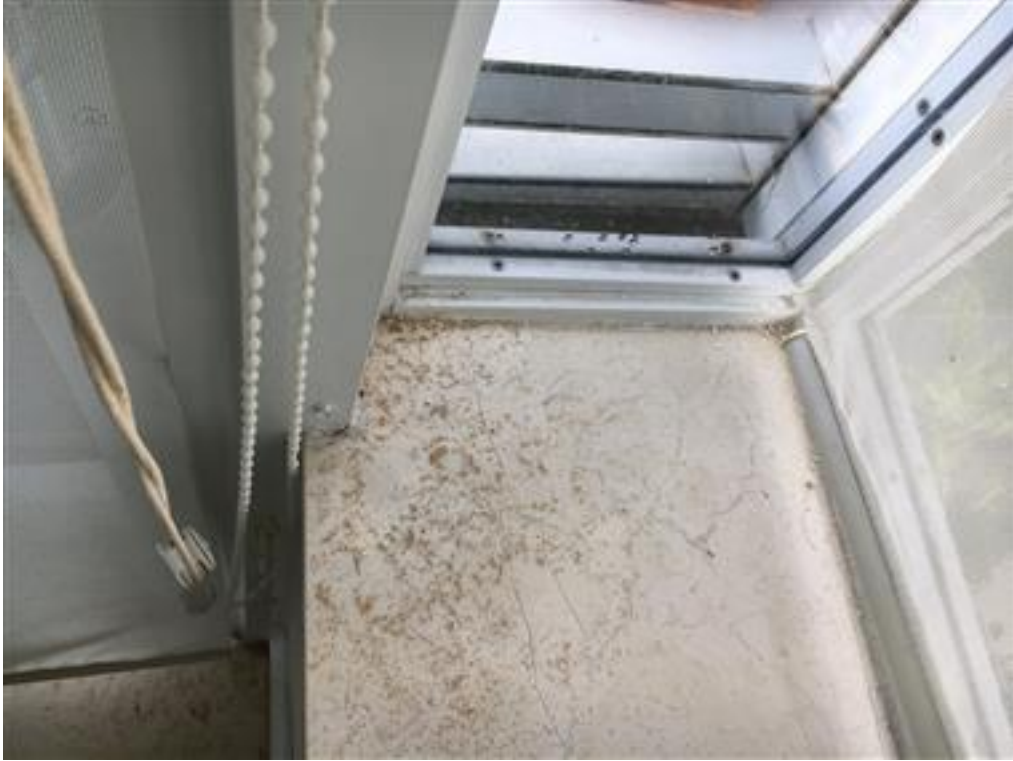
Photo 3-Unit 1601, possible pest infestation
