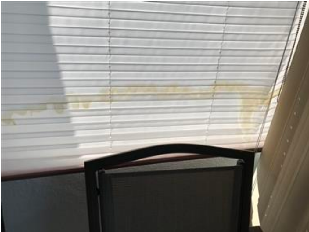
Photo 78-Unit 904, water stain on curtain due to water infiltration
