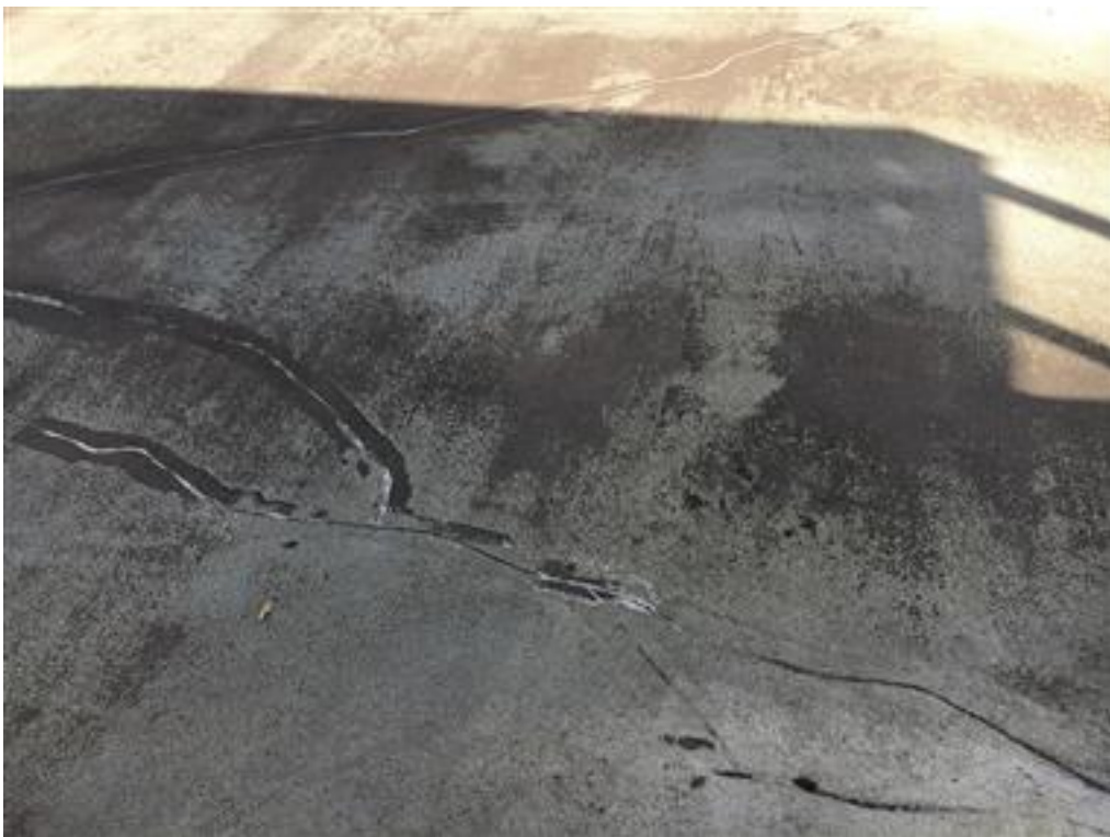
Photo 18-ENTRANCE RAMP- TYPICAL CRACKS
