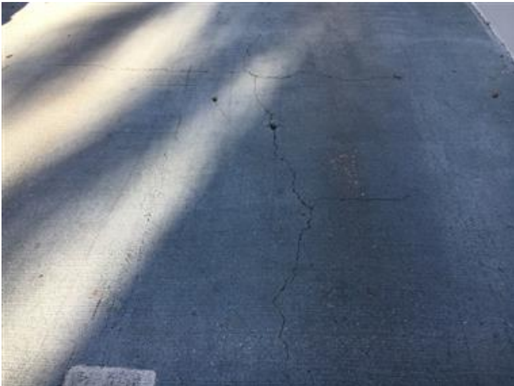
Photo 4-EXIT RAMP- TYPICAL CRACKS
