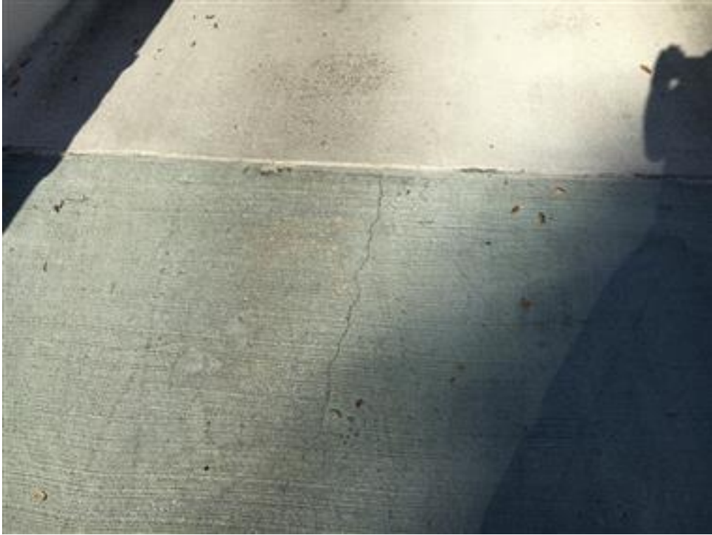
Photo 5-EXIT RAMP- TYPICAL CRACKS
