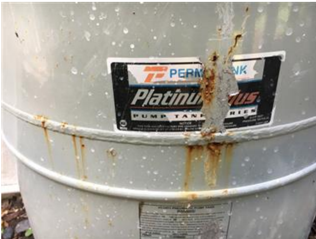
Photo 2- Irrigation pressure tank, average condition
