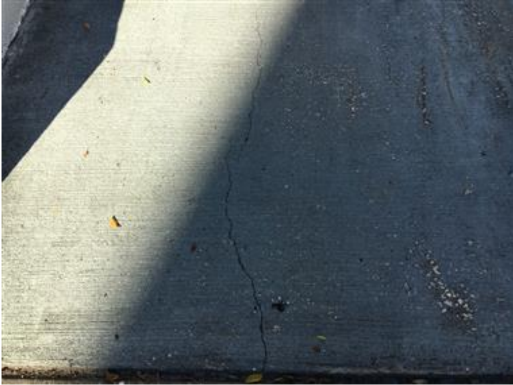
Photo 3- EXIT RAMP- TYPICAL CRACKS
