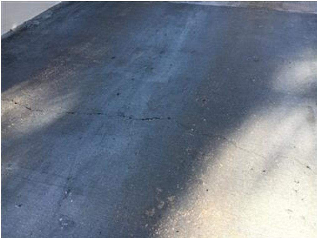
Photo 14-ENTRANCE RAMP- TYPICAL CRACKS
