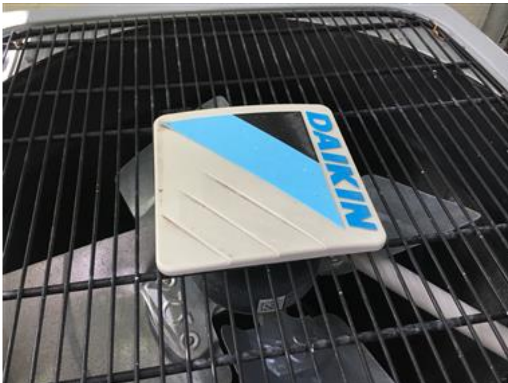
Photo 54-Unit 101 AC condenser, good condition
