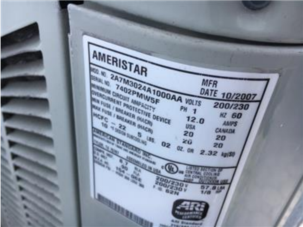
Photo 49-Men's room/storage unit AC condenser, good condition
