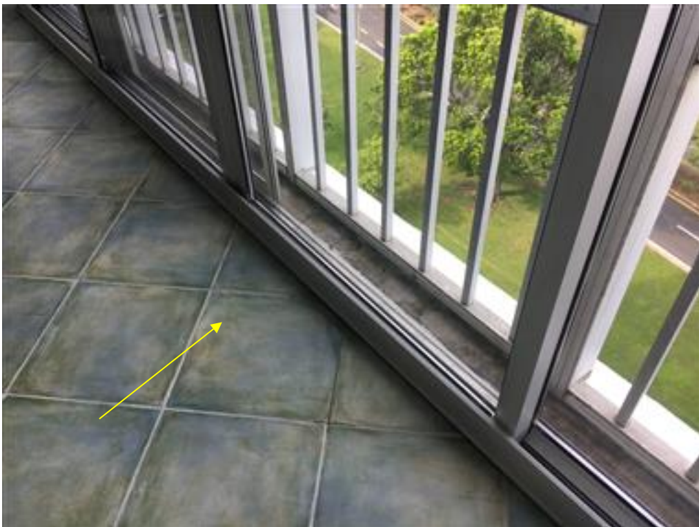
Photo 32-1404, alternate view of water leak at SGD
