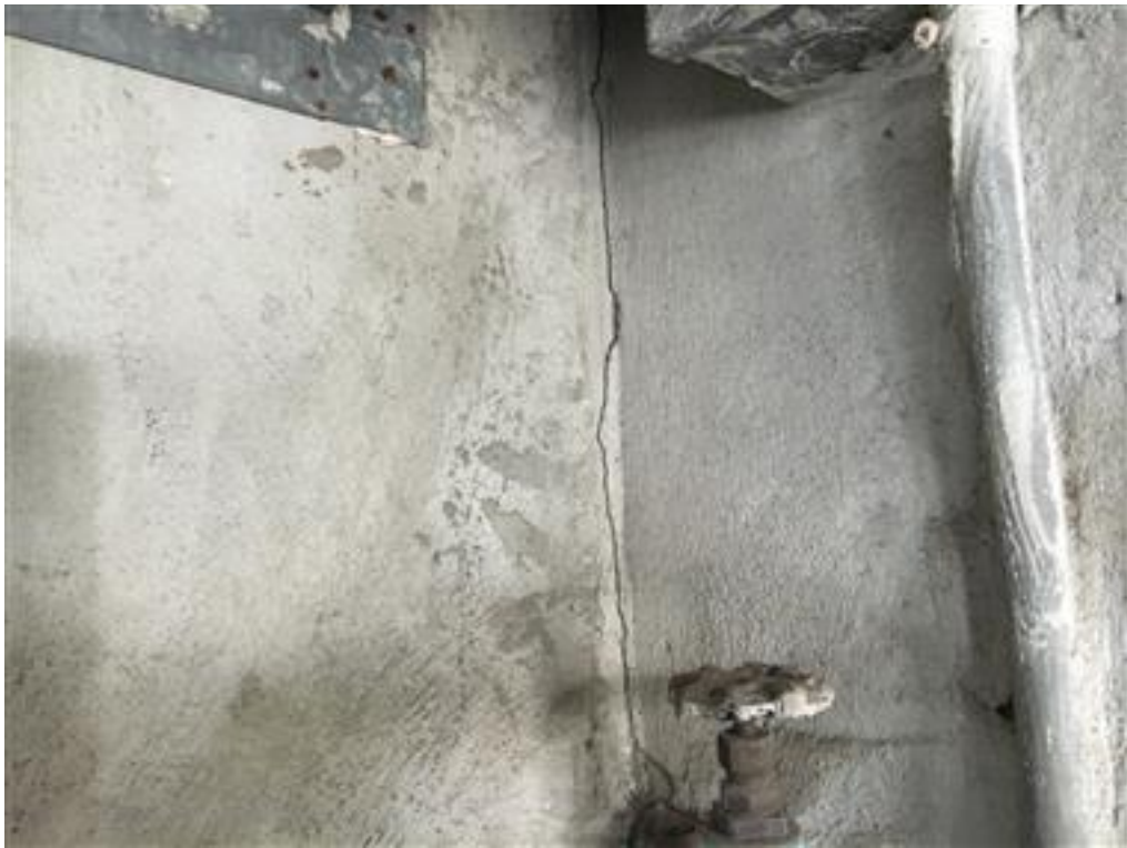
Photo 36-3 RD FLOOR- CRACK
