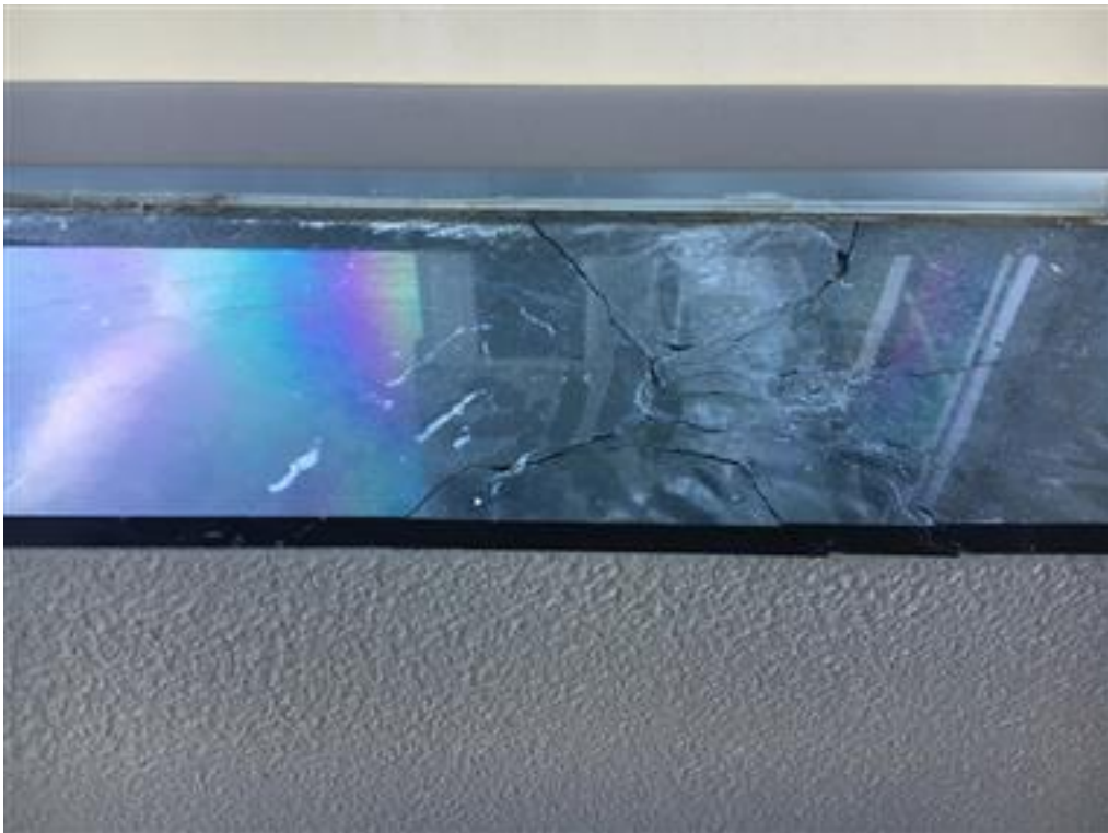
Photo 177-Unit 304, cracked marble sill, typical
