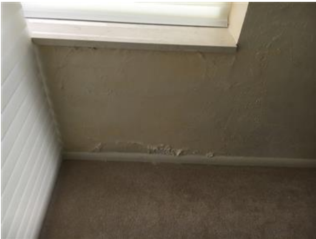
Photo 8-Unit 1602, evidence of water intrusion
