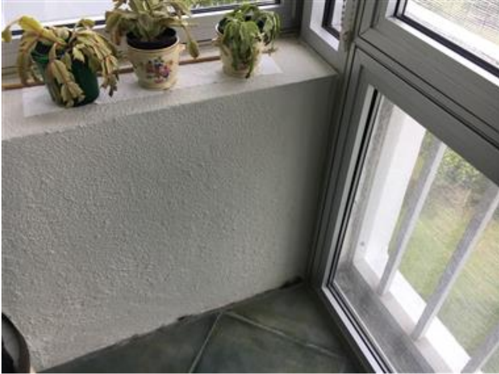
Photo 31-1404, evidence of water damage
