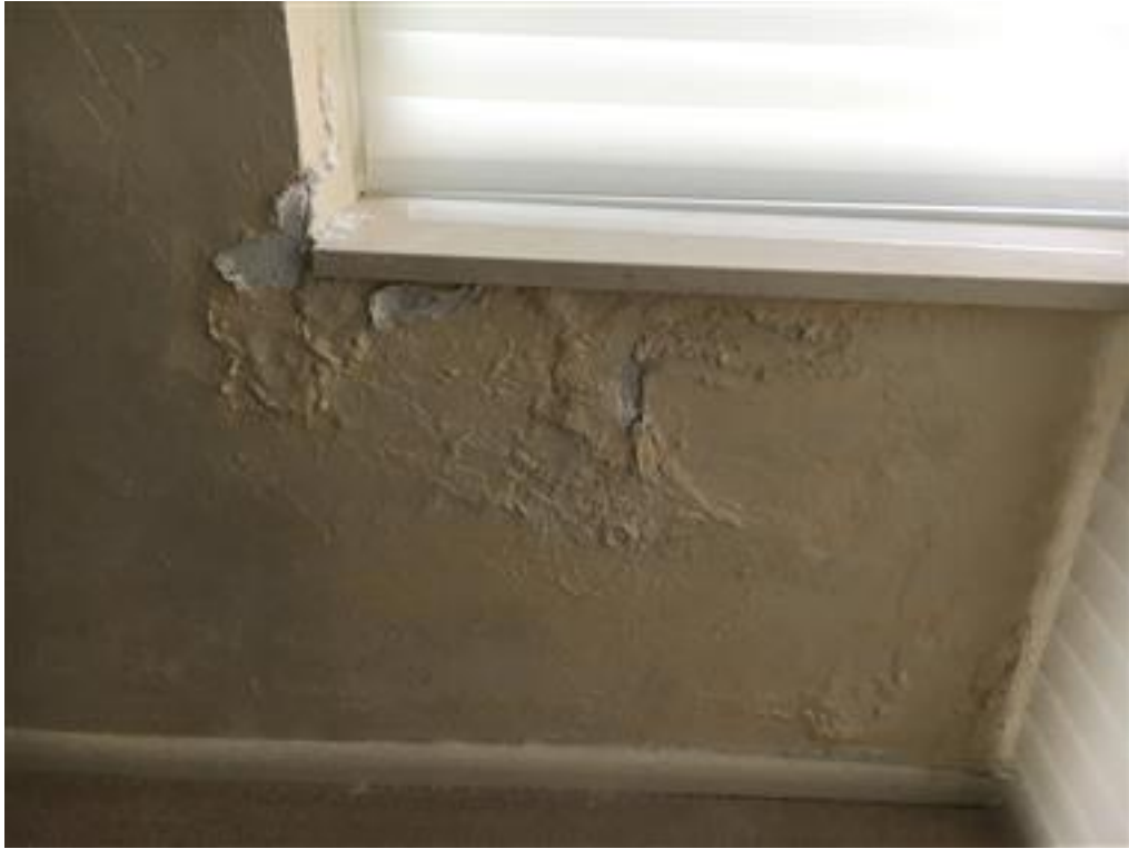
Photo 9-Unit 1602, evidence of water intrusion
