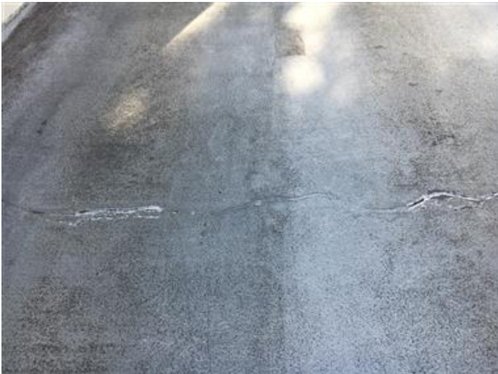
Photo 16-ENTRANCE RAMP- TYPICAL CRACKS
