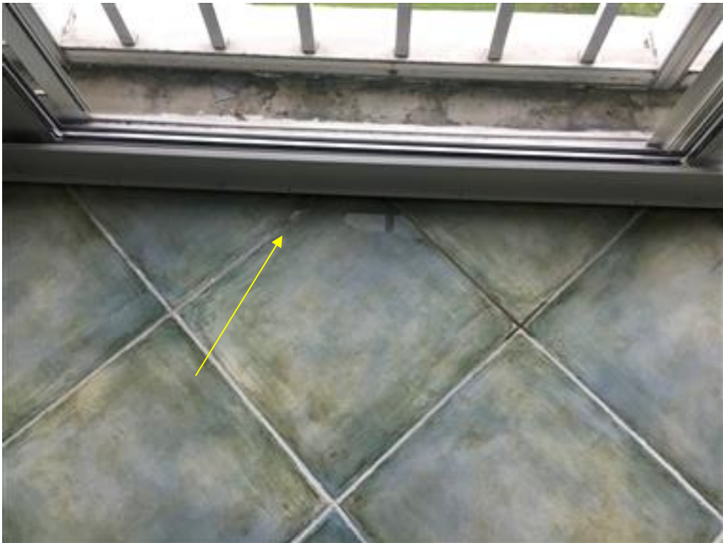
Photo 30-Unit 1404, water leak at SGD
