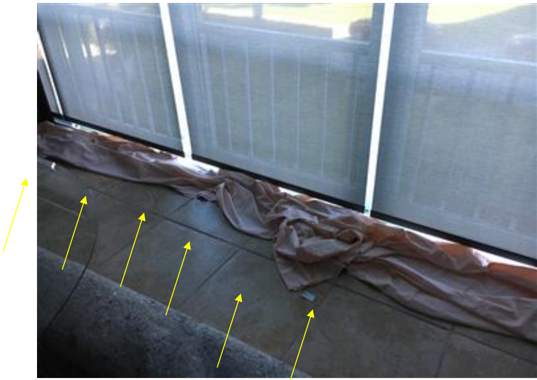
Photo 167-Unit 204, evidence of water intrusion utilizing a sheet to absorb water infiltration
