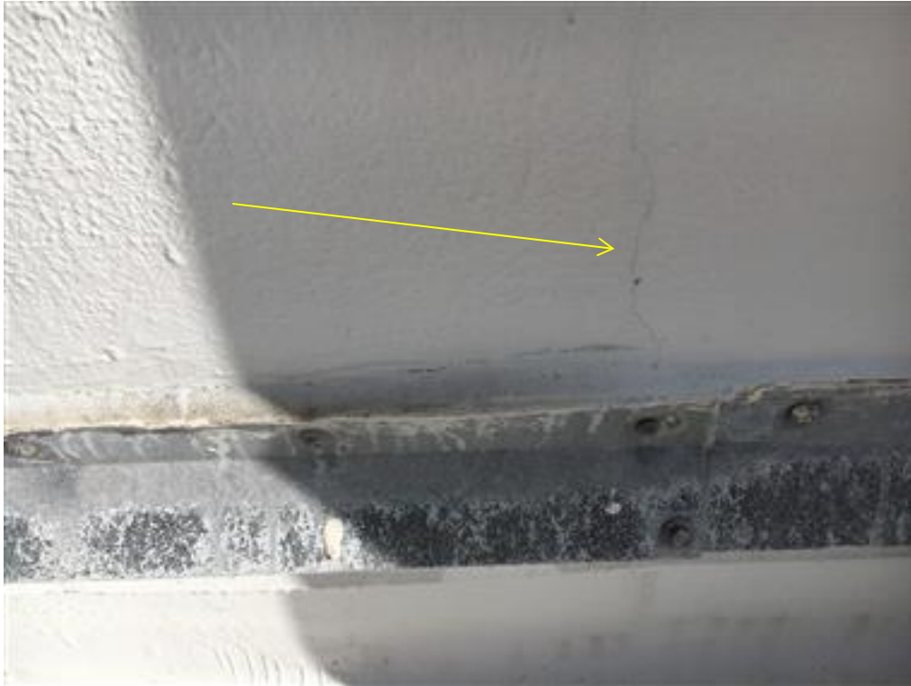
Photo 41-Elevator penthouse, hairline crack at south end
