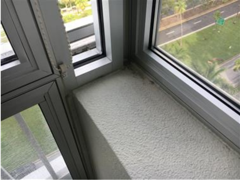
Photo 29-Unit 1404, evidence of water intrusion
