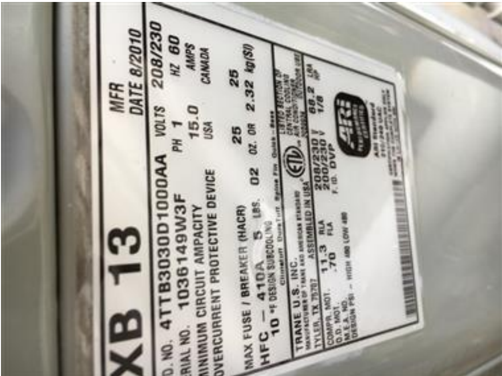
Photo 50-Kitchen AC condenser, good condition
