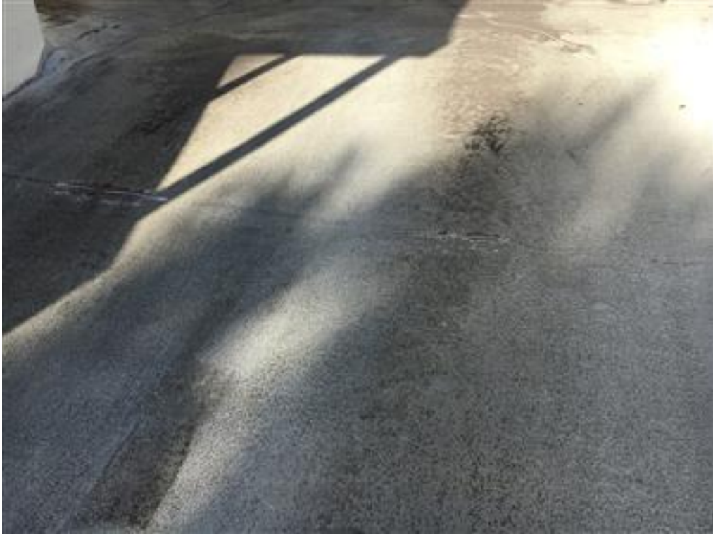
Photo 17-ENTRANCE RAMP- TYPICAL CRACKS
