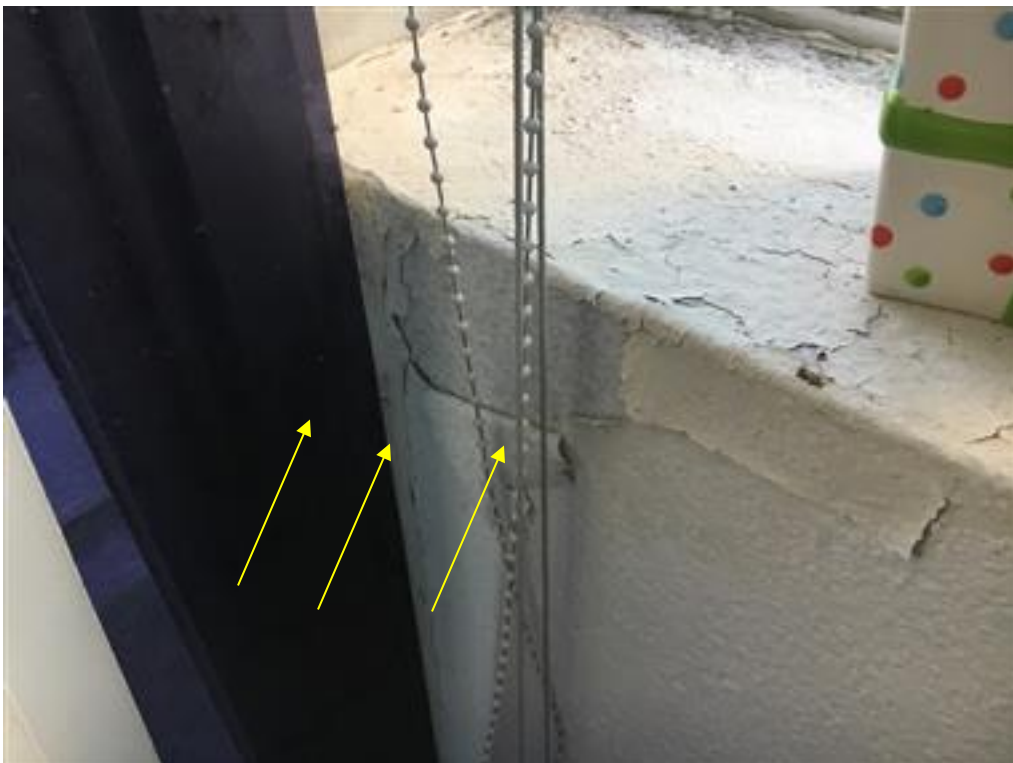
Photo 131-Unit 501, water damage at window sill
