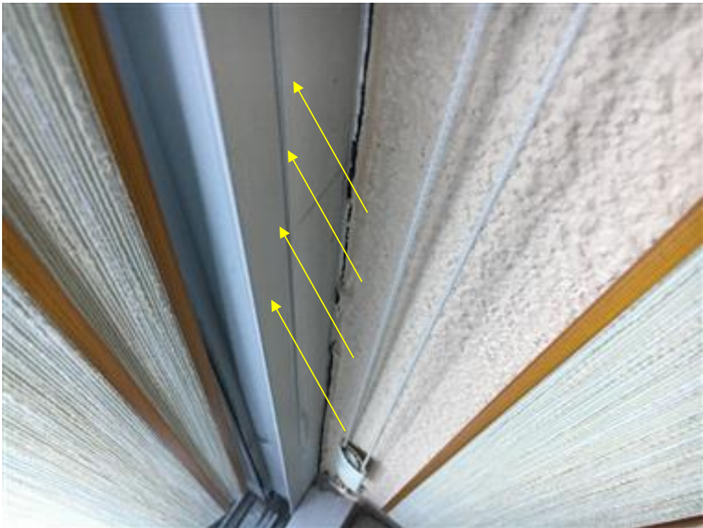
Photo 111-Unit 702, vertical crack at SGD, typical
