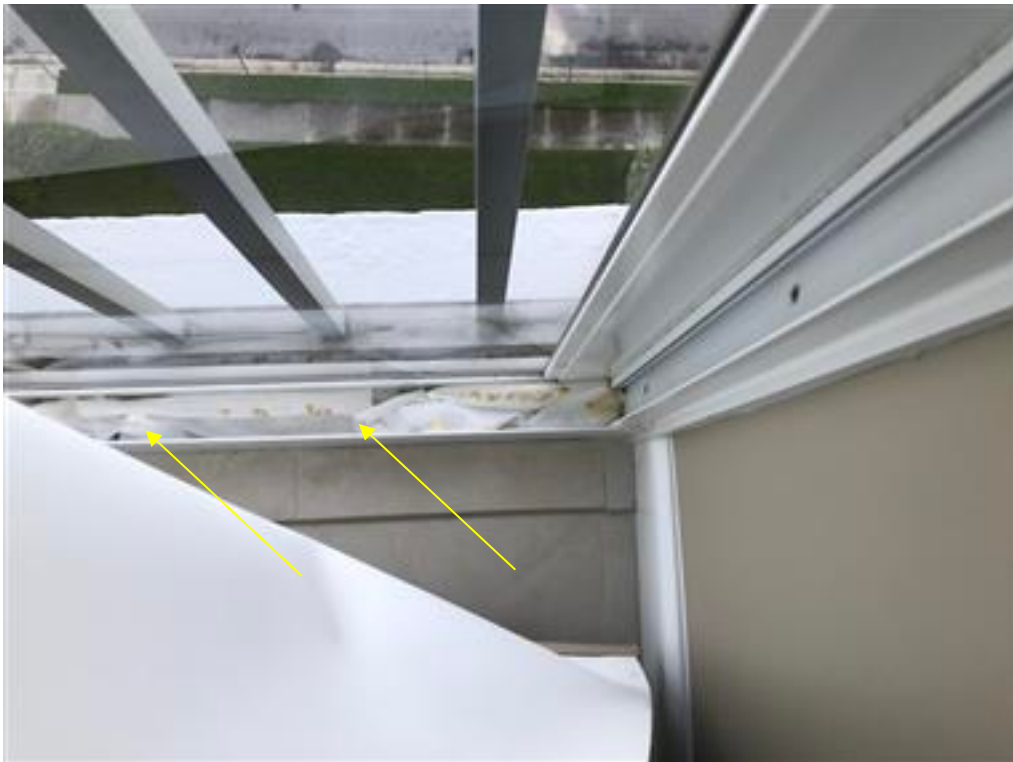
Photo 60-Unit 1001, material used for water absorption at SGD, typical
