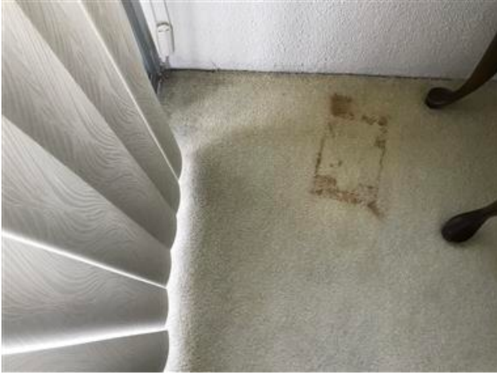
Photo 65-Unit 1002, evidence of water intrusion from rust stain on carpet
