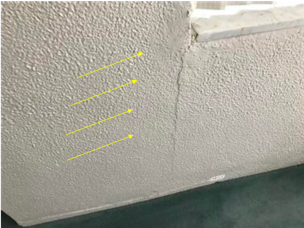
Photo 74-Unit 1003, hairline crack at window sill, typical
