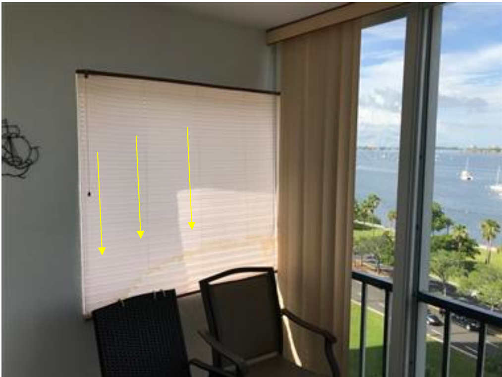
Photo 76-Unit 904, water stain on curtain due to water infiltration
