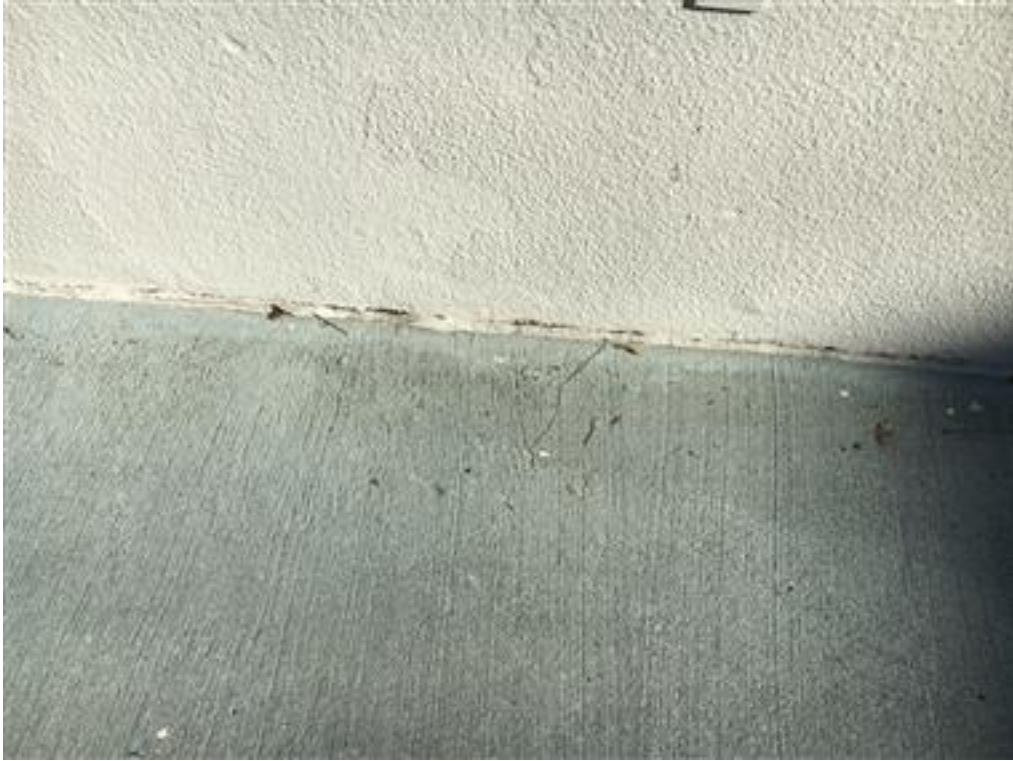
Photo 13-ENTRANCE RAMP- TYPICAL CRACKS
