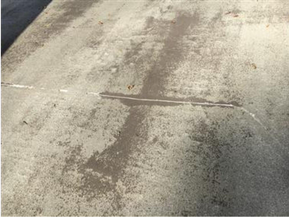
Photo 7-EXIT RAMP- TYPICAL CRACKS
