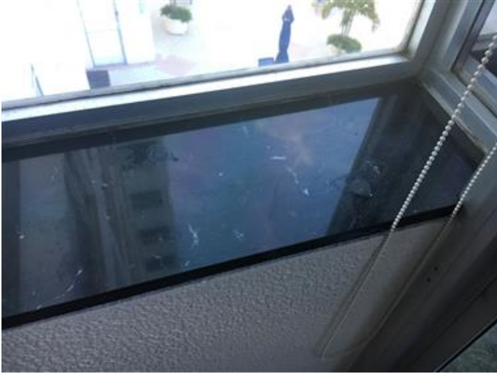
Photo 178-Unit 304, cracked marble sill
