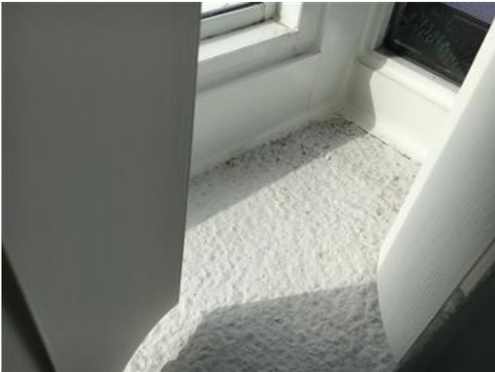
Photo 26-Unit 1404, Water damage at sill
