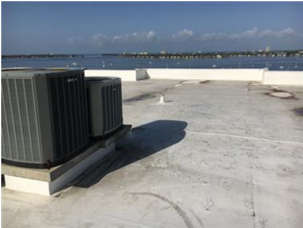
Photo 14-General view, AC curbs, ponding
