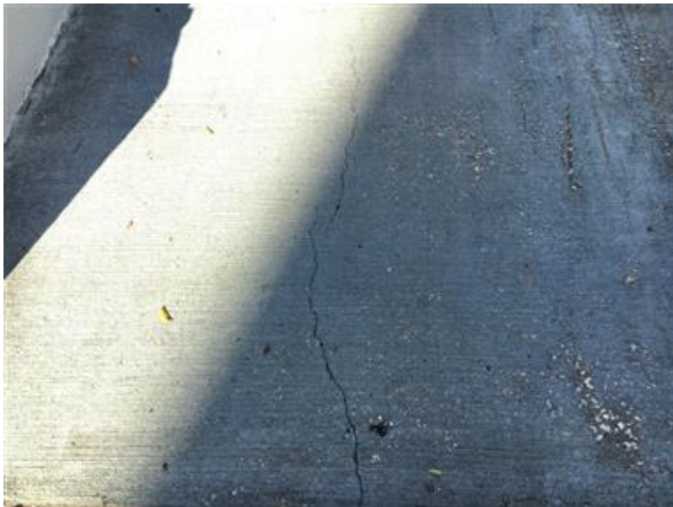
Photo 2-EXIT RAMP- TYPICAL CRACKS
