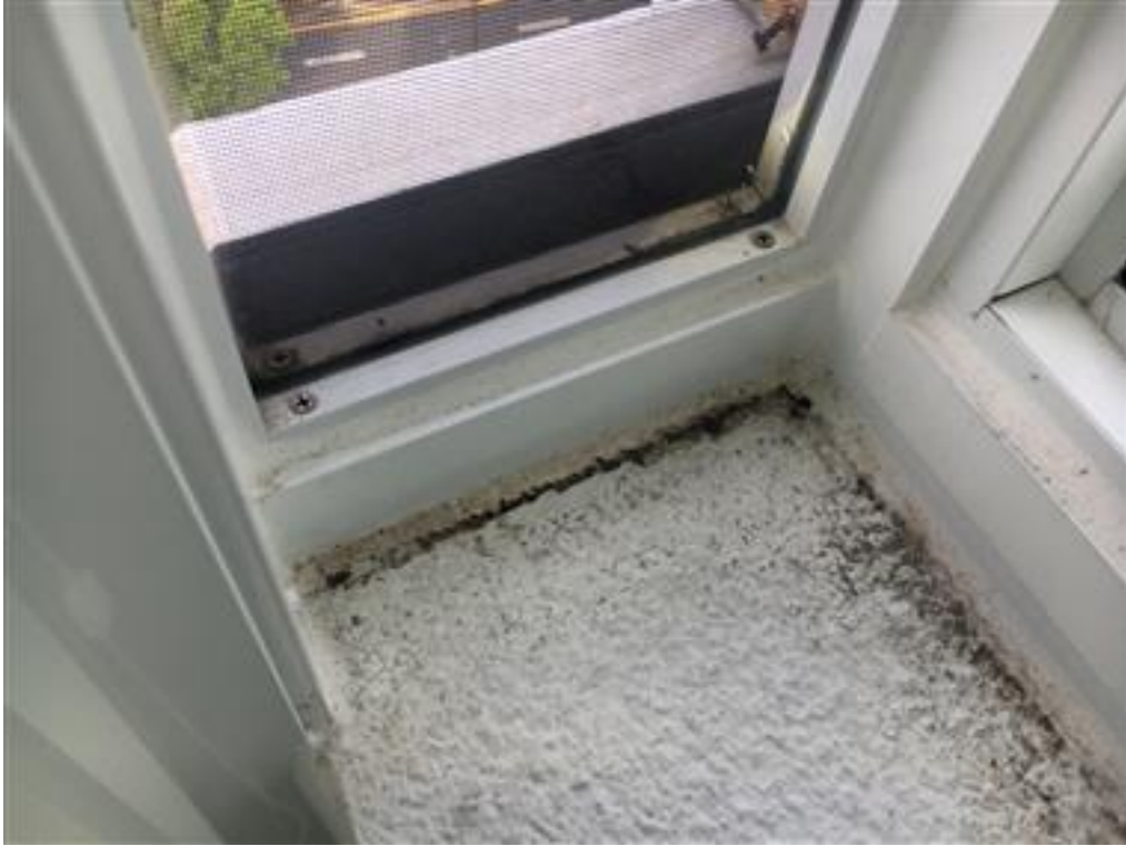
Photo 25-Unit 1404, Water damage at sill, typical
