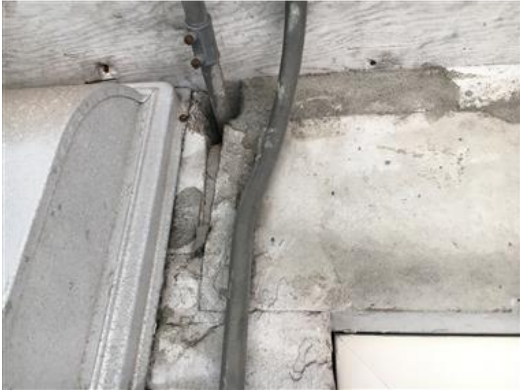
Photo 23-7 th FLOOR- VOIDS
