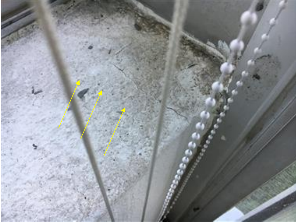
Photo 134-Unit 501, water damage at window sill
