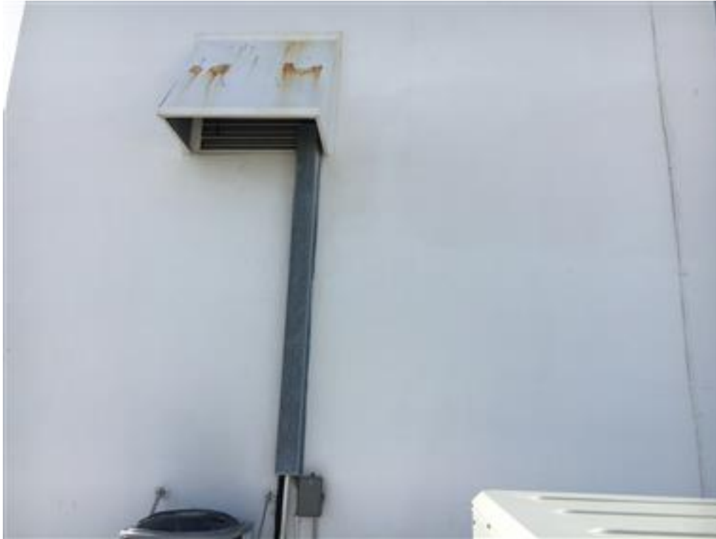
Photo 17-Elevator penthouse, rusted vent hood, north elevator penthouse
