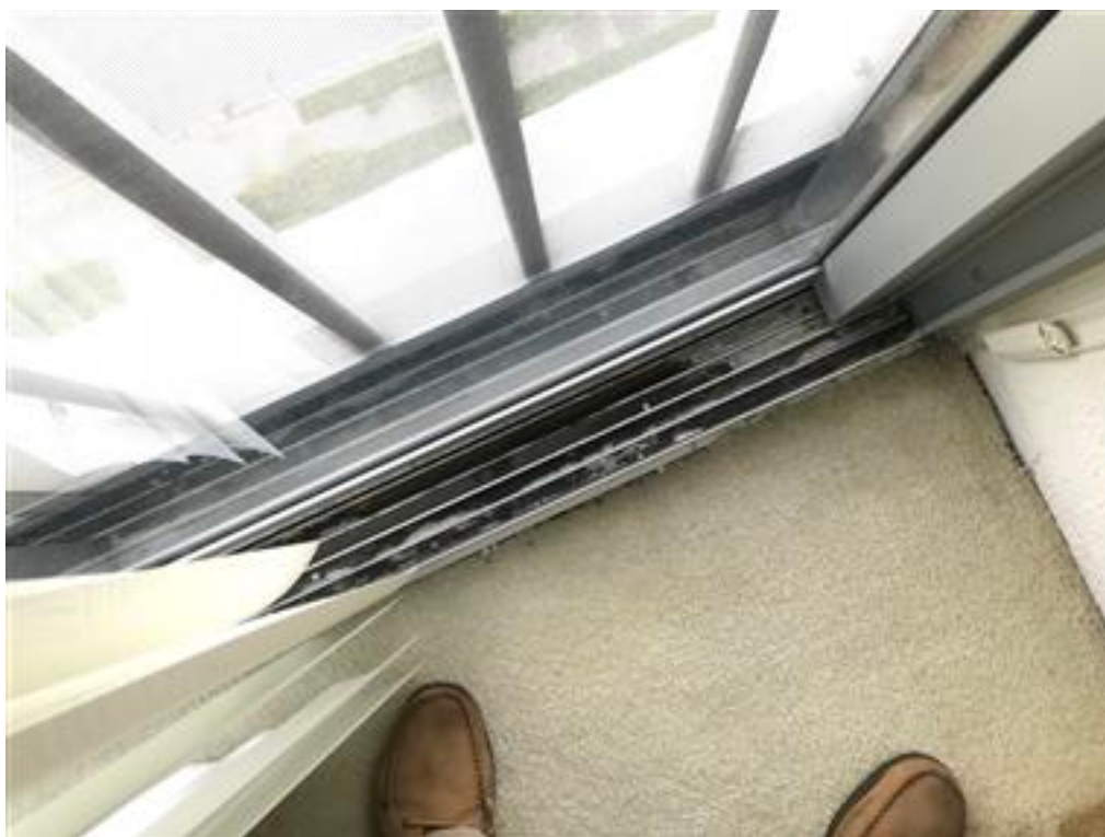
Photo 64-Unit 1002, evidence of water intrusion at SGD threshold
