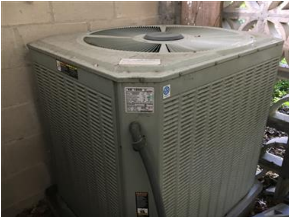
Photo 52-Office Condenser, good condition
