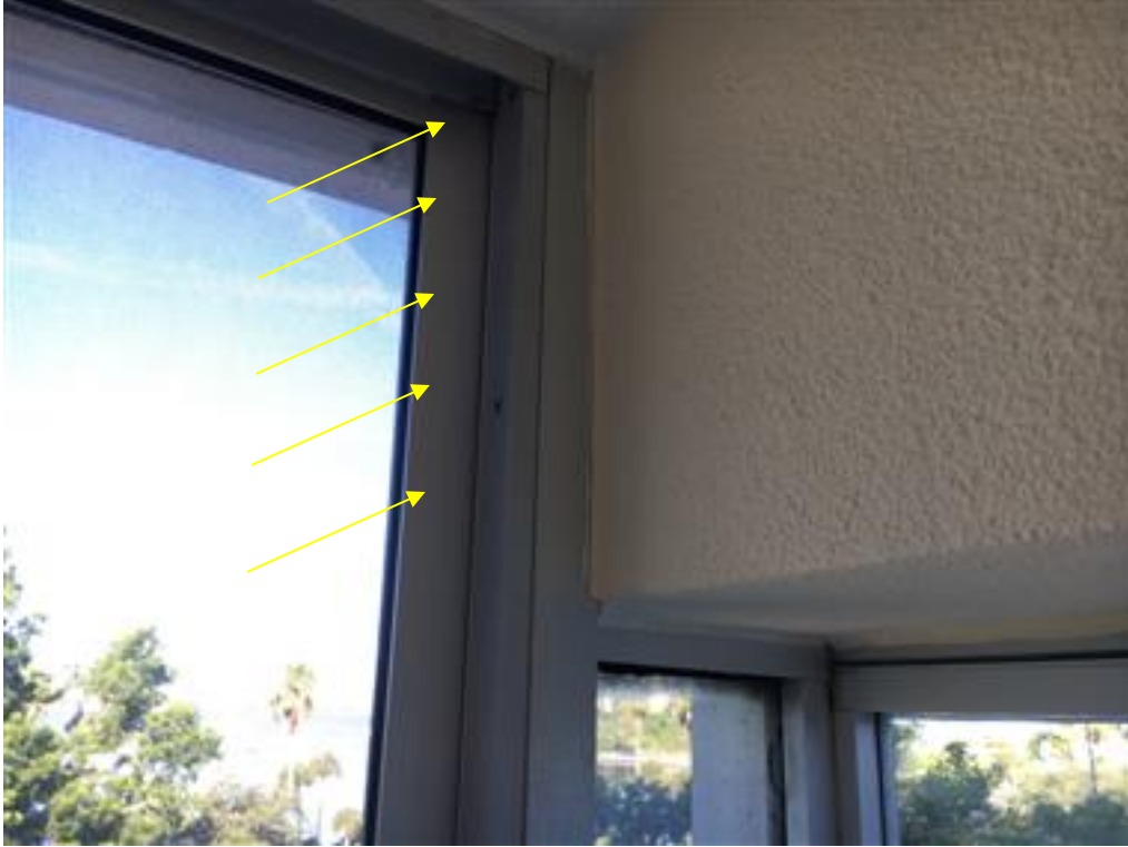
Photo 146-Unit 405, open crack at SGD above window
