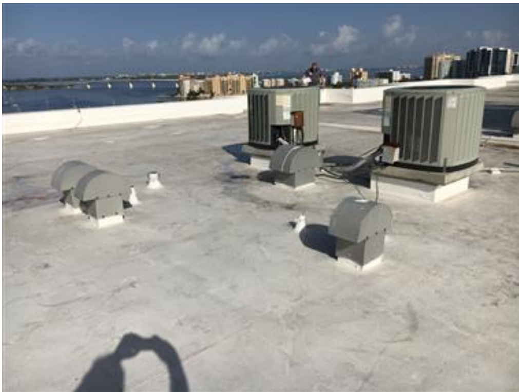
Photo 28-General view, AC stands, vents
