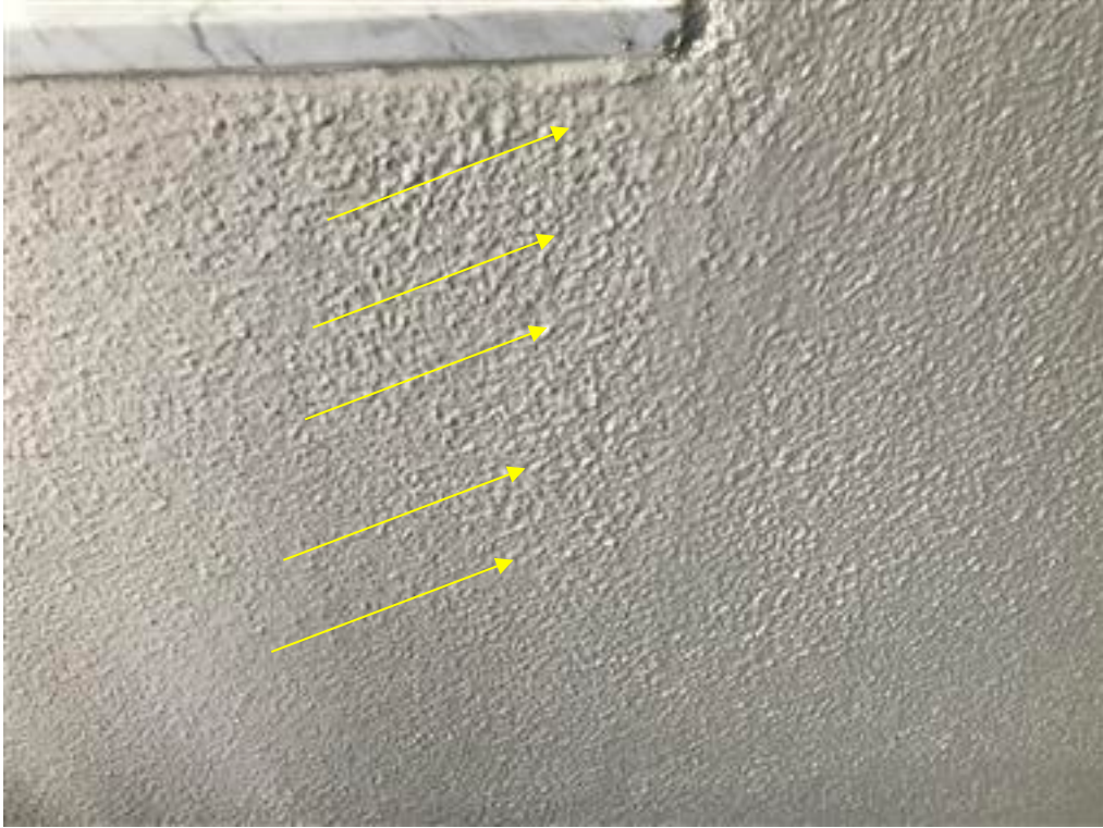
Photo 75-Unit 1002, hairline crack at window sill, typical
