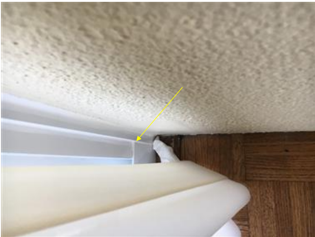
Photo 44-Unit 1201, tissues used to absorb water intrusion at SGD
