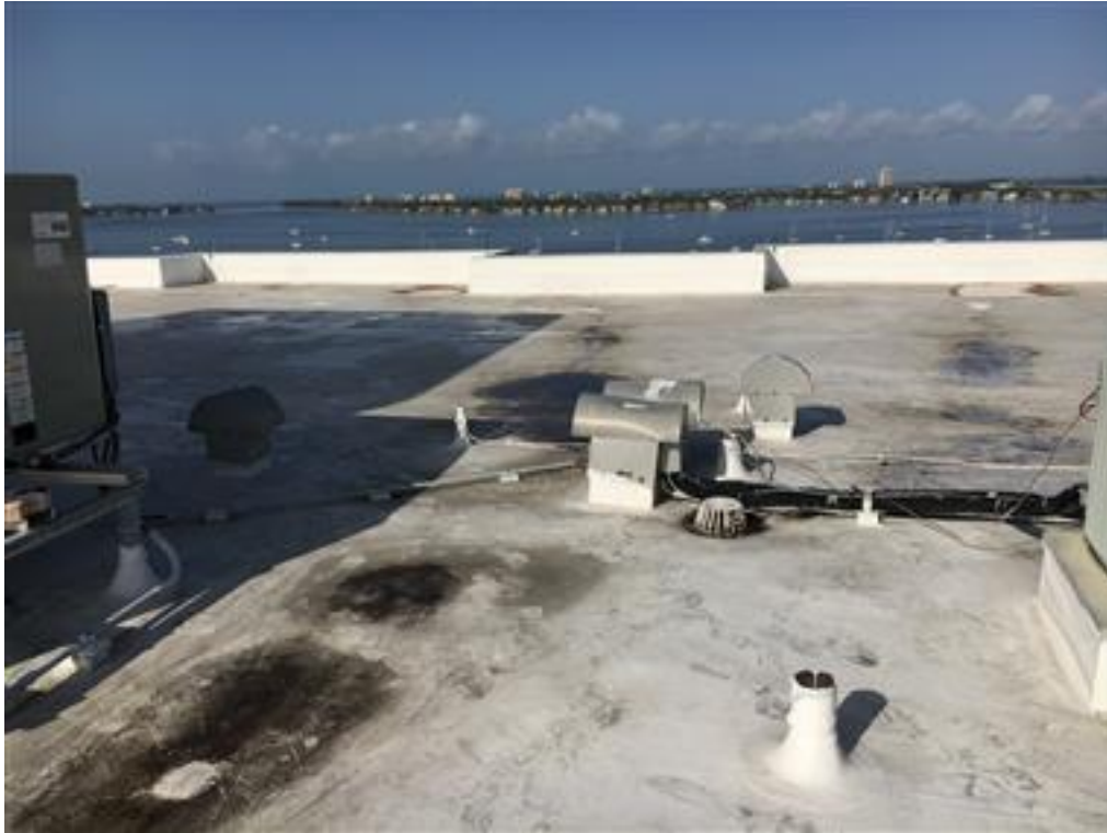
Photo 15-General view, typical vents, ponding
