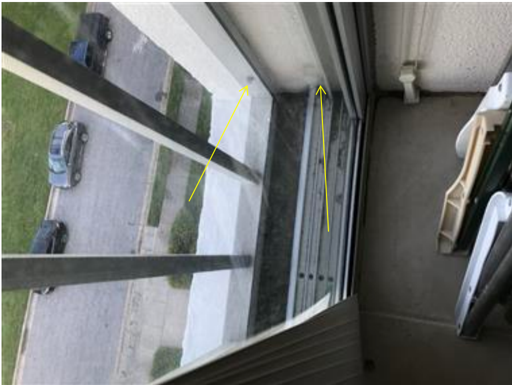
Photo 86-902- water damage at wall
