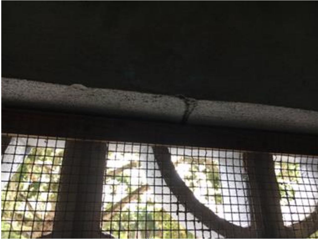
Photo 37-3 RD FLOOR- CRACK
