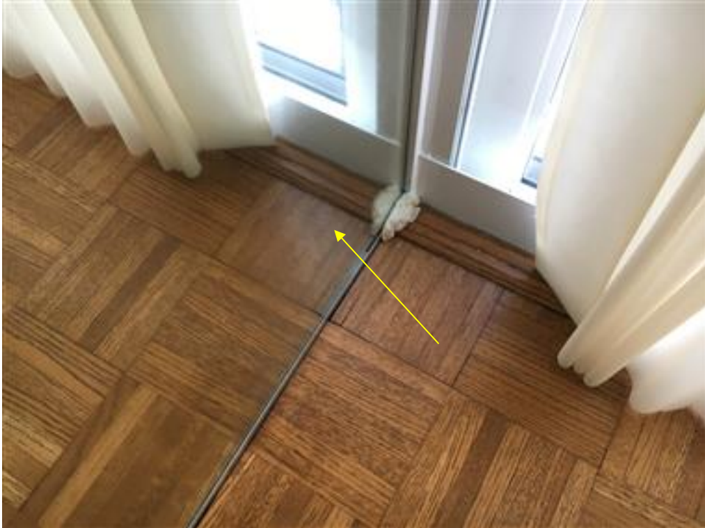
Photo 43-Unit 1201, tissues used to absorb water intrusion at SGD, typical
