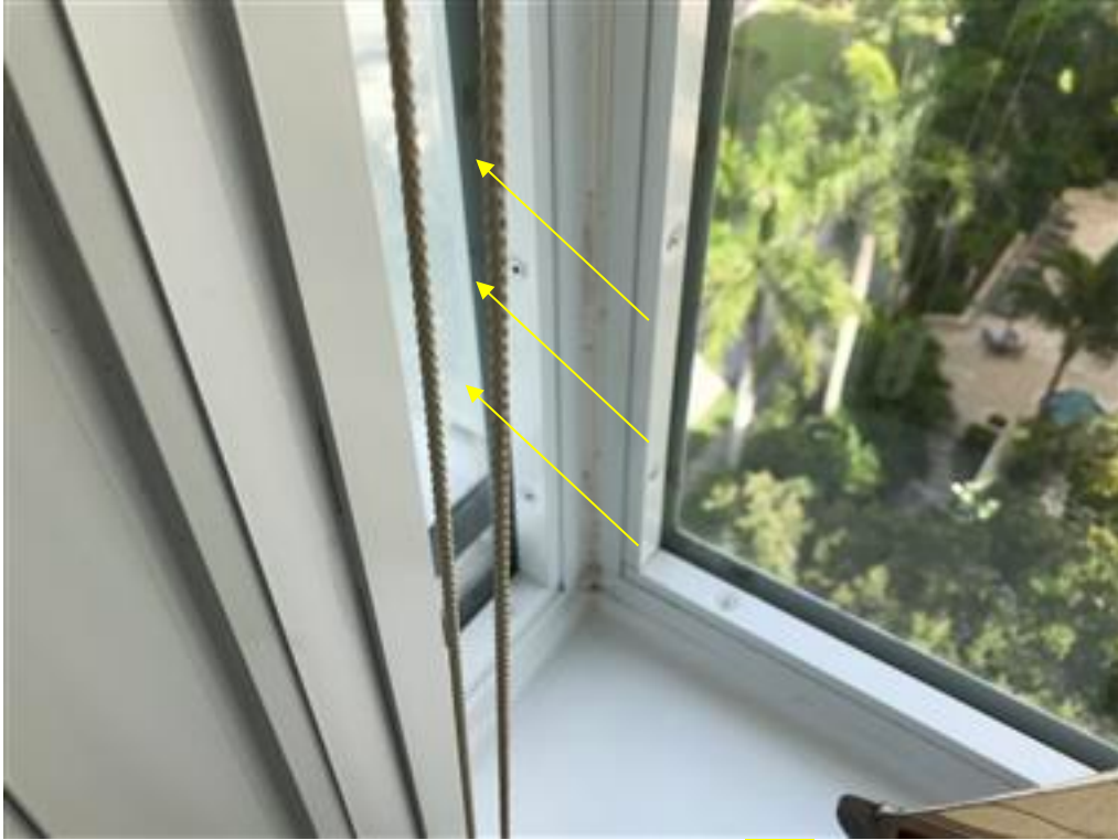
Photo 55-Unit 1101, joint sealant issue
