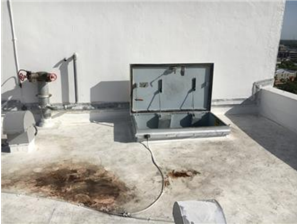
Photo 23-Roof access hatch, average condition, ponding
