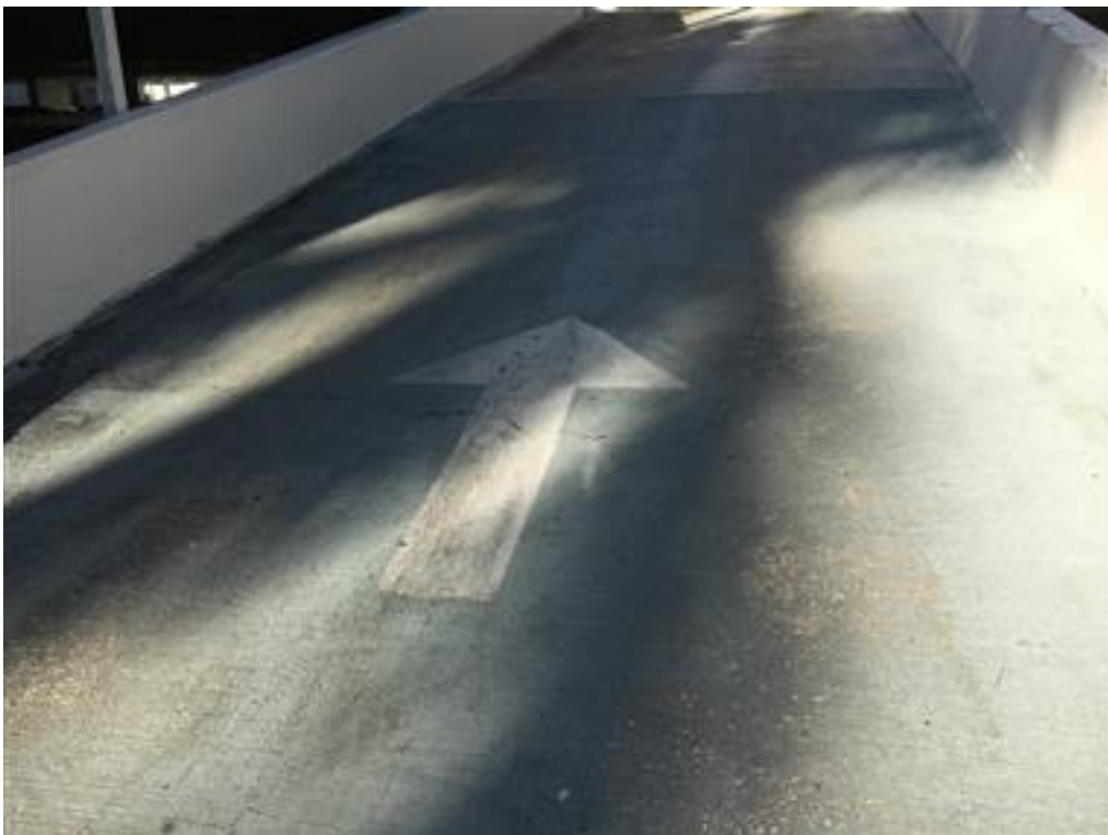
Photo 12-ENTRANCE RAMP- TYPICAL CRACKS
