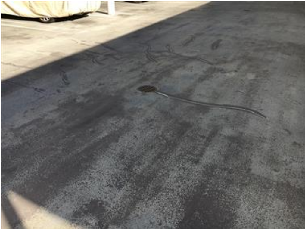
Photo 20- UPPER LEVEL-TYPICAL CRACKS
