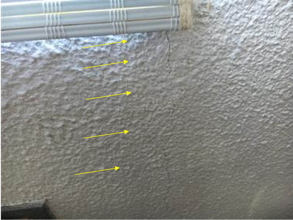
Photo 124-Unit 504, hairline crack at window sill, typical
