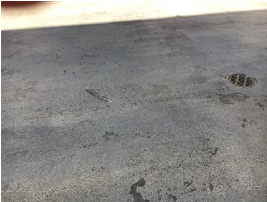
Photo 22- UPPER LEVEL-TYPICAL CRACKS
