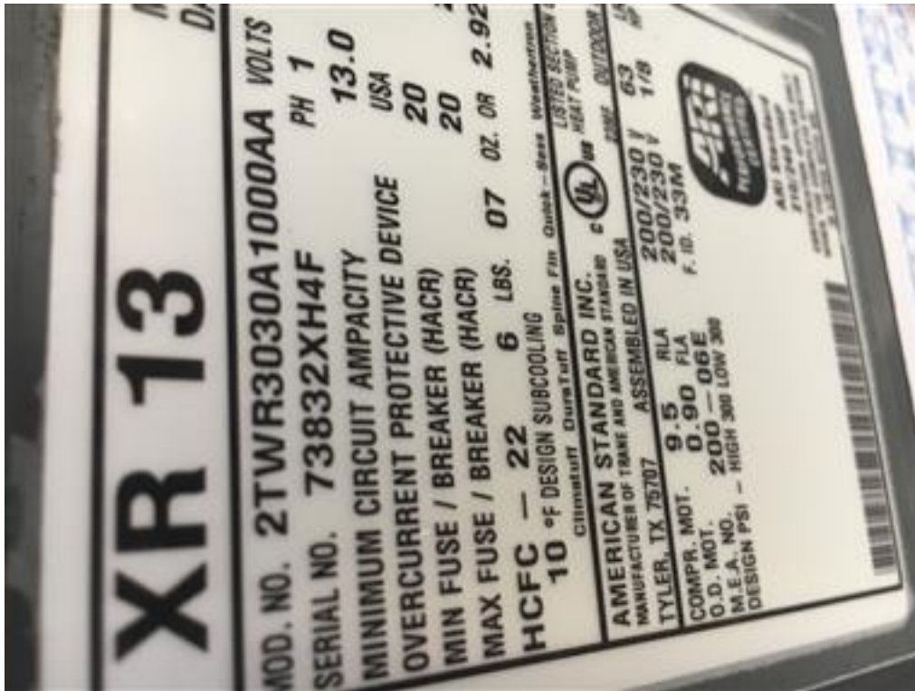
Photo 51-Kitchen AC condenser, good condition
