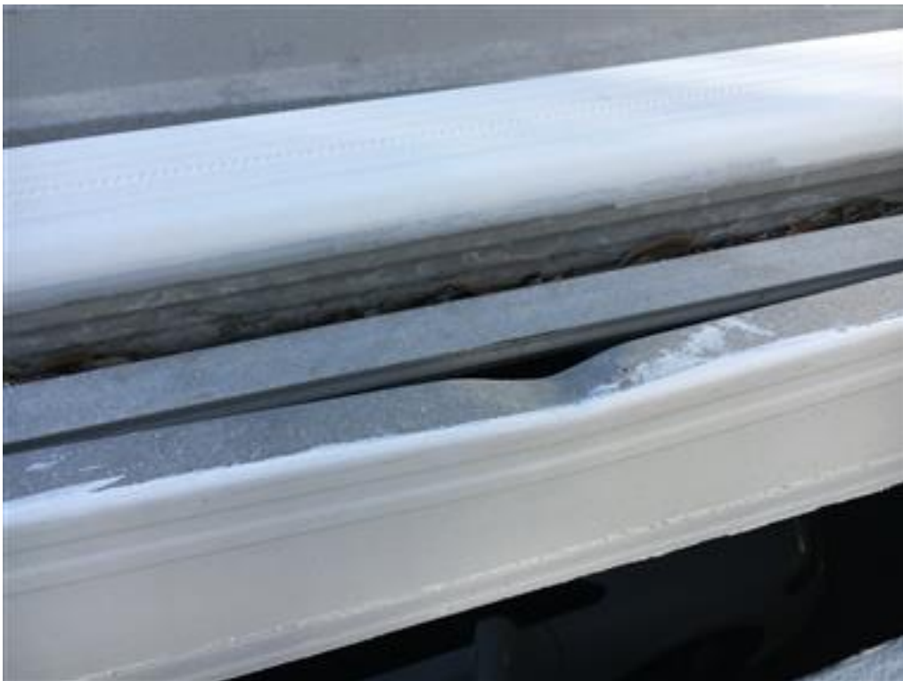
Photo 24-DENT AT ENTRANCE RAMP CARPORT ROOF
