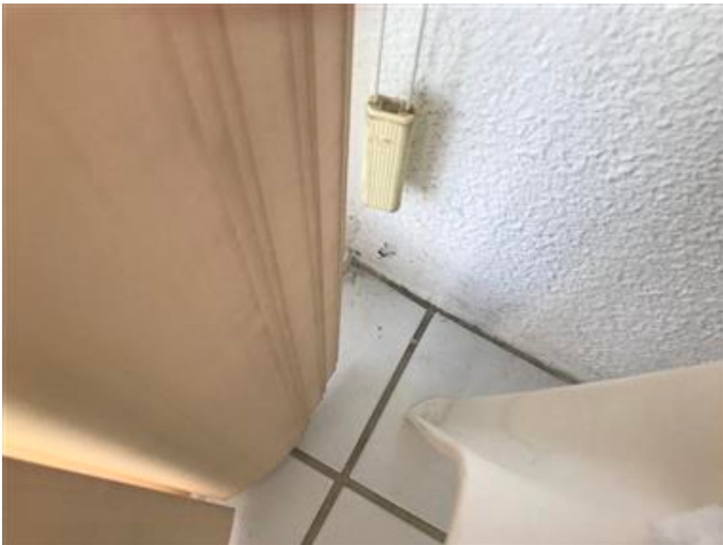
Photo 80-Unit 904, blistering paint due to water infiltration
