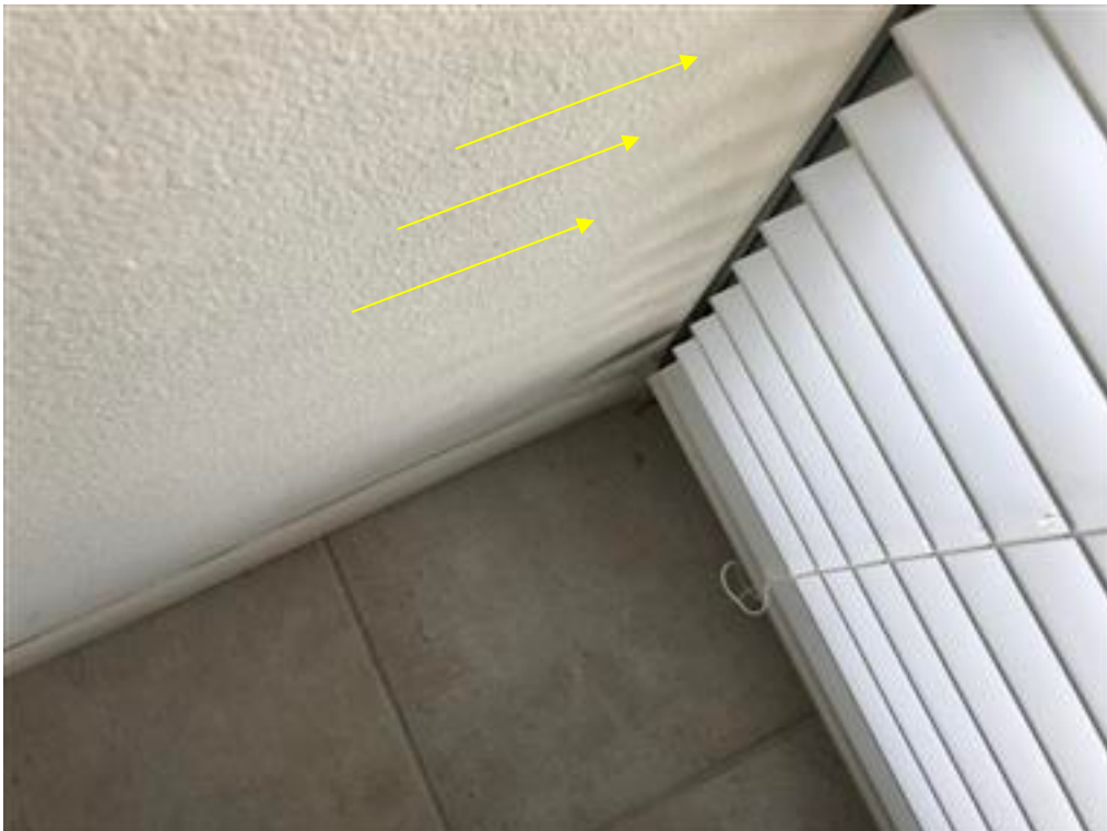
Photo 70-Unit 1002, crack in drywall at SGD
