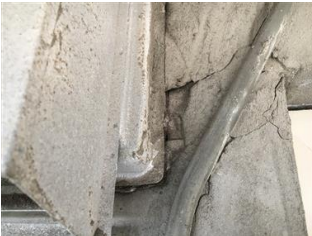
Photo 13-10 th FLOOR – CRACKS AT DOOR
