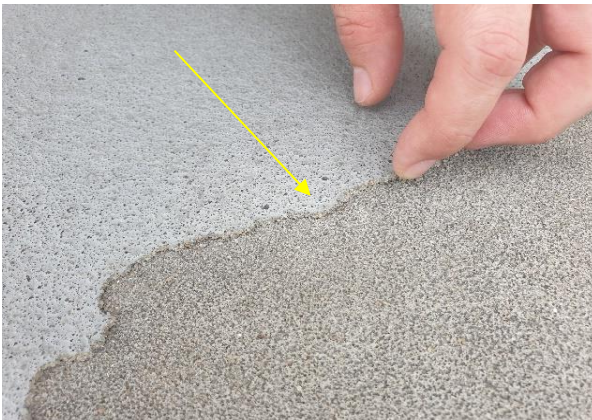
Photo 5: Bond failure between base and topcoat
