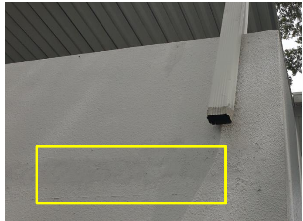
Photo 4: Previous concrete repair to the exterior of the parking garage
