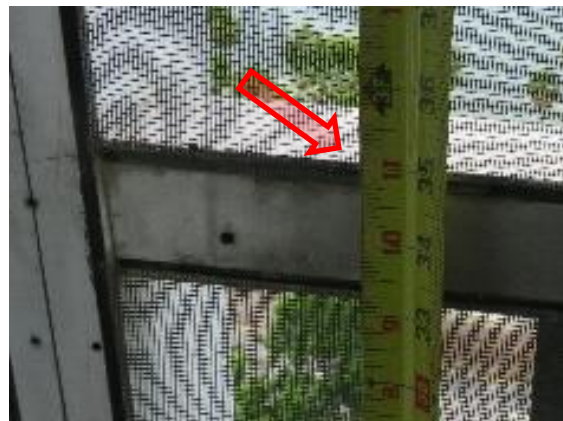
Photo 11: Guard rail below code required height
