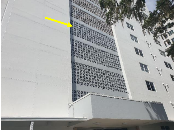
Photo 6: Overall Photo of Exterior Showing Damaged Stucco
