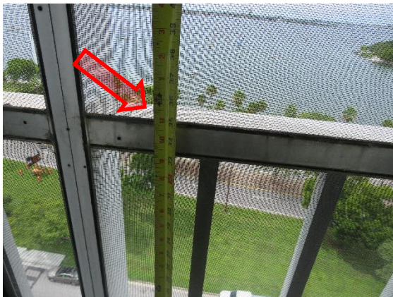
Photo 10: Guard rail below code required height.
