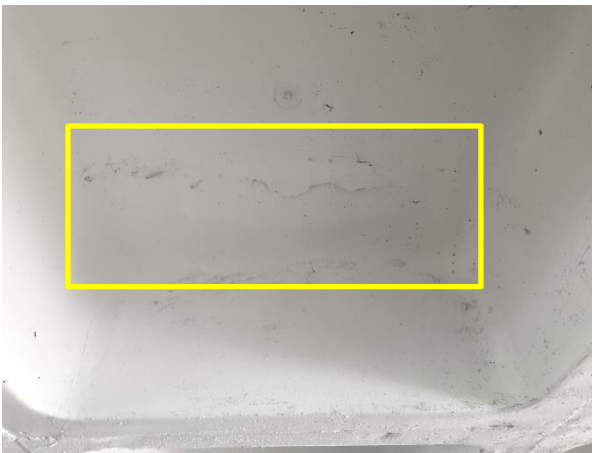
Photo 3: Peeling paint between the slab ribs
