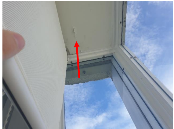
Water Damage at Interior Drywall
