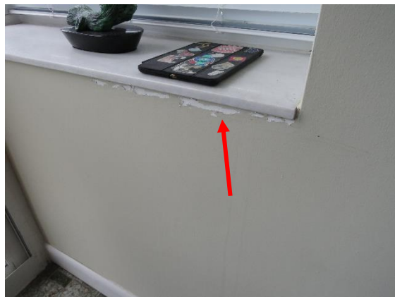
Peeling Paint at Enclosed Balcony
