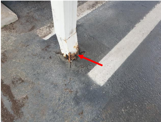
Damaged Steel Canopy Support
