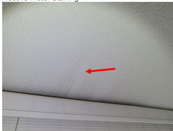
Inactive Water Staining
