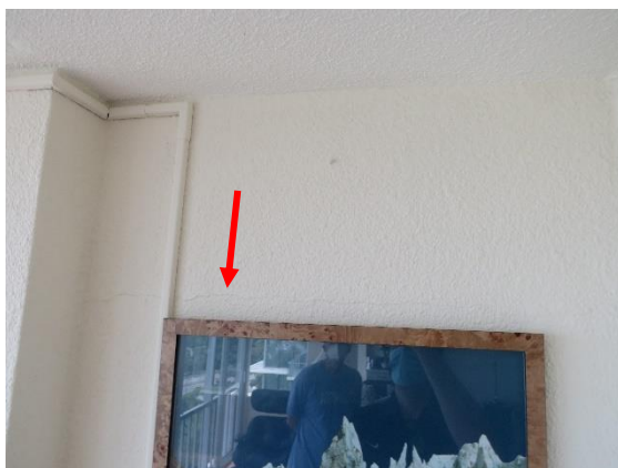
Cracking at Interior Drywall
