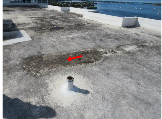
Ponding Water at Rooftop
