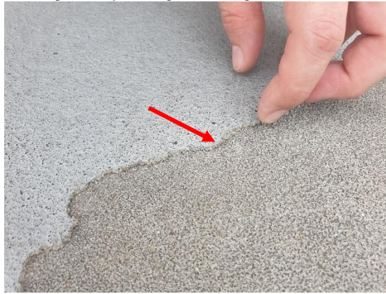
Additional Area of Bond Failure
