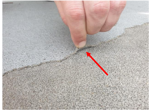
Bond Failure Between Base and Topcoat
