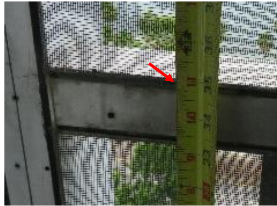
Guardrail Below Code Required Height
