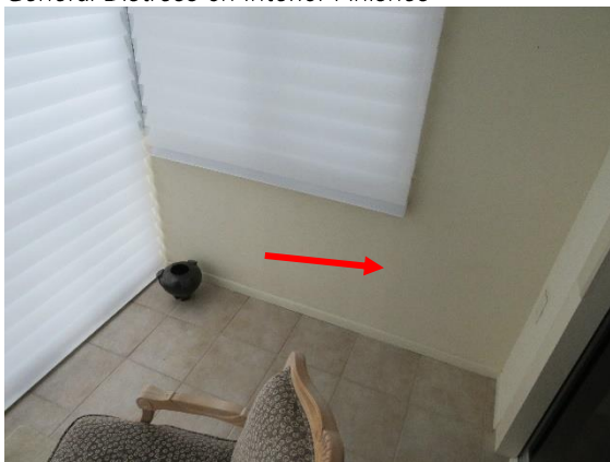
Inactive Water Staining
