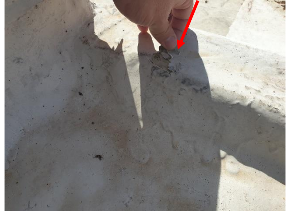
Tear in roof coating
