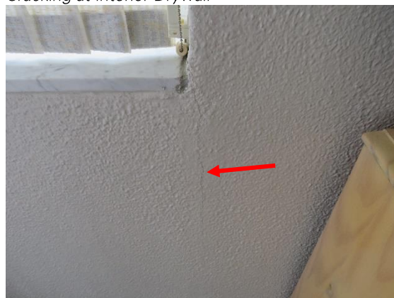
Cracking at Interior Drywall
