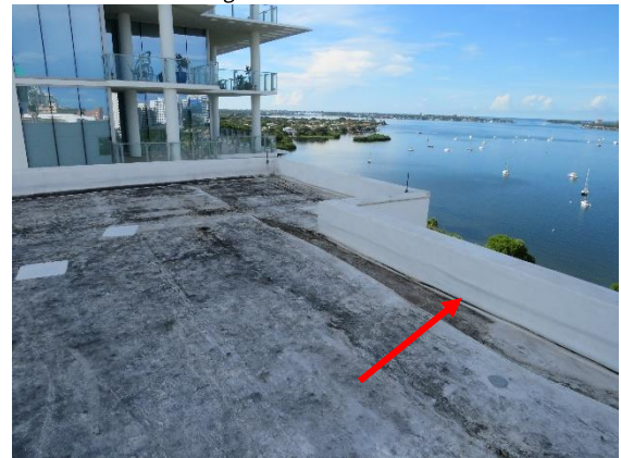
Wrinkling of Membrane at Parapet
