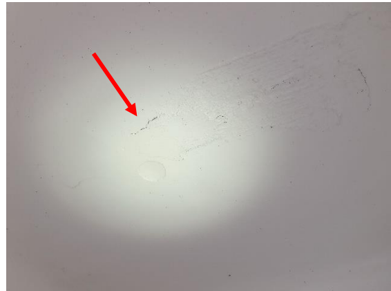
Concrete Spalling at Underside of Slab
