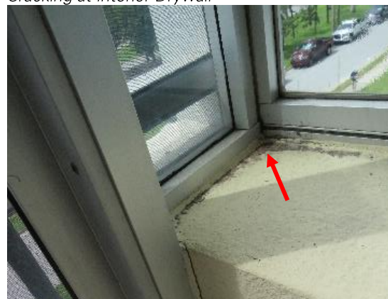
Cracking at Interior Drywall
