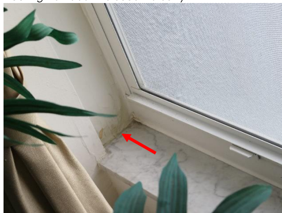
Inactive Water Staining
