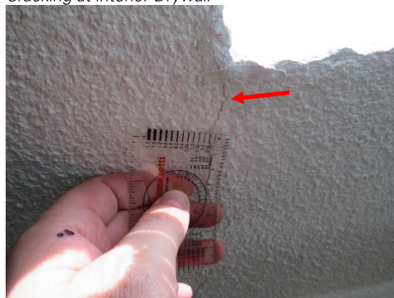
Cracking at Interior Drywall
