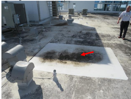
Ponding Water at Rooftop
