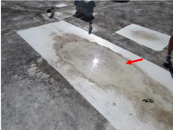
Ponding Water at Rooftop
