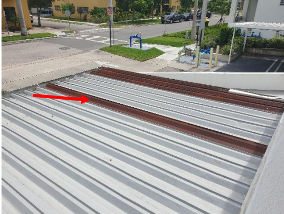
Corroded Metal Deck
