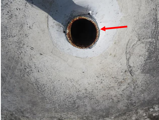
Hole in Penetration Screen Cover
