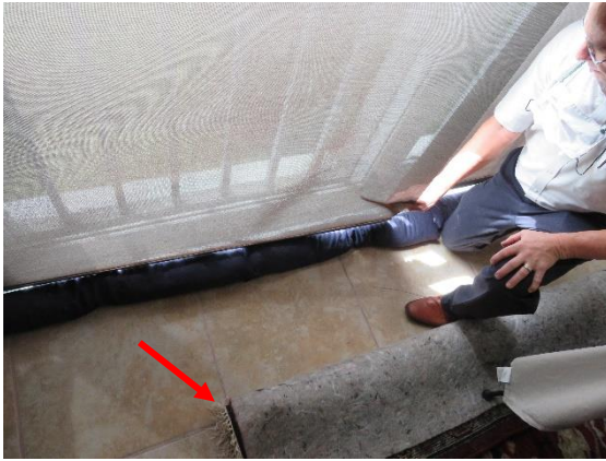
Cracked and Debonded Tile
