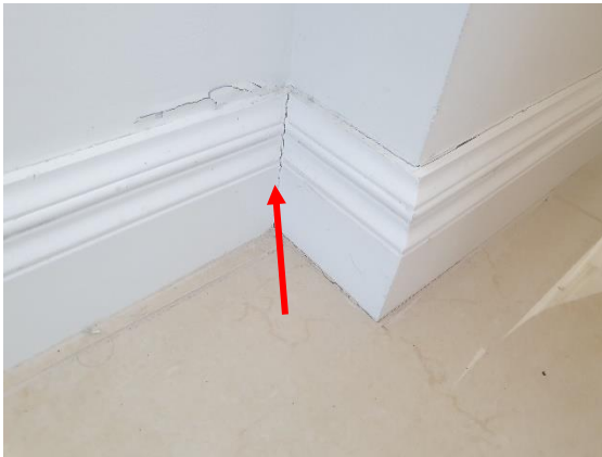
Cracking at Interior Drywall and Baseboards
