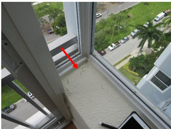
Blistering Paint at Enclosed Balcony
