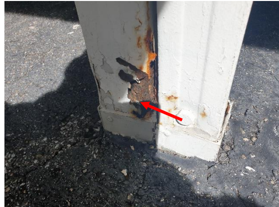
Corrosion at Canopy Support
