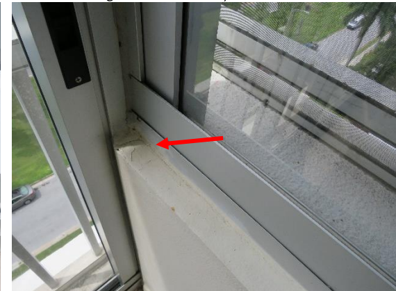
Blistering Paint at Enclosed Balcony
