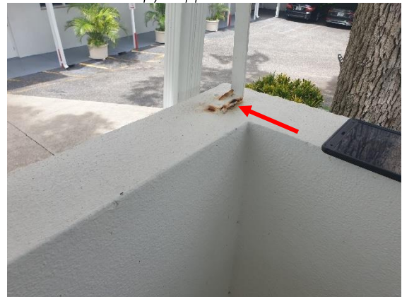
Corrosion at Canopy Tie Down Strap
