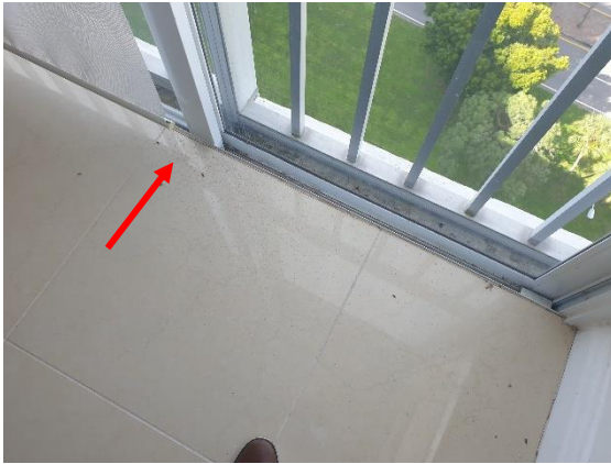
Termites Present in Unit
