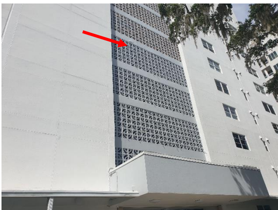
Overall Photo of Exterior Showing Damaged Stucco
