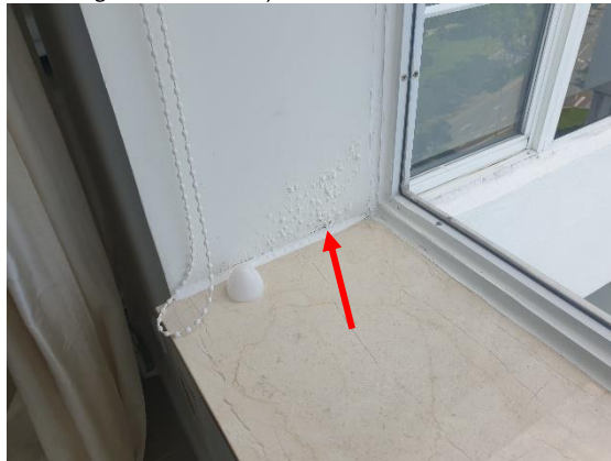
Water Damage of Interior Drywall
