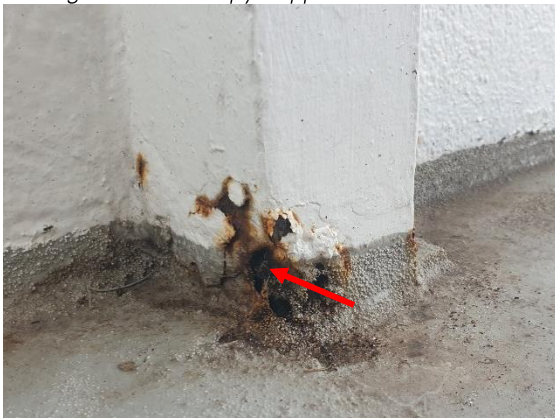
Corrosion at Canopy Support, Voids in Waterproofing
