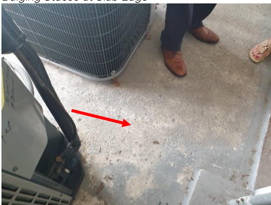
AC Condenser Area Slab Condition
