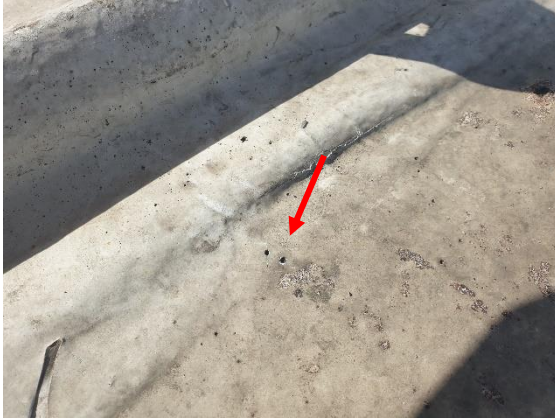
Voids and tear in roof coating
