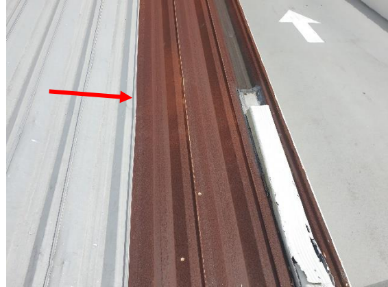
Corroded Metal Deck
