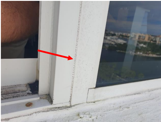
Failing Metal to Metal Sealant
