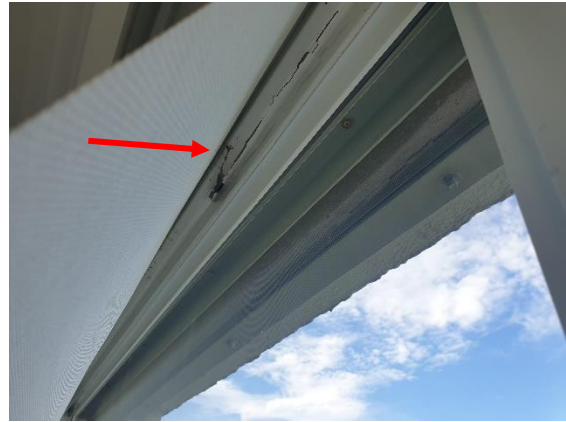
Wood Frame Showing Evidence of Termites
