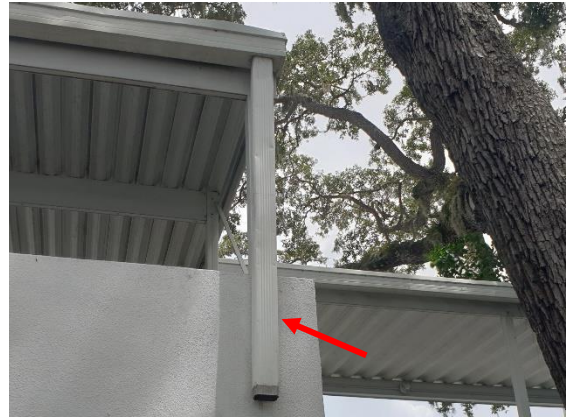
Corrosion at Canopy Support
