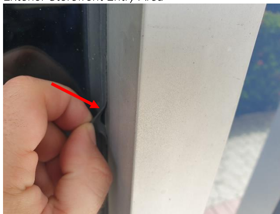
Failing Sealant at Storefront
