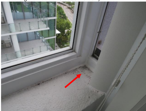
General Distress on Interior Finishes
