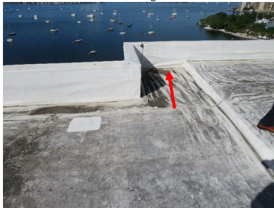
Wrinkling of Roof Membrane
