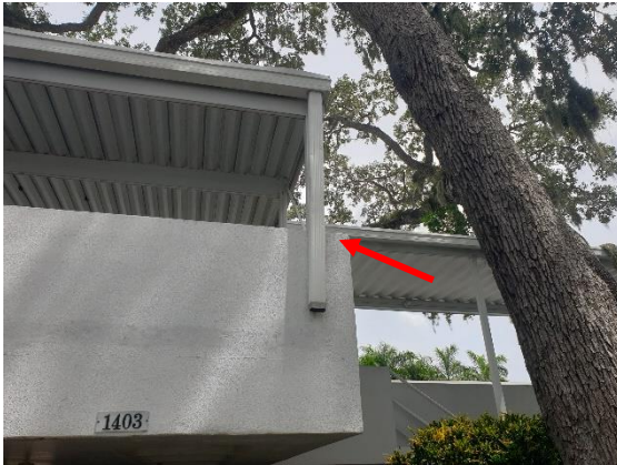
Damaged Steel Canopy Support
