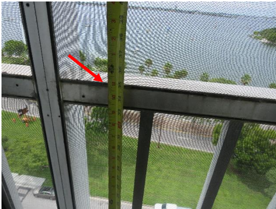
Guardrail Below Code Required Height
