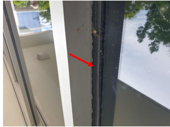
Failing Sealant at Storefront
