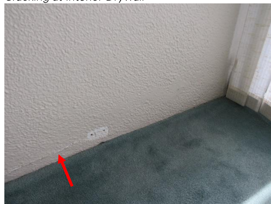
Cracking at Interior Drywall
