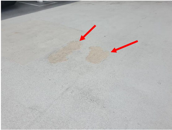
Missing Waterproofing at Parking Slab
