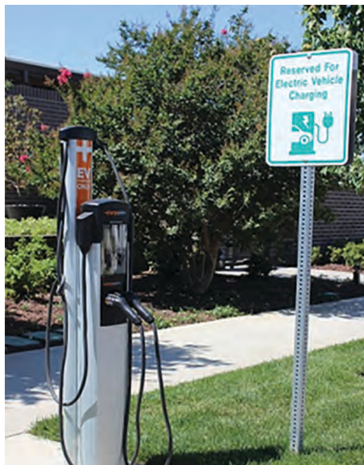
FIGURE 2 State Housing Law Program staff photo: electric vehicle charging station at multifamily residential complex.
