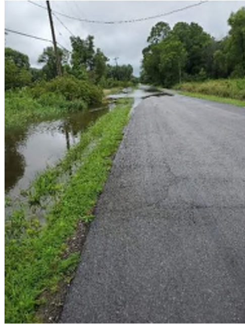
Photo 2.2 – Mantua Center Road Overtopped with Flood Waters
