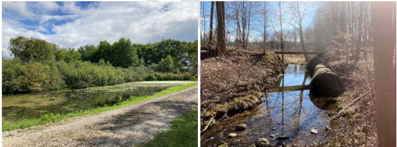
Figure 6. Poned area upstream of driveway embankment (left) and blown out culvert at old railroad line crossing (right)
