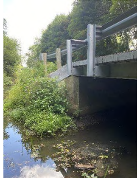
Figure 6 - Flow Sensor on Mantua Center Road Bridge
