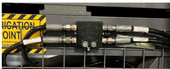
Figure 12: Remote Grease Lines
