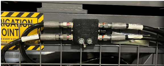
Figure 13: Remote Grease Lines
