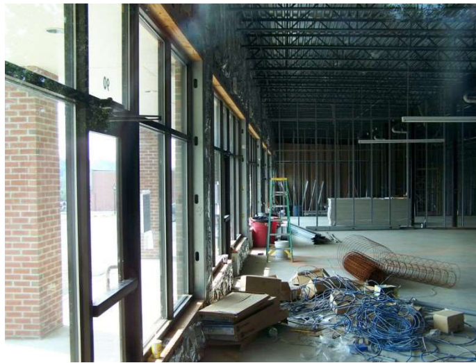
Figure 8. Lack of fire stopping between occupancies.
