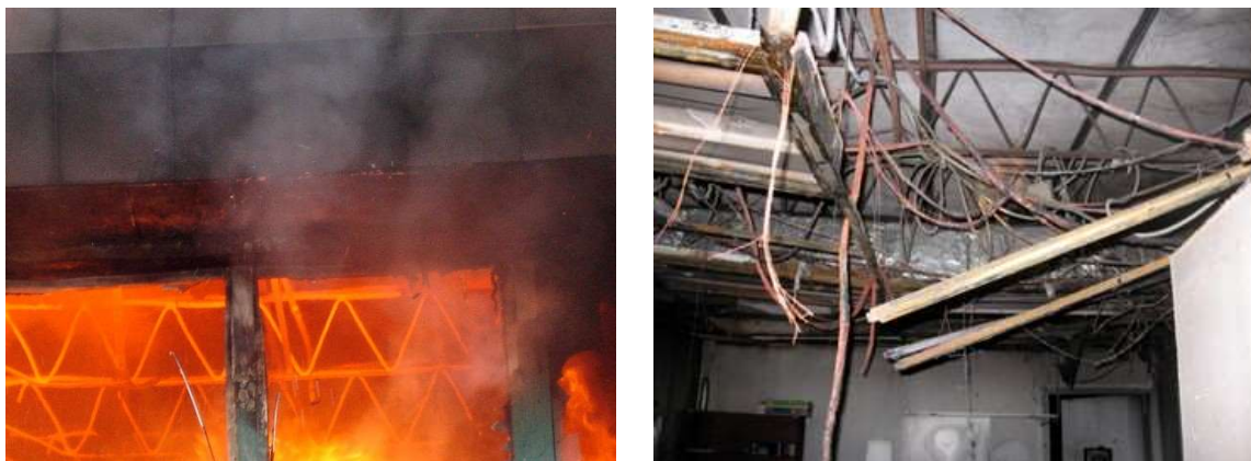
Figure 22. Steel bar joists. Beginning to fail in high temperatures (left) and frozen in place once cooled (right).
