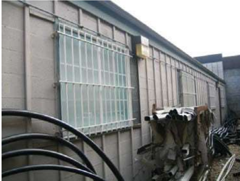
Figure 1. Rear windows secured with metal bars.
