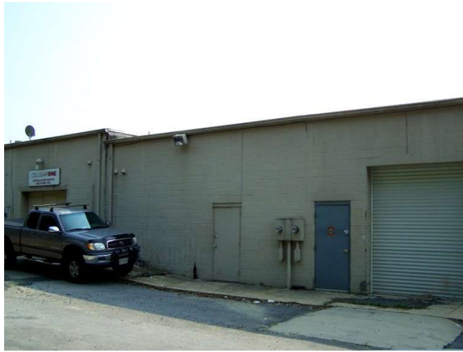
Figure 4. Difficult-to-identifying individual occupancies in the rear.
