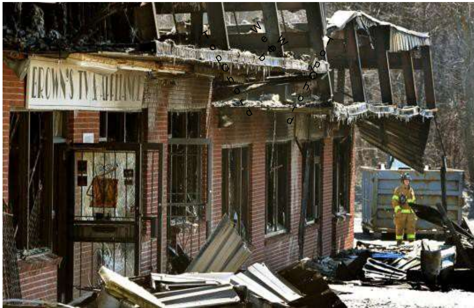
Figure 23. Fire spread to facade with collapse in a strip shopping center fire in Northborough, Massachusetts.
