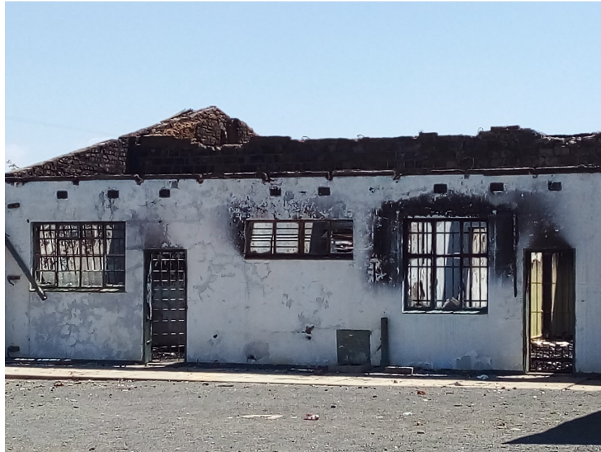
Fire-damaged property – future church and school.
