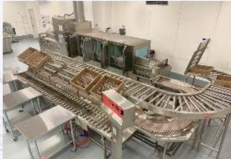
DISH ROOM CONVEYORS
