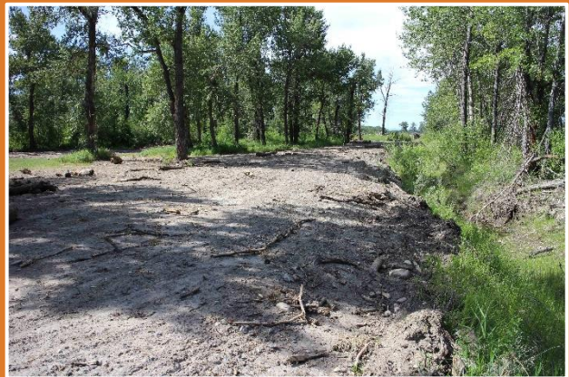
This area of bare ground has resulted from removal of a riverbank berm structure and initial reclamation of adjacent house footprints. Soil bioengineering bank stabilization, rough and loose soil surface treatment and riparian plantings should be considered as part of the restoration prescription for this site.
