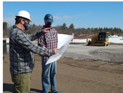
Owner Shaw Dwight, left, and Cultivation Manager Michael Tillman review blueprints for the new 12,500-square-foot Paul's Boutique cultivation and manufacturing facility under construction in the Enterprise Development District Zone of North Windham. PHOTO BY ED PIERCE
