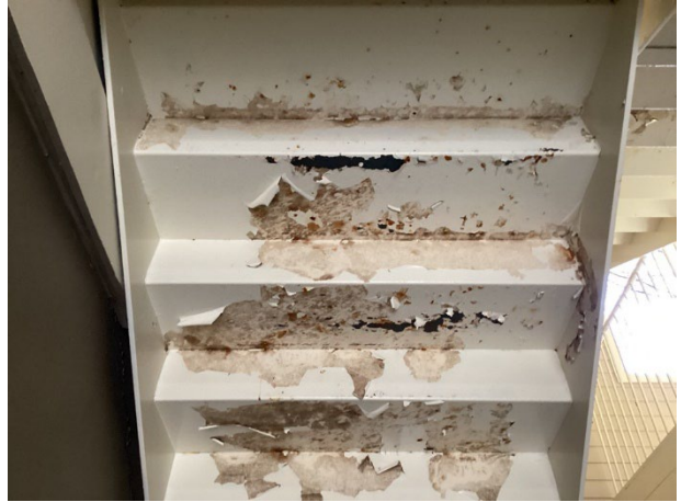
Corrosion at metal frame
