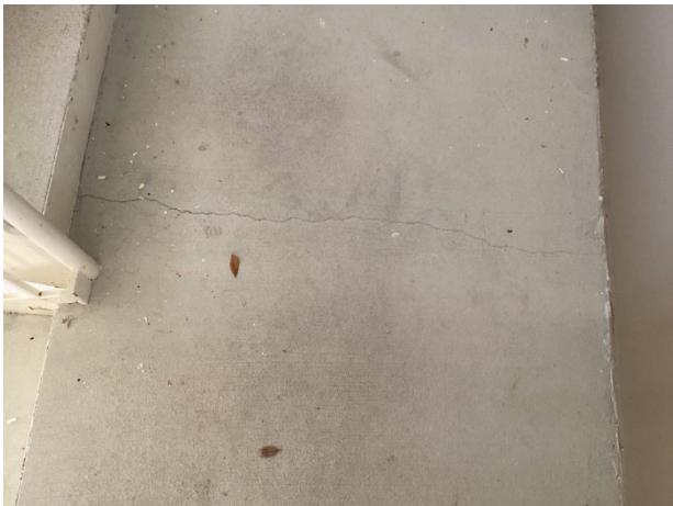
Concrete crack at landing
