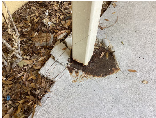
Rust and concrete damage at column base
