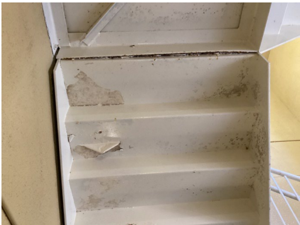
Metal frame damage
