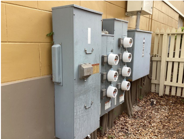
Electrical system components
