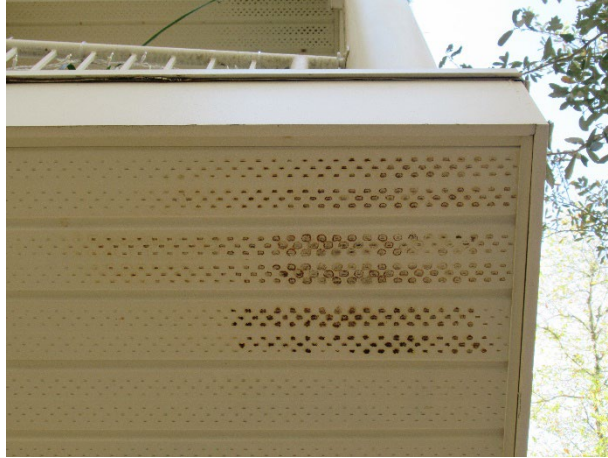
Stains indicative of previous water intrusion
