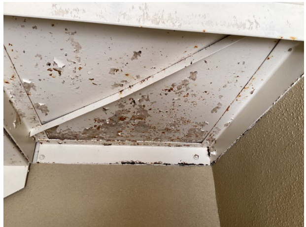
Corrosion at metal frame
