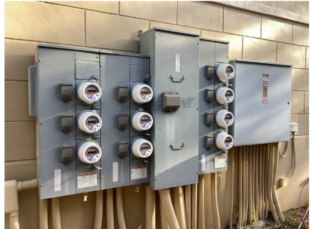
Electrical system components
