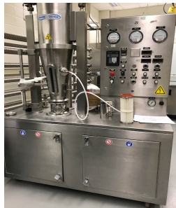
A spray dehydrator at Purdue University's Mock Sterile Food Production Lab. They host food manufacturing courses conducted by the FDA.
