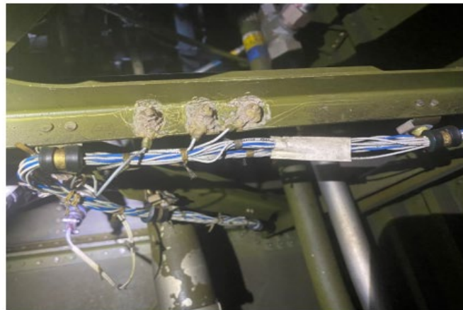
Figure 13 - Grounding Terminals Not Properly Bonded (Discrepancy #10)
