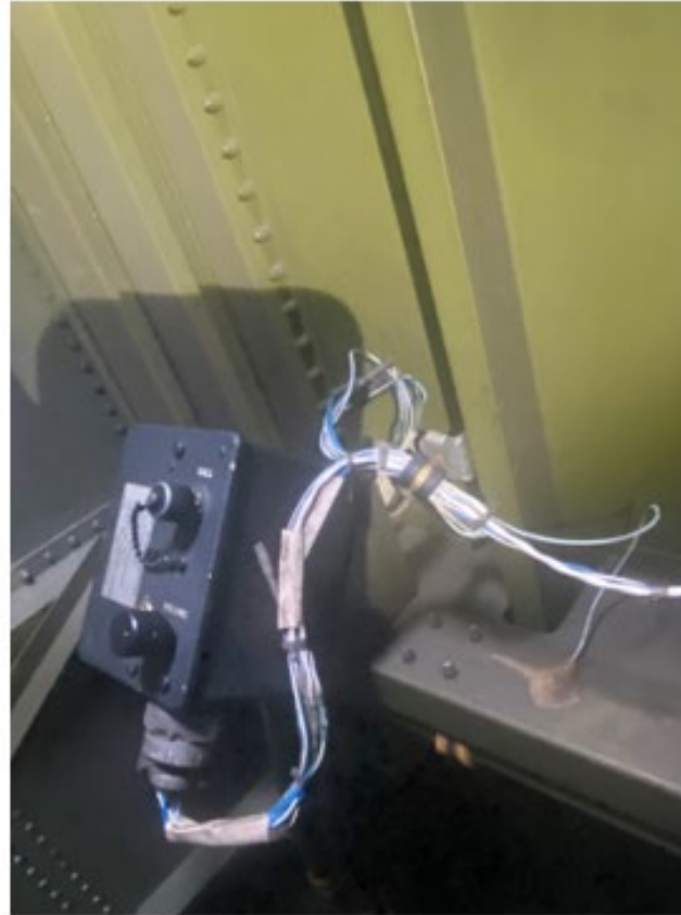
Figure 17 - Top Intercom Station Incorrect Splices and Slack (Discrepancy #14)
