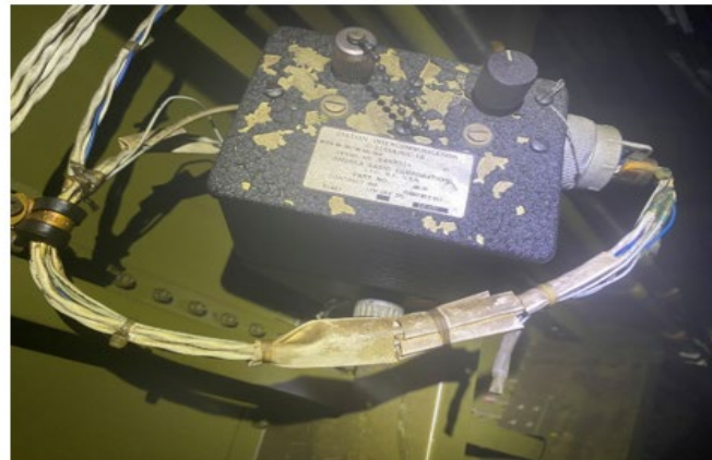
Figure 7 - Intercom Station Cannon Plug Cable Bend Radius (Discrepancy #4)
