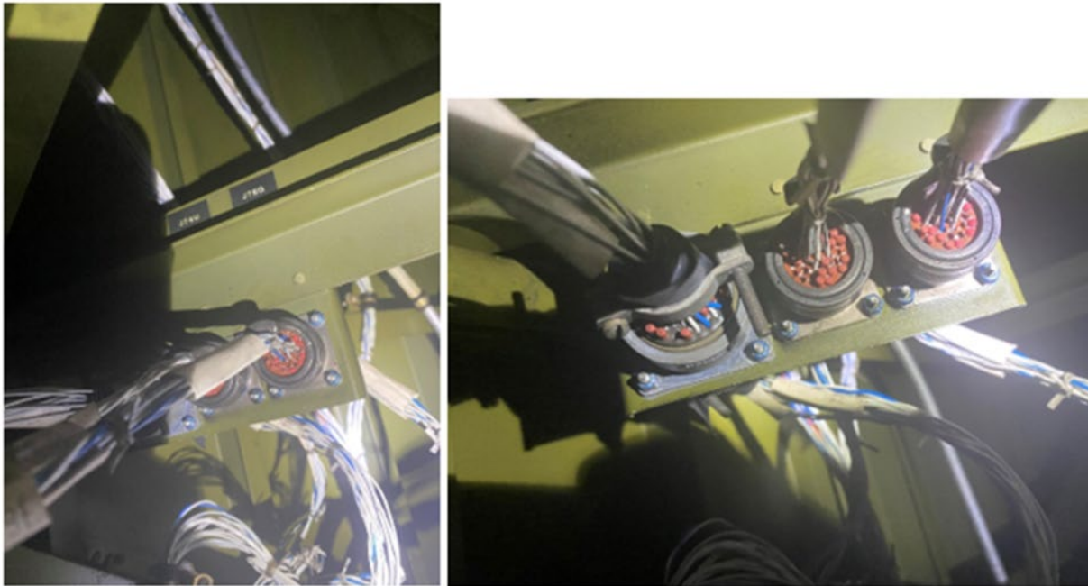
Figure 4 - J75G Cannon Plug Missing Pin Filler Inserts (Discrepancy #1)
