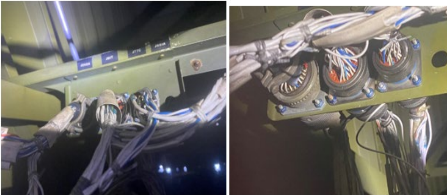
Figure 5 - J61T Cannon Plug Missing Pin Filler Inserts (Discrepancy #2)
