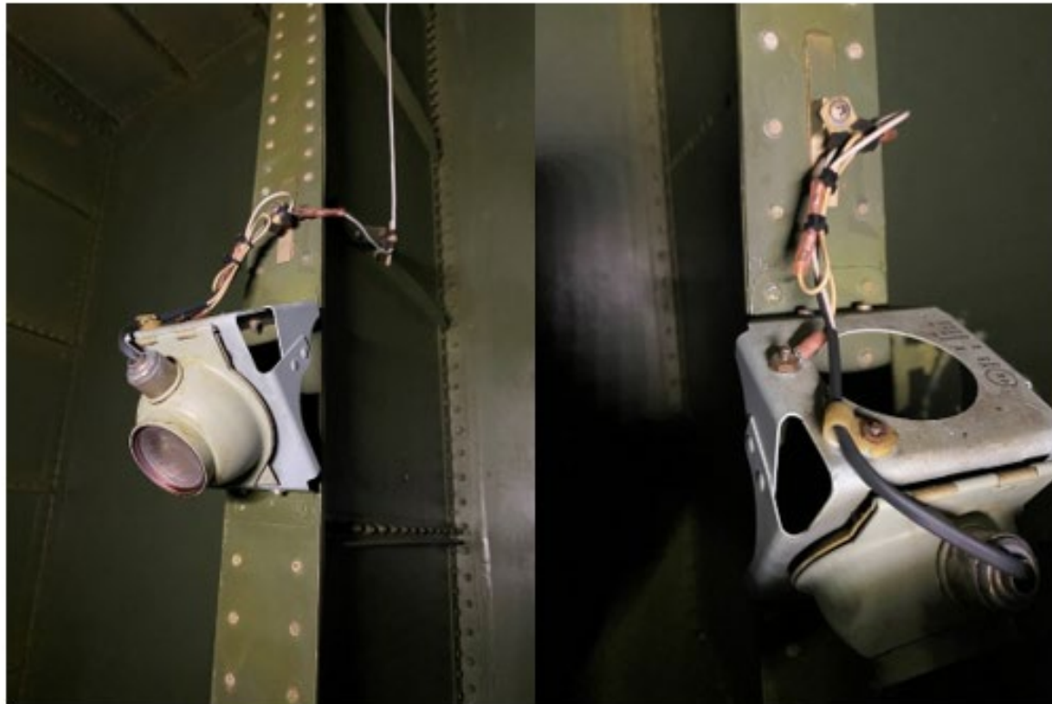
Figure 44 - Improper Cable Management (Discrepancy #41)
