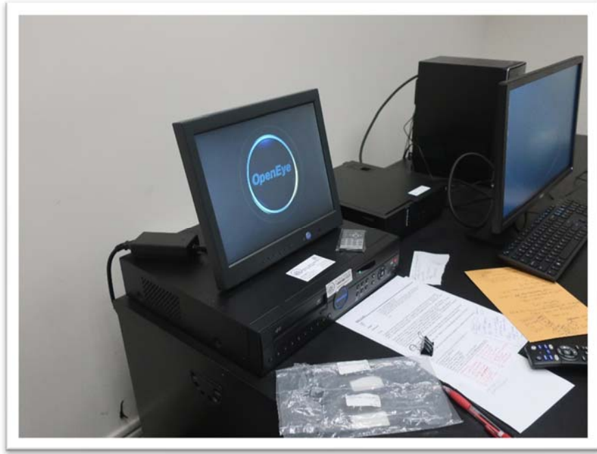
Photograph 17: Typical view of video security system
