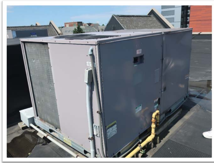
Photograph 7: Typical view of roof top unit
