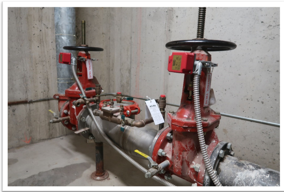
Photograph 27: Typical view of backflow preventer
