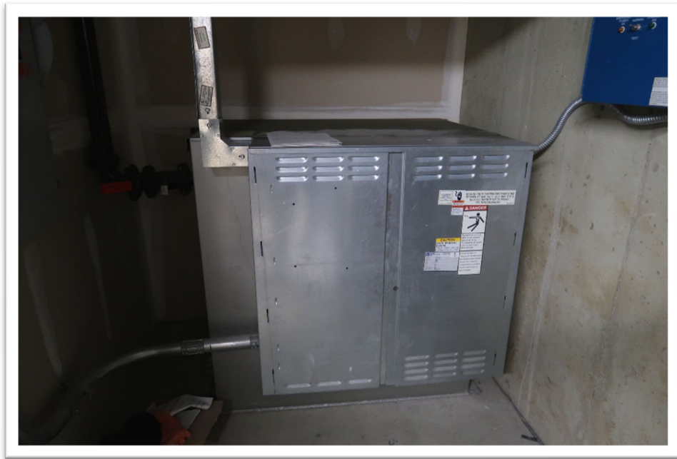
Photograph 23: Typical view of elevator hydraulic tank
