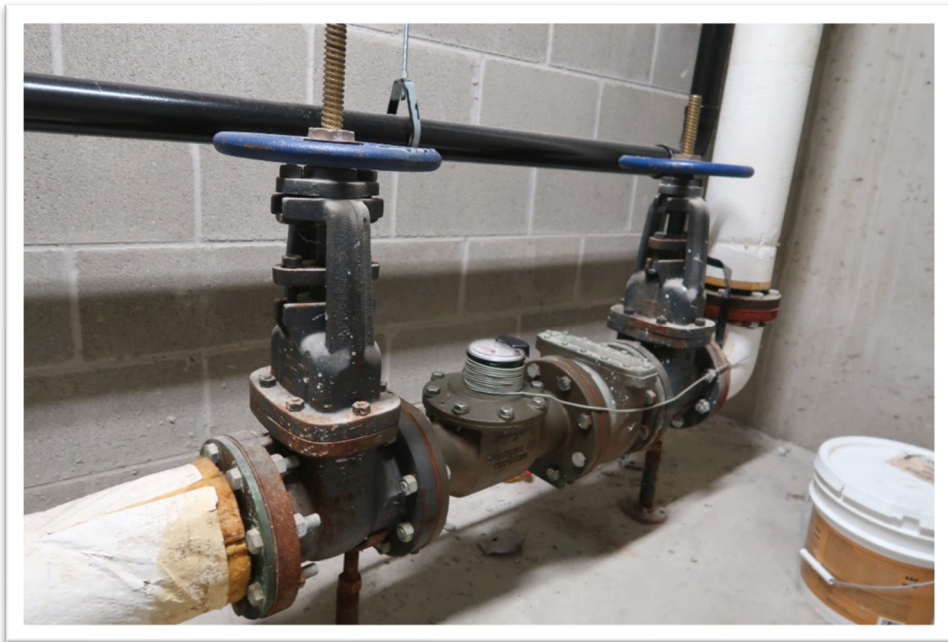
Photograph 28: Typical view of backflow preventer
