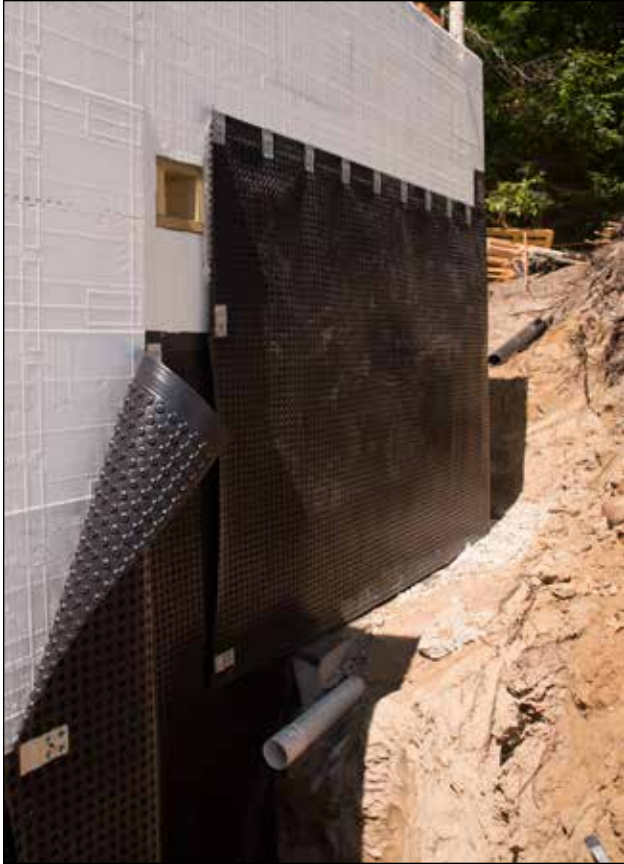
Waterproofing membrane and air gap membranes installed and mechanically attached above grade levels.
