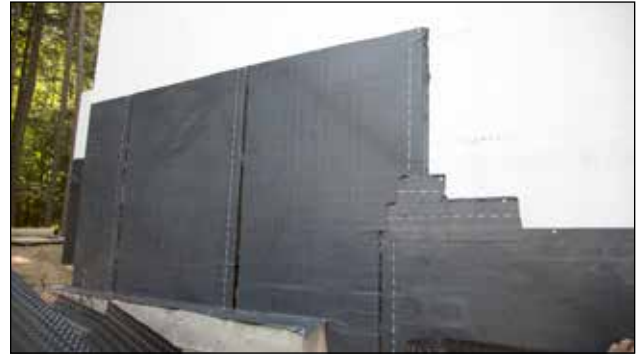
Adhesive waterproofing membrane installed. Note overlap on all seams and mechanical attachment at the top of the membrane.
