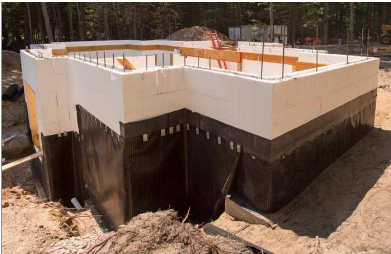
Typical walkout ICF basement using a waterproofing barrier and an air gap membrane installed as well as perimeter foundation drainage.
