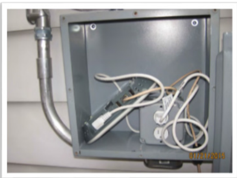
Photo D9: Equipment is not rated for location. In this case, a non-GFCI outlet for PV monitoring equipment is located in a wet location: NEC 110.3(B), 210.8(A)(3)
