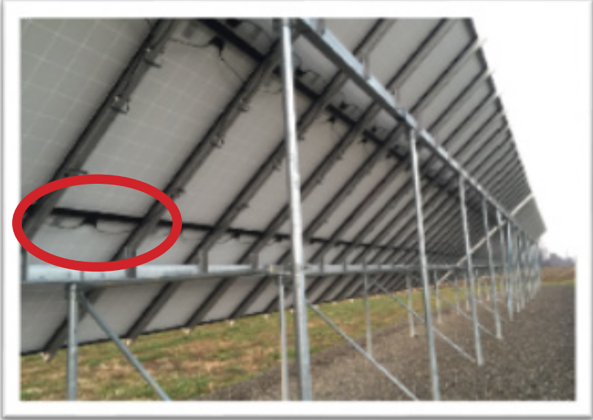
Photo D5 - Conductors over 30V not guarded, installed in raceway, or otherwise inaccessible: NEC 690.31(A)
