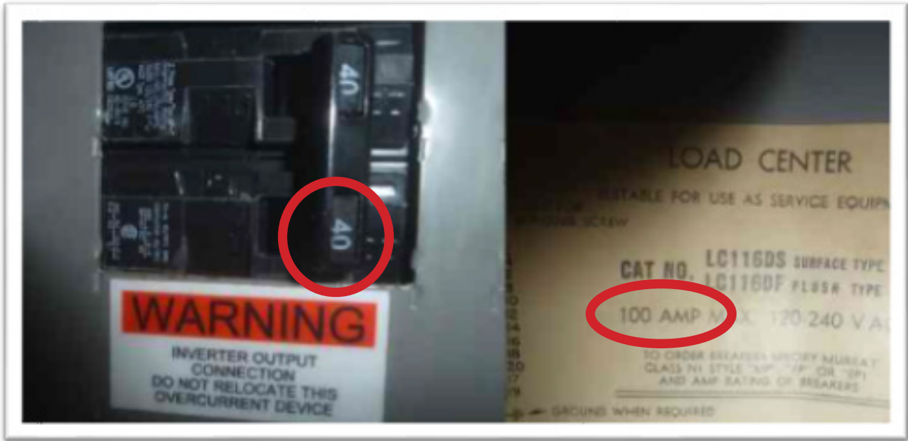
Photo D1: Main service panel overloaded per NEC 705(D)(2)(3)(b). (100 amp main circuit breaker + 40 amps of PV) ÷ 100 amp bus rating >120%.
