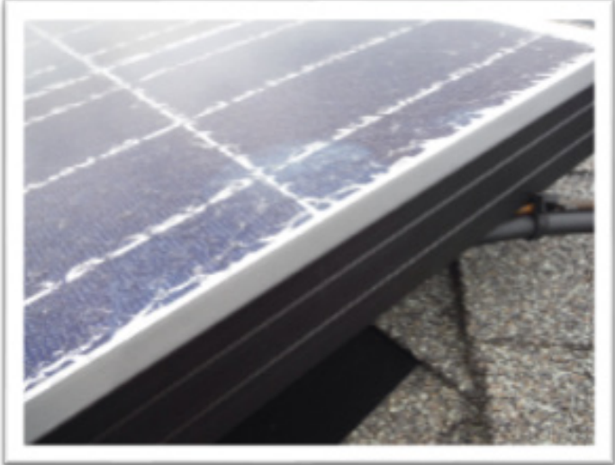
Photo D4: Equipment visibly damaged
