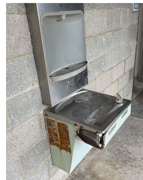
Old rusty water fountain at South Jetty Park
