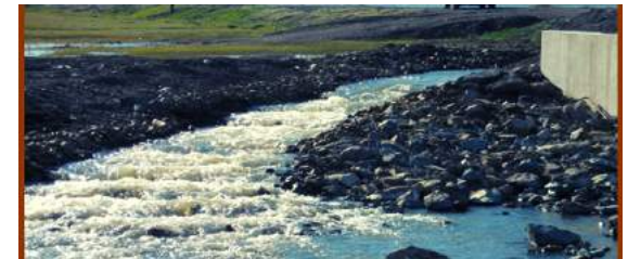
Bypass Channel allow fish to re-enter the stream below diversion during irrigation season when barriers are in place
