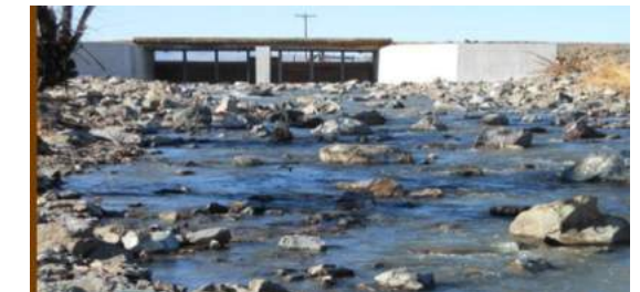
Rock Ramp constructed to increase stream elevation so fish can pass over concrete apron
