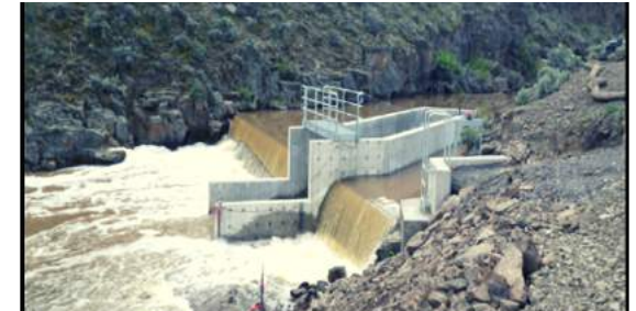
Cement cast technical fishway-ladder designed specifically for Warner sucker and Redband trout
