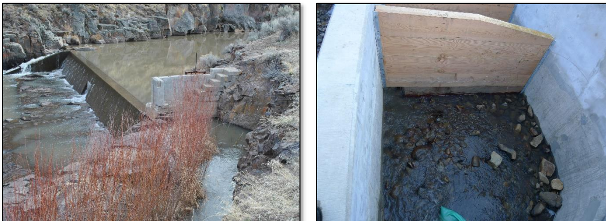
Figure 6-1. The existing Dyke diversion weir showing the weir, Denil fish ladder, and headwall with irrigation canal (left). The fish ladder completed in 2015, includes wooden weir walls with a 12-inch square orifice and streambed simulation material (right, photo during construction).
